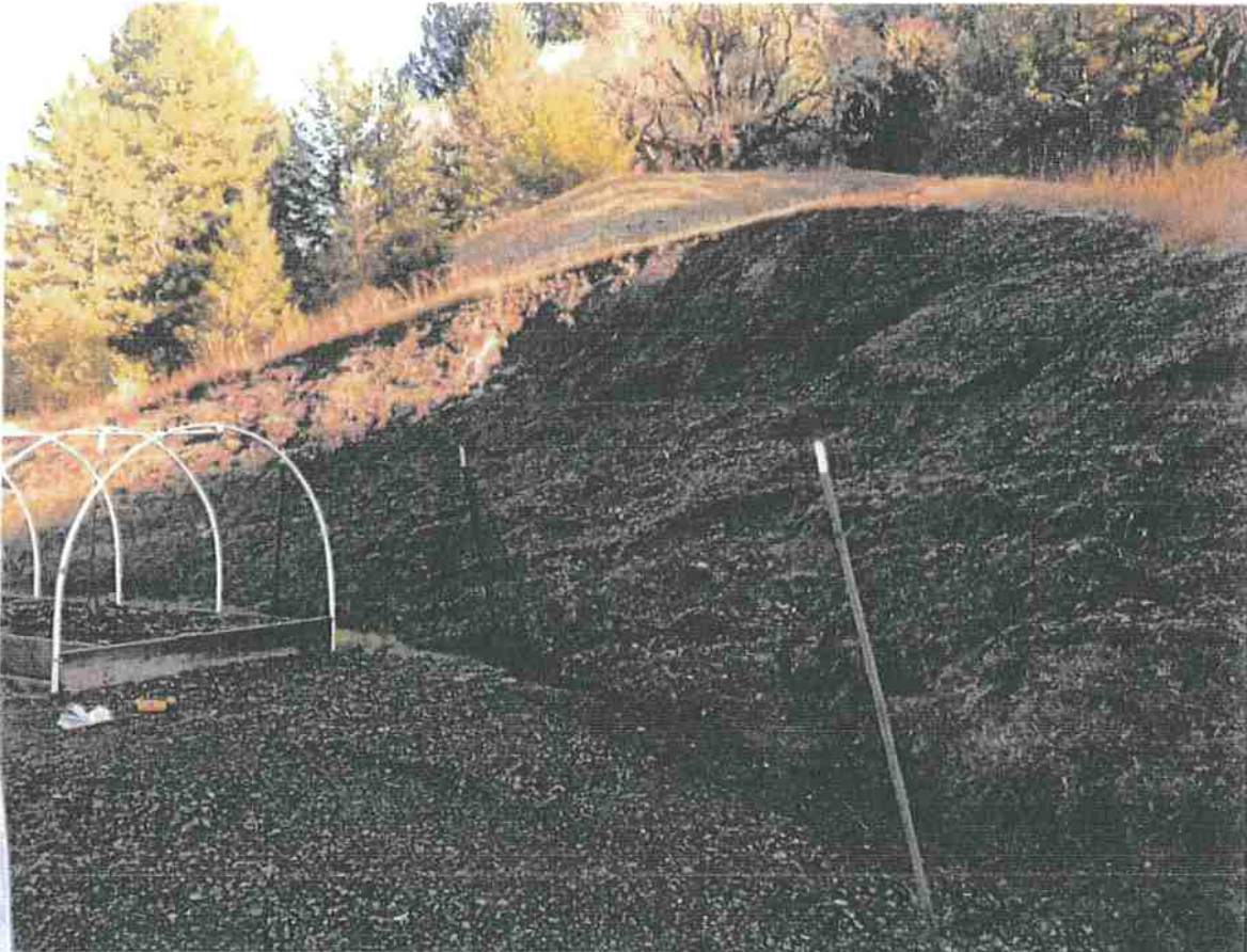
Photo #1: Erosion occurring on the cut bank at Map Point #5 (MP 5). The cut-bank will be reshaped to a slope no greater than 1.5/1. The slope will be seeded with native annual and perennial grasses. A rolled erosion control product will then be fastened over the slope. Photo Date: 11/27/2017.
