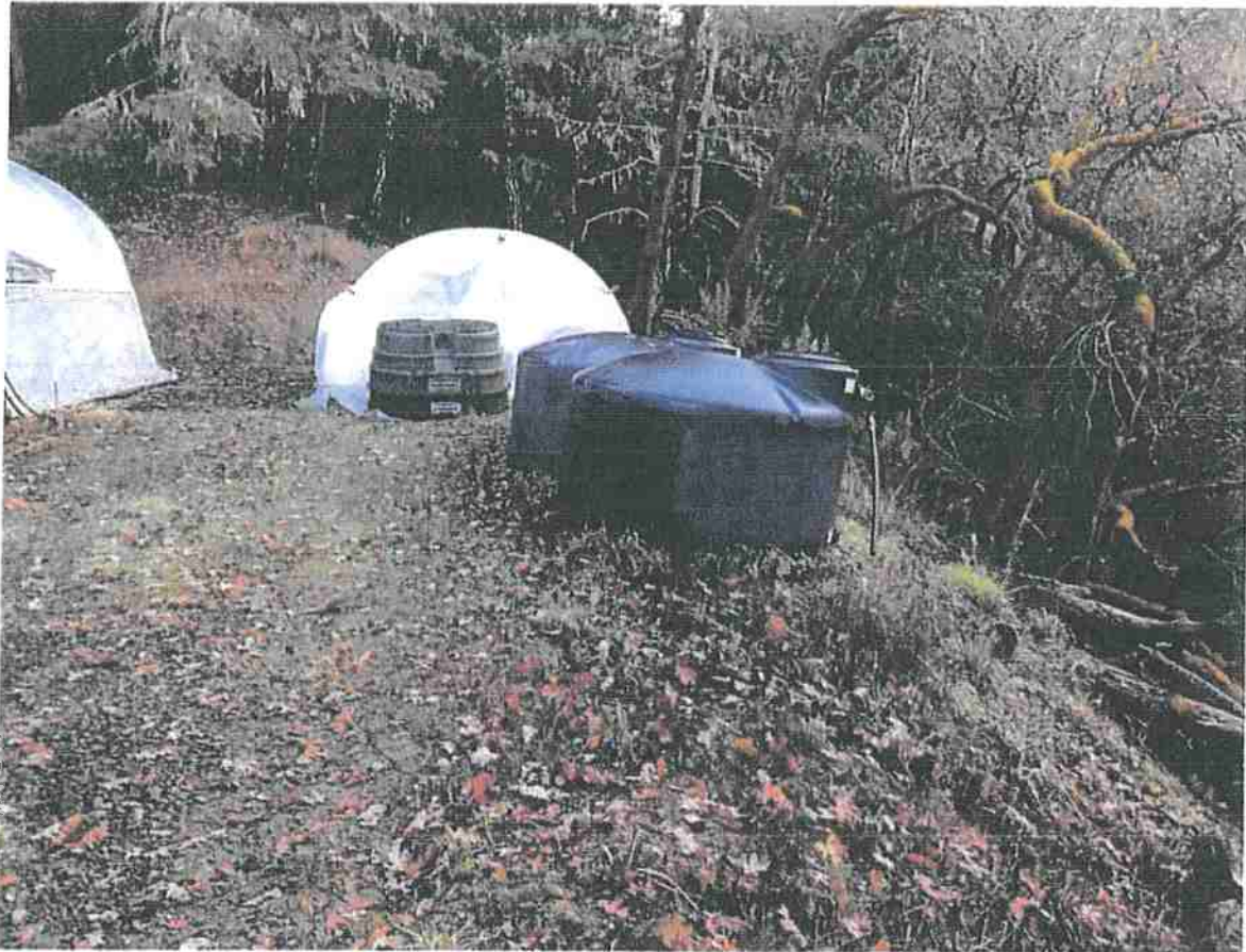
Photo #2: Water storage tanks that are inadequately installed within the riparian area of the adjacent Class II watercourse. These water storage tanks will be relocated to a location outside of all riparian buffer zones, and installed on flat stable ground. Photo Date: 11/27/2017.
