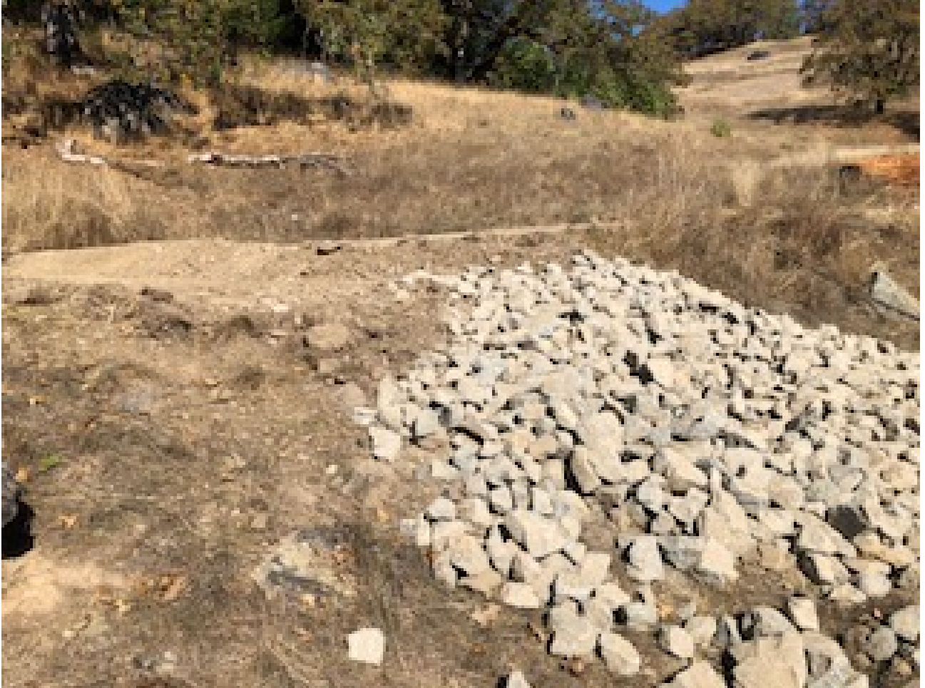
Figure 4: Close up of WB-2, the second waterbar east of the residence.
