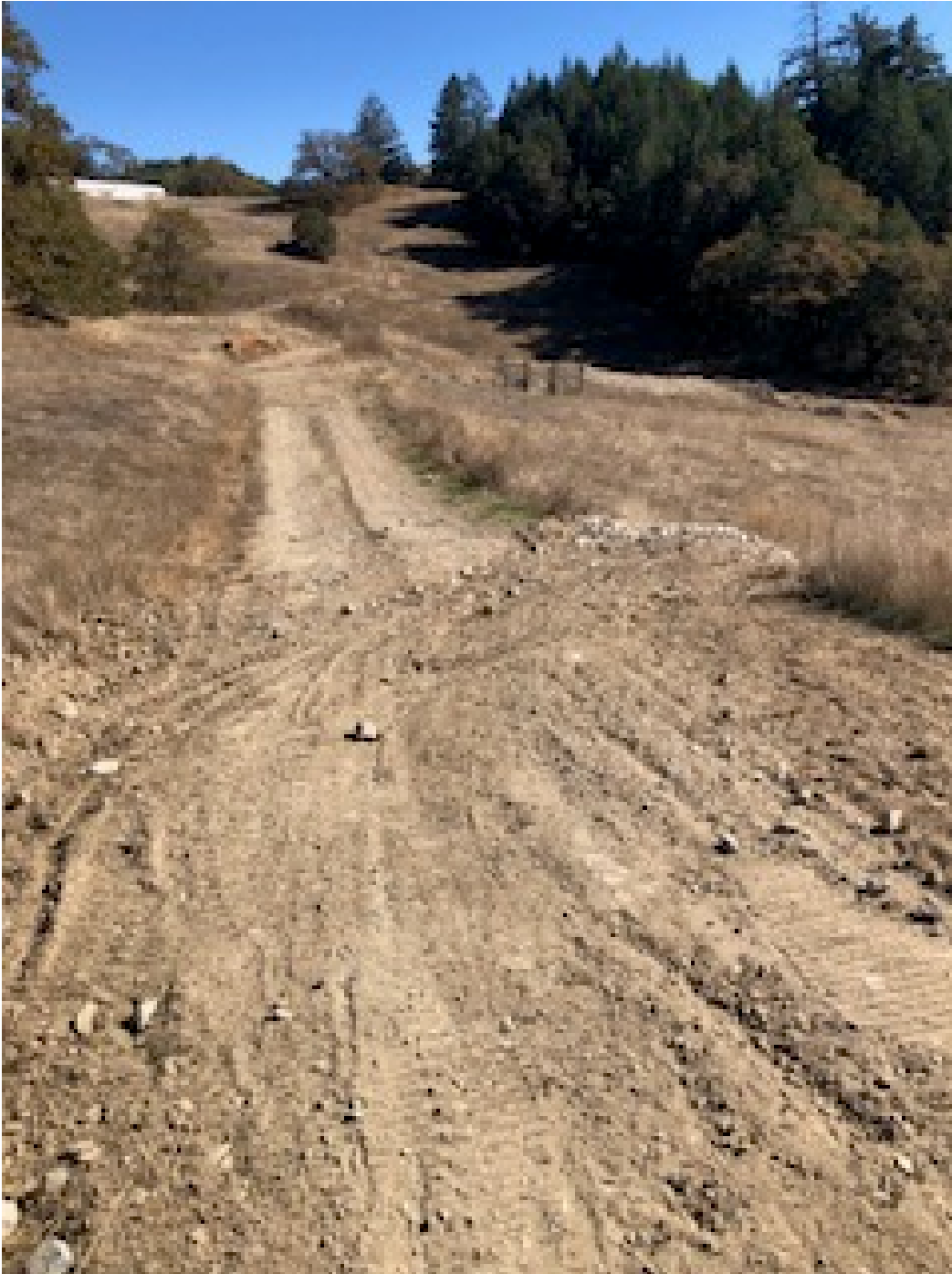
Figure 1: Looking NE to WB-1, the first waterbar east of the residence.
