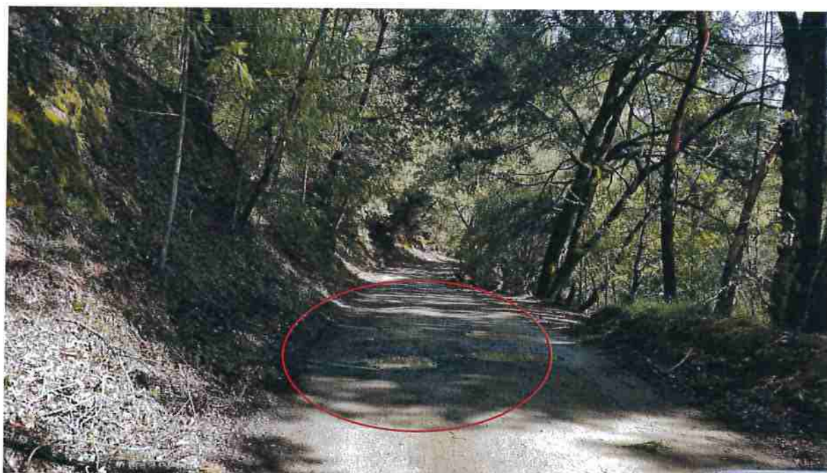
Figure 37. Photograph showing road point RP39 where the roadway has pot-holes. The roadway surface needs to be regraded in this.
