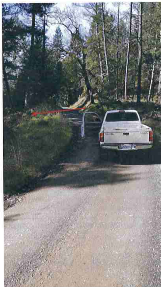
Figure 53. Photograph showing concentrated flow on the roadway surface at road point RP58. A rolling dip need to be installed to prevent concentrated flow on the roadway surface.
