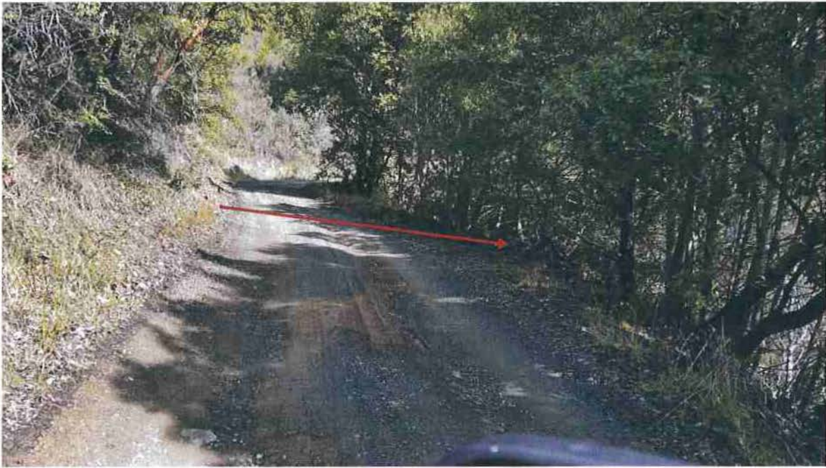
Figure 32. Photograph showing road point RP34 where water is channelizing on the roadway surface. A rolling dip needs to be created to divert the concentrated roadway runoff off of the roadway surface.
