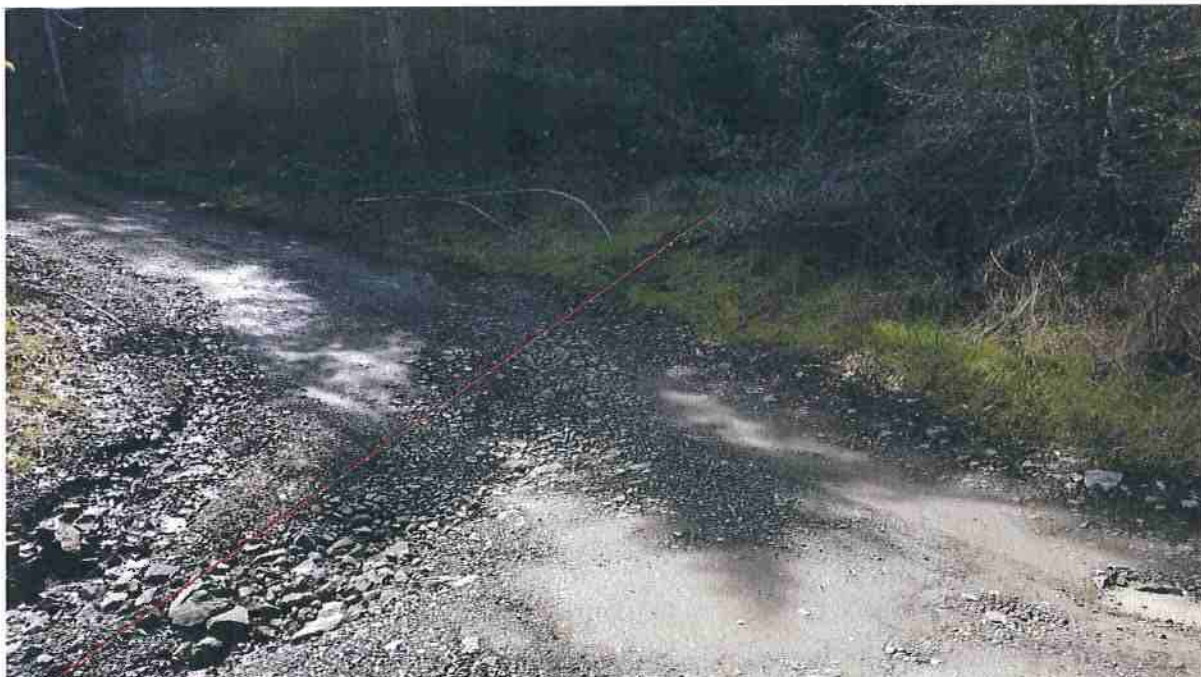
Figure 6. Photograph showing road point RP4 which is at an intersection to a neighboring roadway. The neighboring access roadway lacks a proper drainage the start of a class three watercourse intersect the roadway at the intersection. A culvert needs to be installed at the start of the class III watercourse
