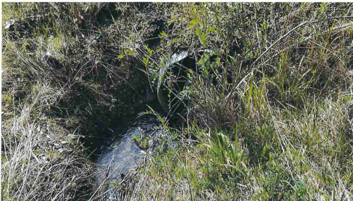
Figure 17. Photograph showing road point RP16 which is a 24 inch culvert on a class III watercourse that needs debris cleared from the inlet. The culvert is in good condition..
