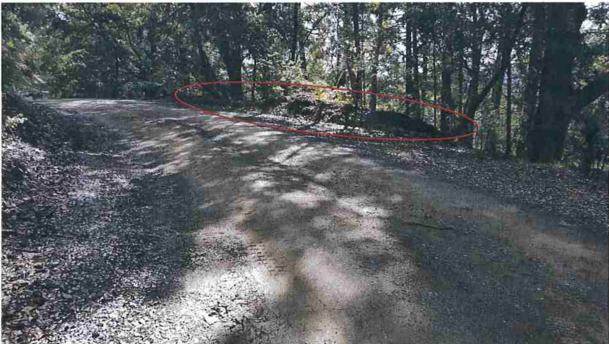
Figure 39. Photograph showing road point RP41 where a pullout needs to be expanded by grading the outside berm back onto the roadway.
