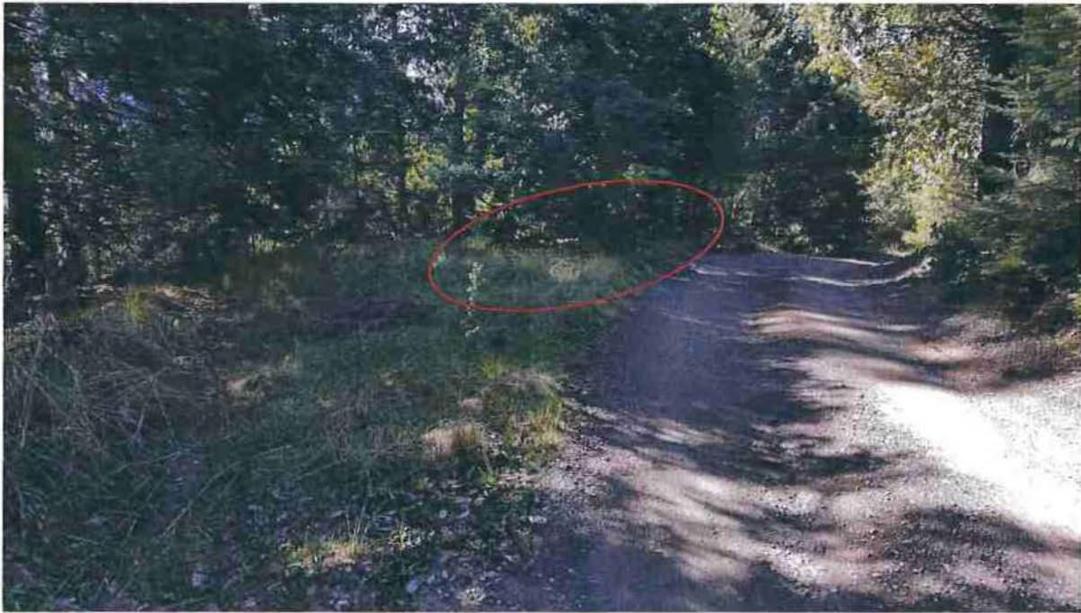
Figure 25. Photograph showing road point RP24 which is a pullout that needs brush to be cleared and to be regraded.
