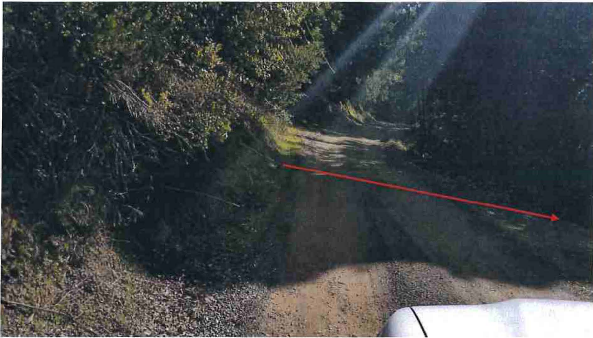
Figure 40. Photograph showing road point RP43 where a rolling dip needs to be created to disconnect the roadway surface from the watercourse approximately 100' south-west of RP43.
