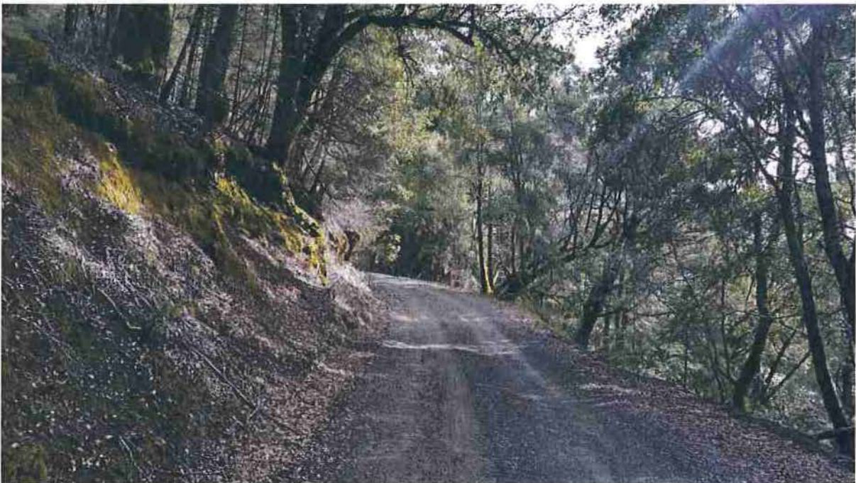
Figure 43. Photograph showing narrow section of roadway located at RP46.
