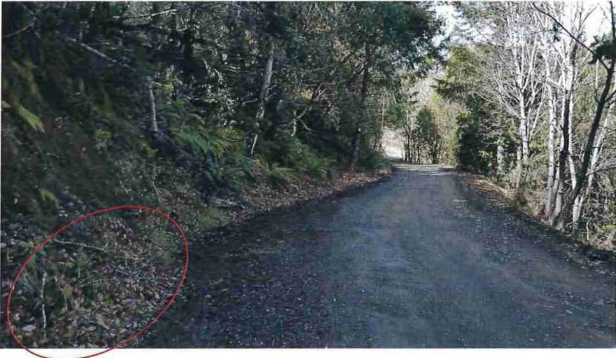
Figure 9. Photograph showing road point RP7 which is turnout that needs to be regraded.
