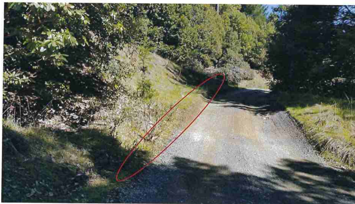
Figure 24. Photograph showing road point RP23 which is a section of roadway that needs to be regraded. Regrading needs to widen the roadway and re-establish an inside ditch.
