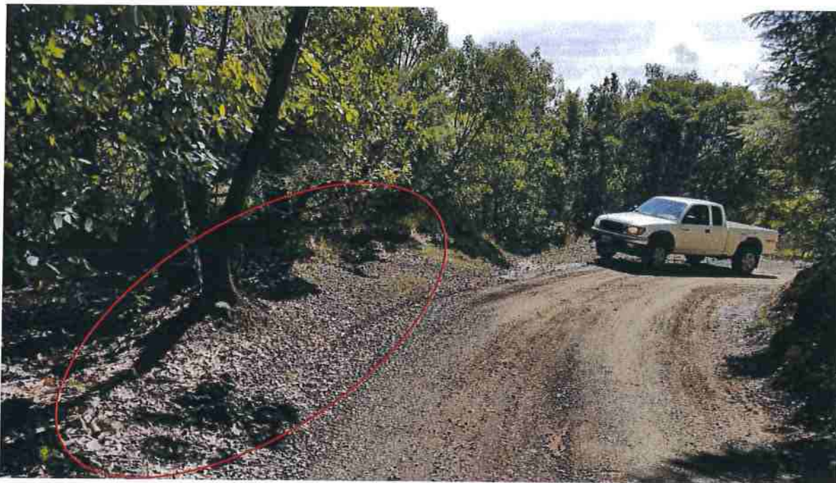
Figure 23. Photograph showing road point RP22 which is a pullout that needs a two tree to be removed and to be regraded.
