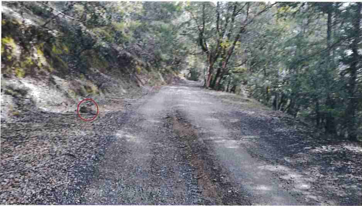
Figure 44. Photograph showing a pullout located at road points RP47 with a rock that needs to be cleared from the pullout..
