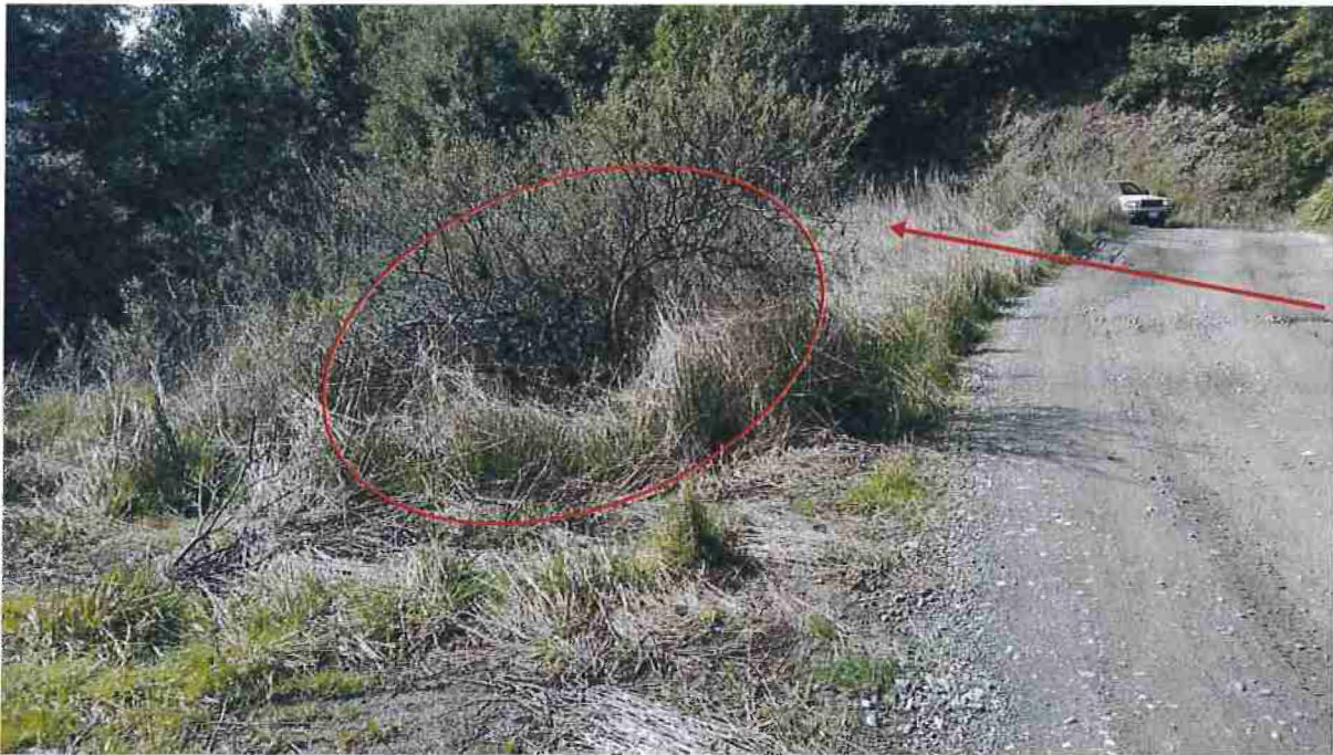
Figure 30. Photograph showing road point RP31 that is a pullout that needs brush to be cleared and regraded to create a turnout and a rolling dip to disconnect the roadway surface from the watercourse located at RP32.
