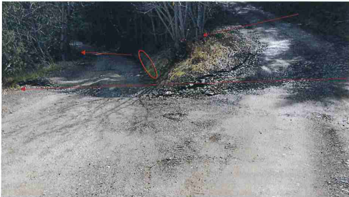
Figure 7. Photograph showing road point RP5 which is at an intersection to a neighboring roadway. The neighboring access roadway lacks a proper drainage the start of a class three watercourse intersect the roadway at the intersection. A culvert needs to be installed at the start of the class III watercourse crossing both of the access roads and a drainage relief culvert needs to be installed below the intersection to catch the runoff from need to be installed rolling dip installed approximately 50' up the neighboring property. The roadways inside ditch need to be installed from the proposed drainage relief culvert to the intersection.
