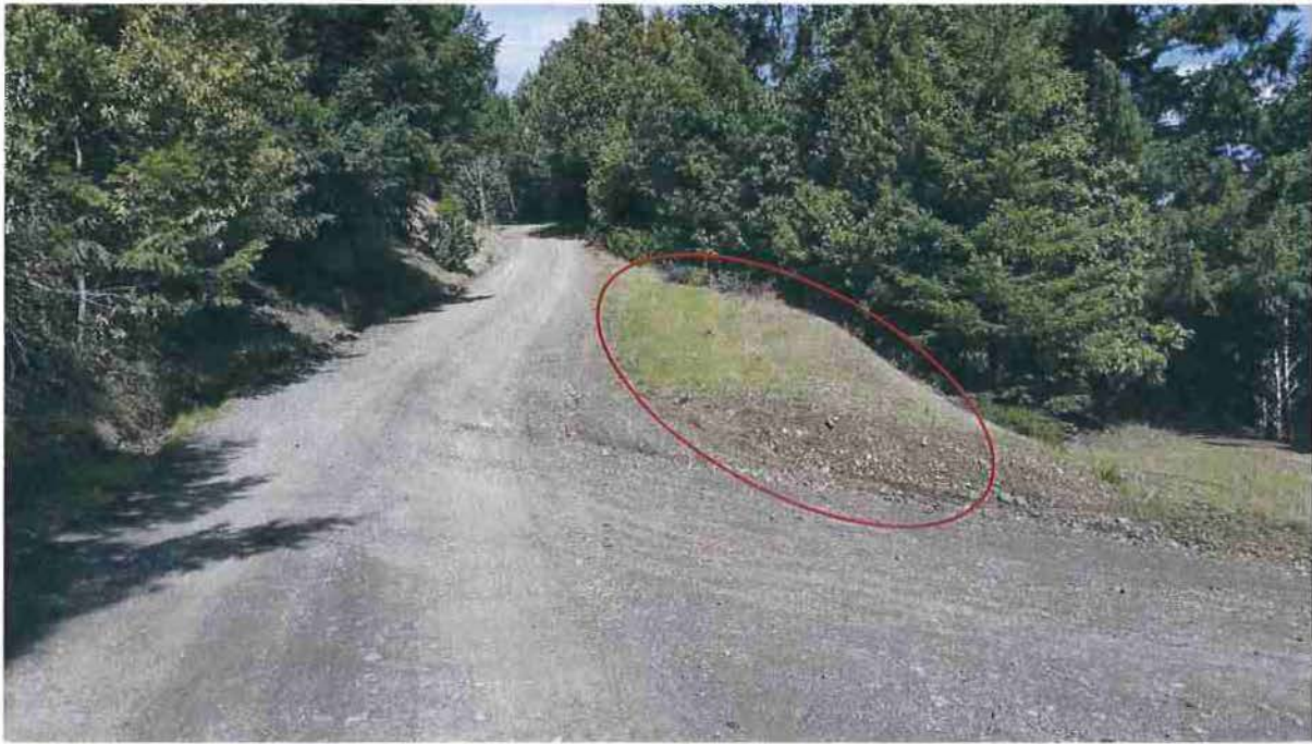
Figure 11. Photograph showing road point RP9 which is a pullout at an intersection that needs to be regraded to make the transition into the intersection smoother.
