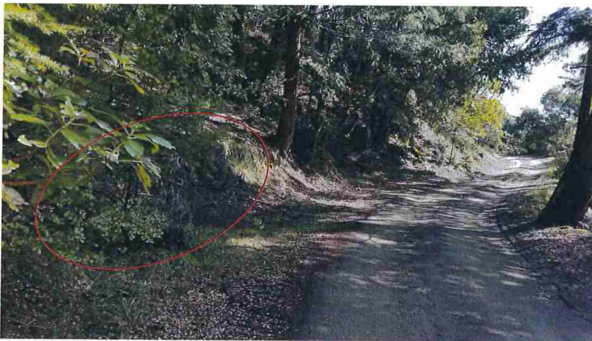
Figure 36. Photograph showing road point RP38 where a pullout needs brush cleared.
