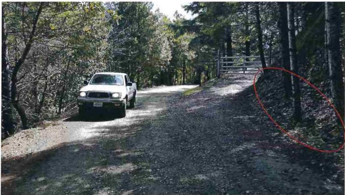
Figure 10. Photograph showing road point RP8 which is turnout that needs trees to be removed from the inboard ditch and to be regraded.
