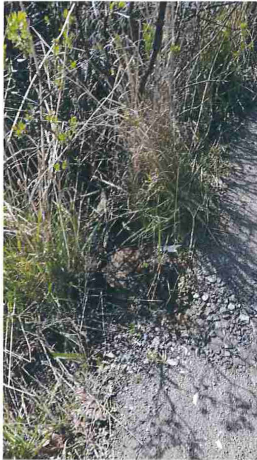
Figure 29. Photograph showing road point RP27 which is a failing culvert that drains a class II stream/spring area below a water tank. The culvert needs to be replaced which will require a 1600 and additional permitting.
