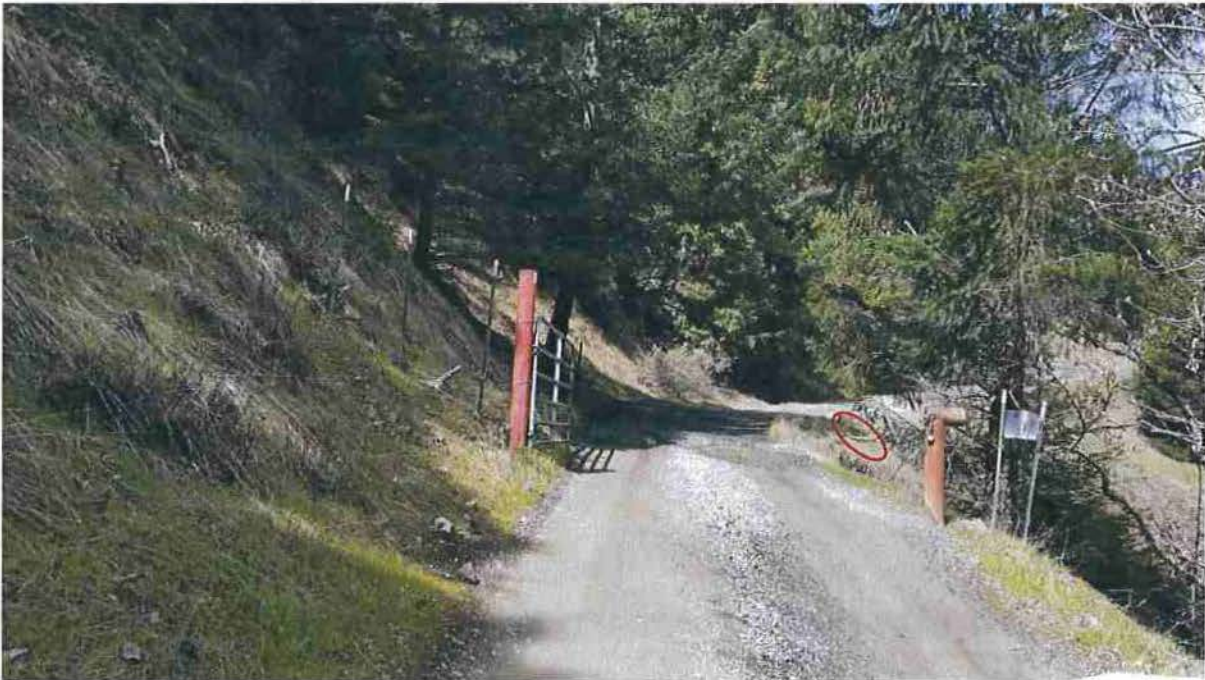
Figure 12. Photograph showing road point RP11 is a gate with pullout on either side. On the east side of the gate is drainage relief culvert that needs to be extended by approximately 10' (RP10)
