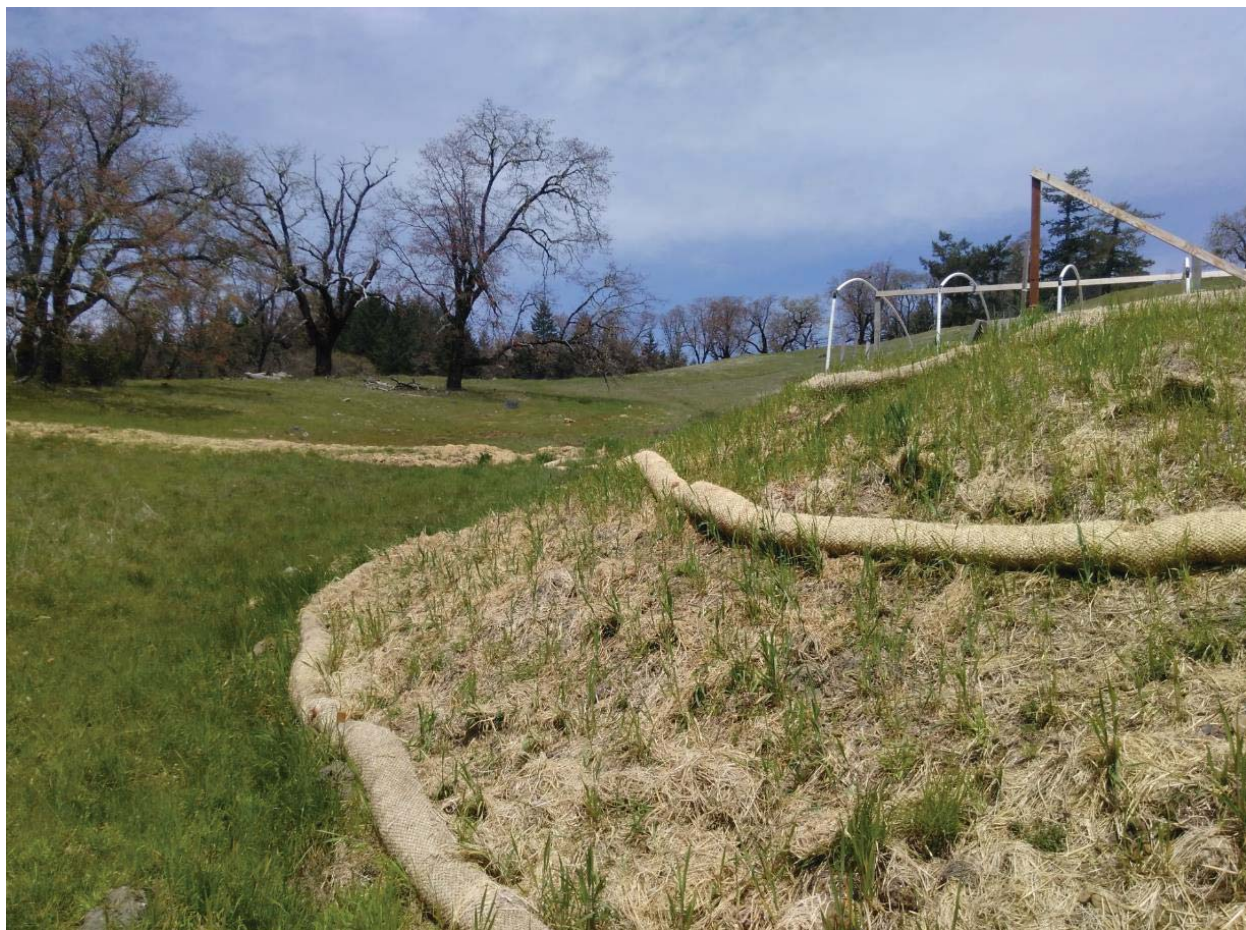
SW corner of CA-3 showing strawing and waddles installed. Drainage for Class III is in lower left corner of photo, not a very defined channel, very vegetated, waddle installed in channel. Retake of OP-4
