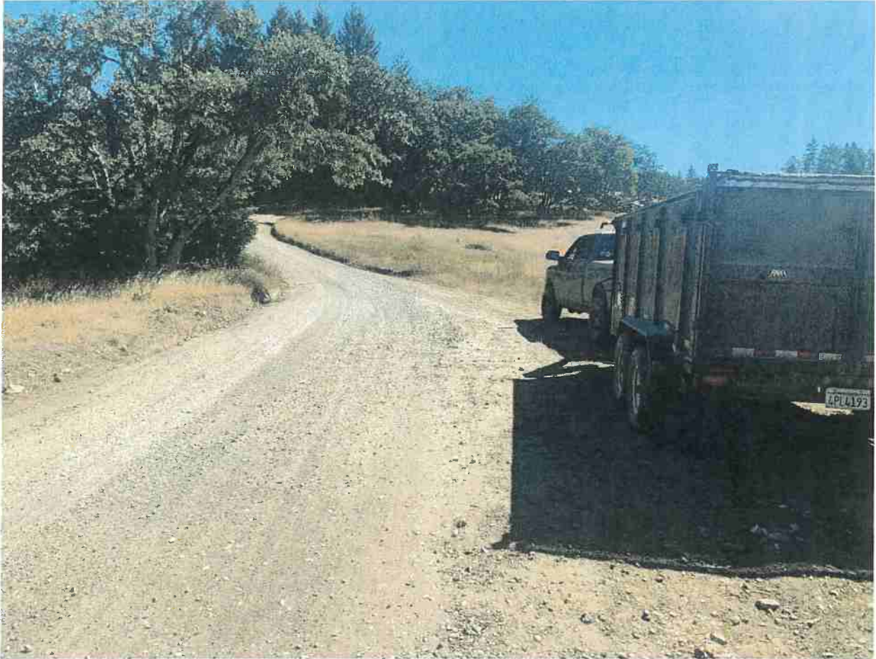
Mm —.25. Photos 2/3 large pull out and recently graded road with new ditches for proper water drainage
