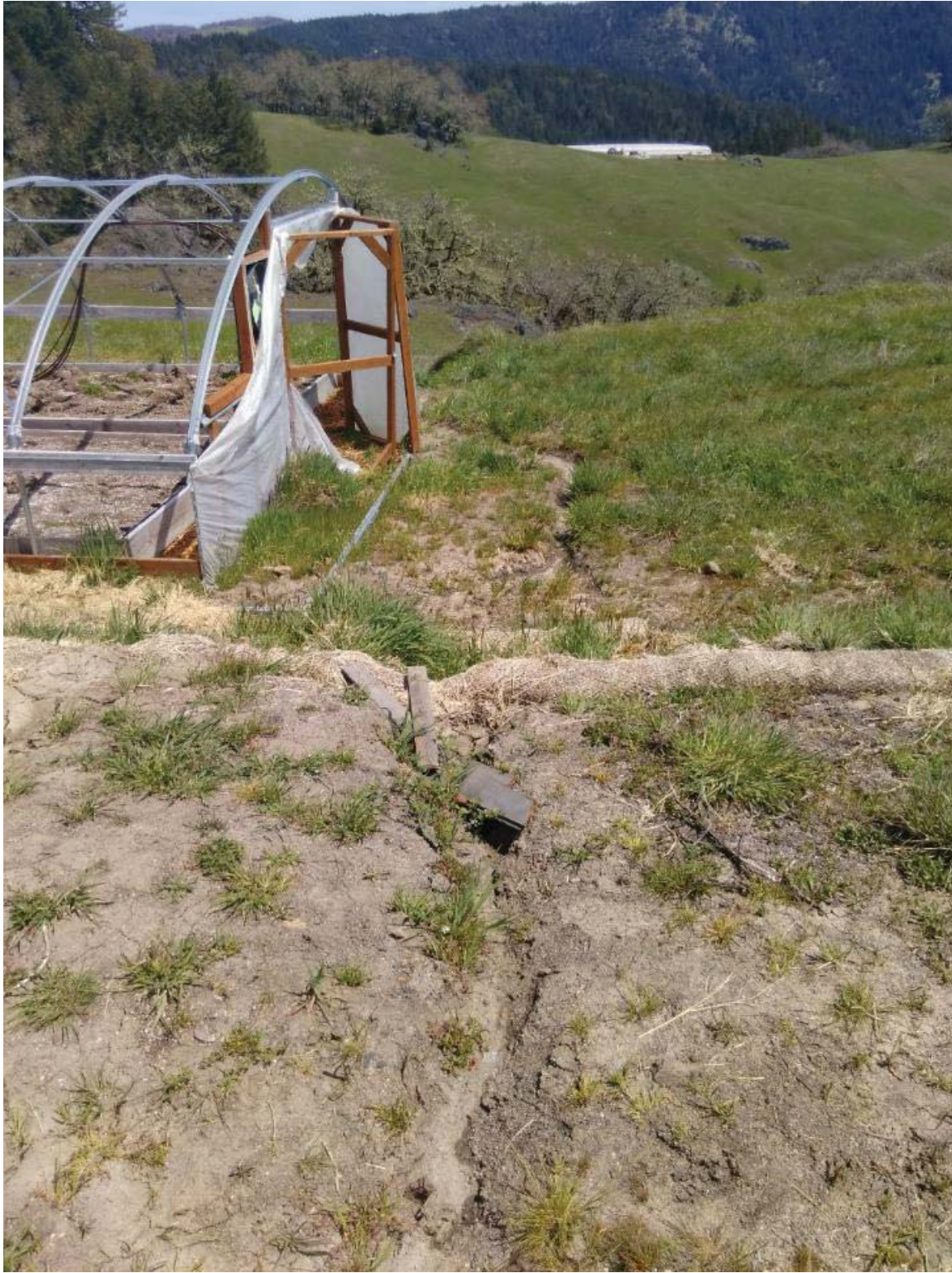
Eroding drainage channel at the SE corner of CA-5. Silt fence to be installed at lower perimeter.
