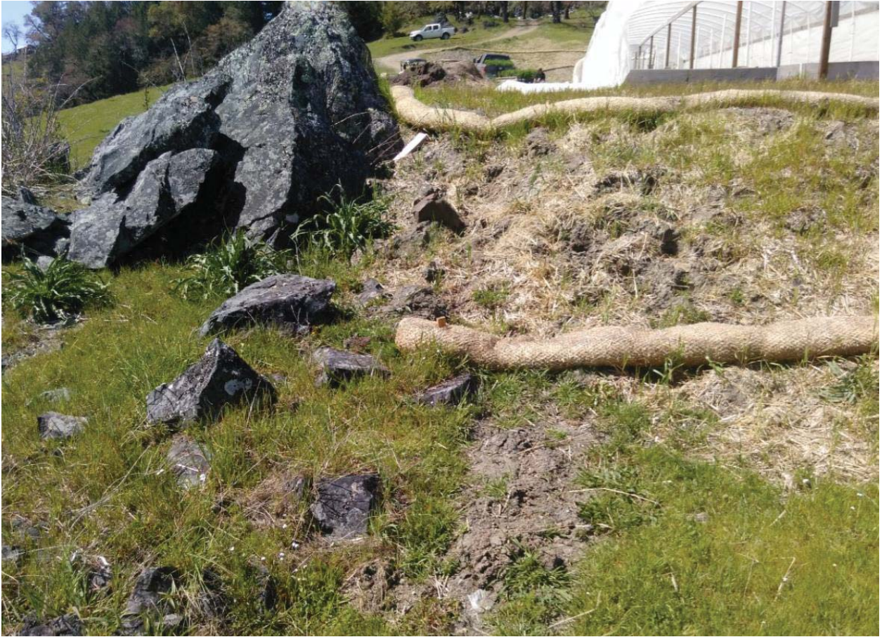
Drainage outlet at SE corner of CA-6. Silt fence to be installed
