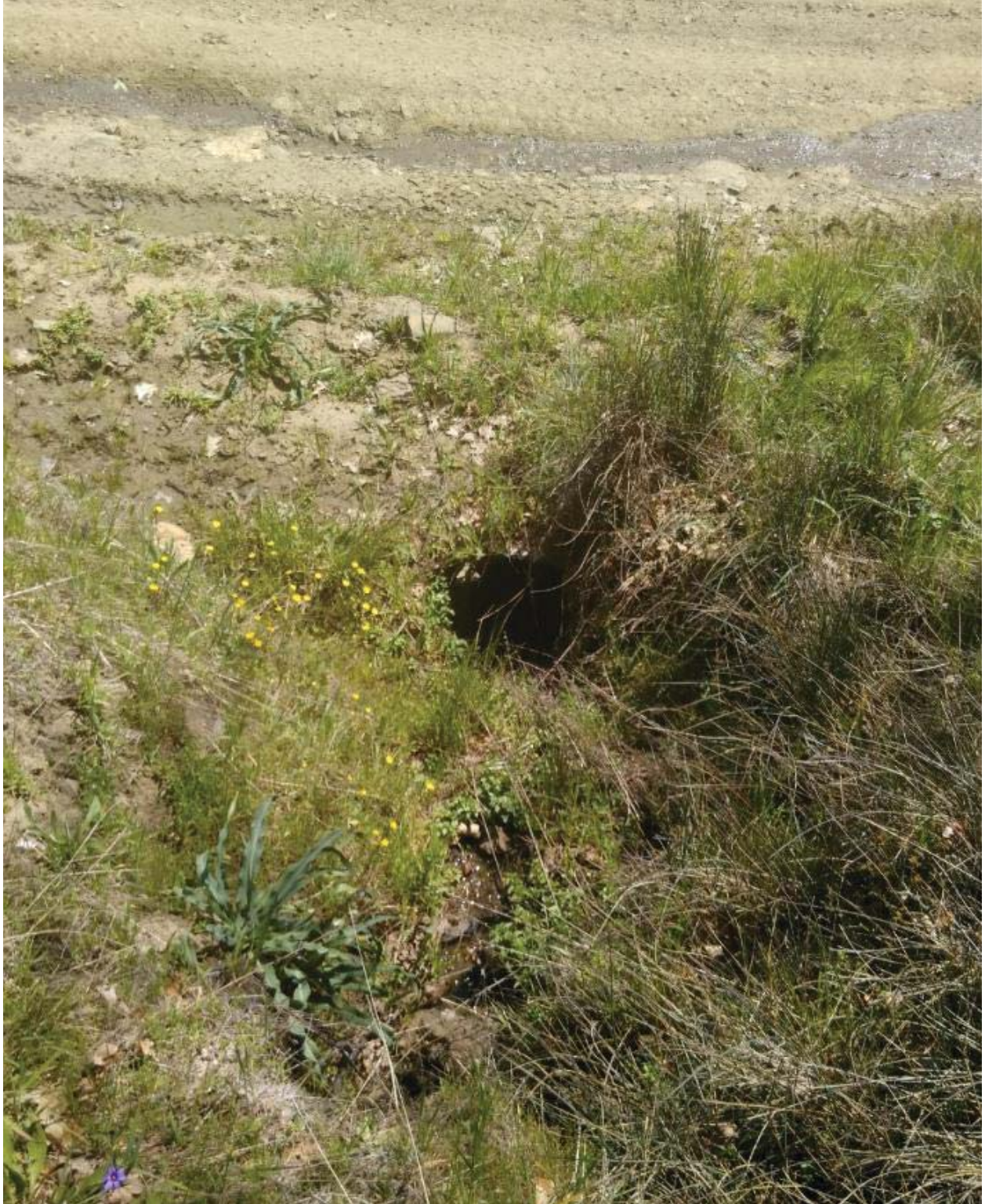
Inlet of CV-1
