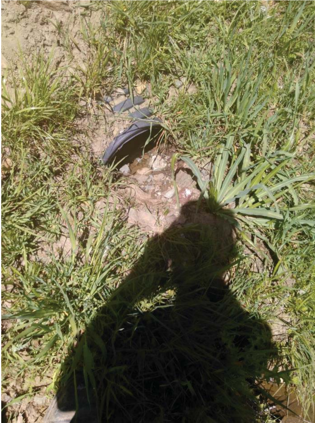
Outlet of CV-1 is inundated
