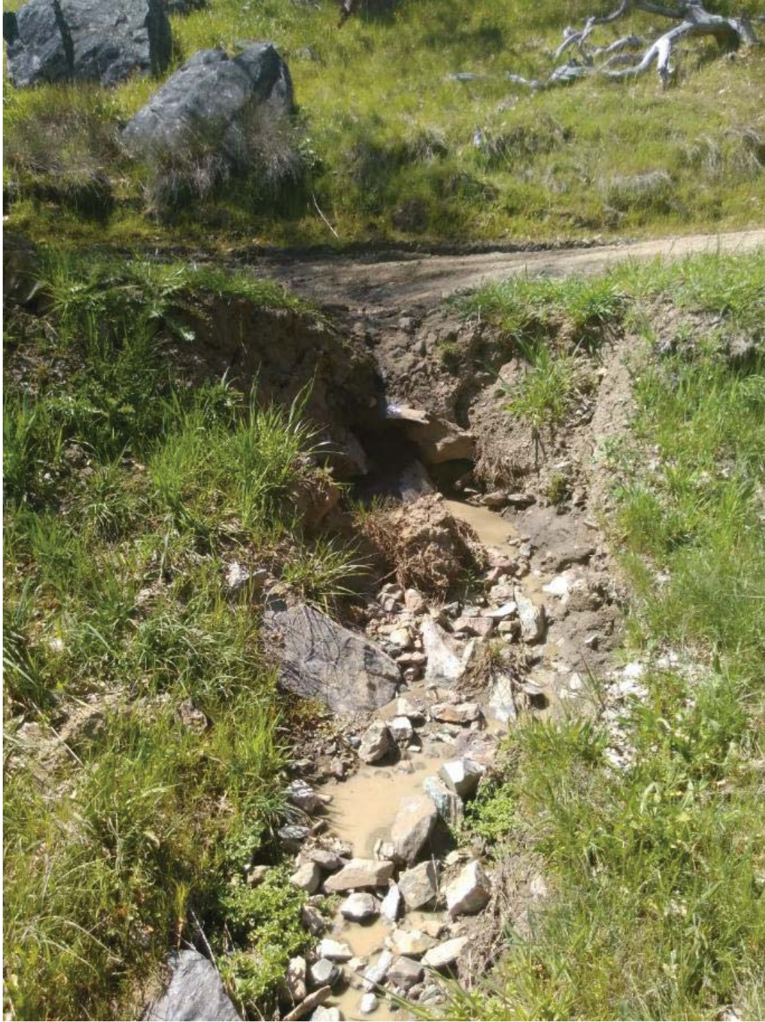
AC-1. View of erosion on the downslope side caused by hydrologic connectivity.
