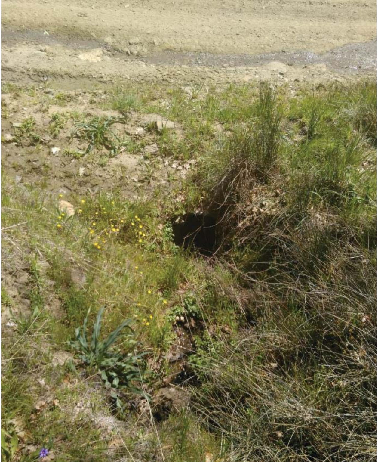
Inlet of CV-1
