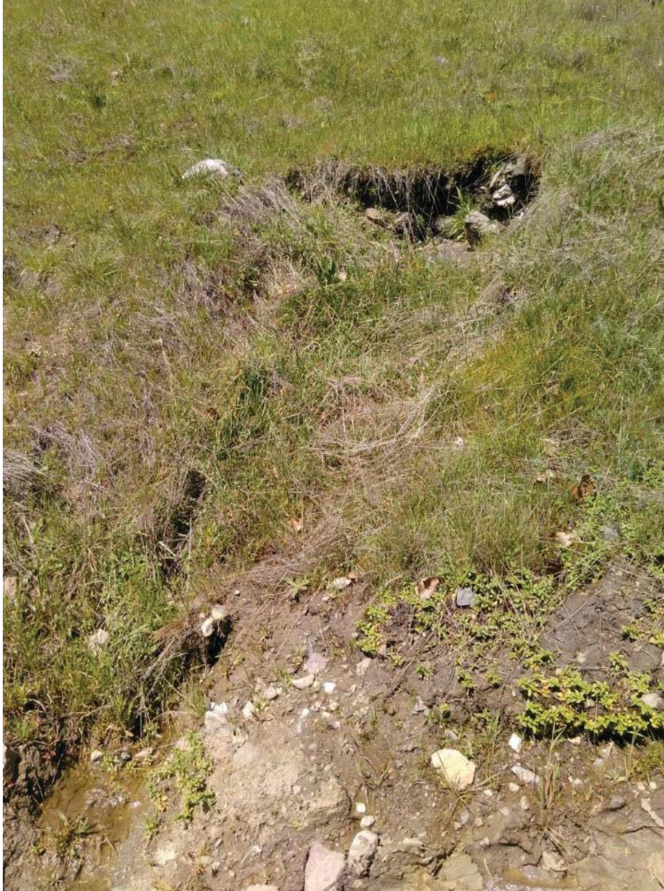
CV-3 proposed stream crossing. Site of a seep that intercepts roadway with no conveyance.
