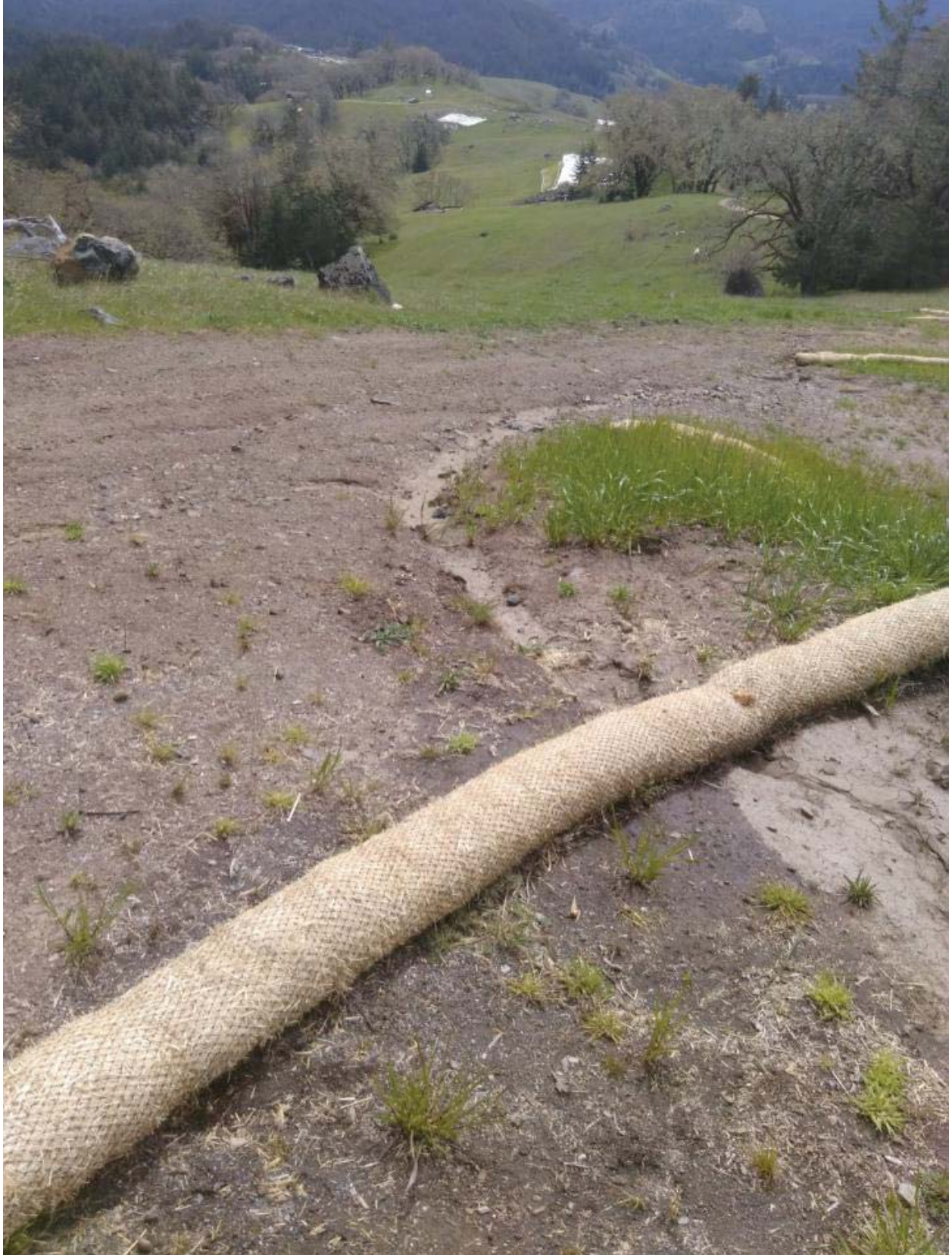
CA-1, closeup on channelized runoff
