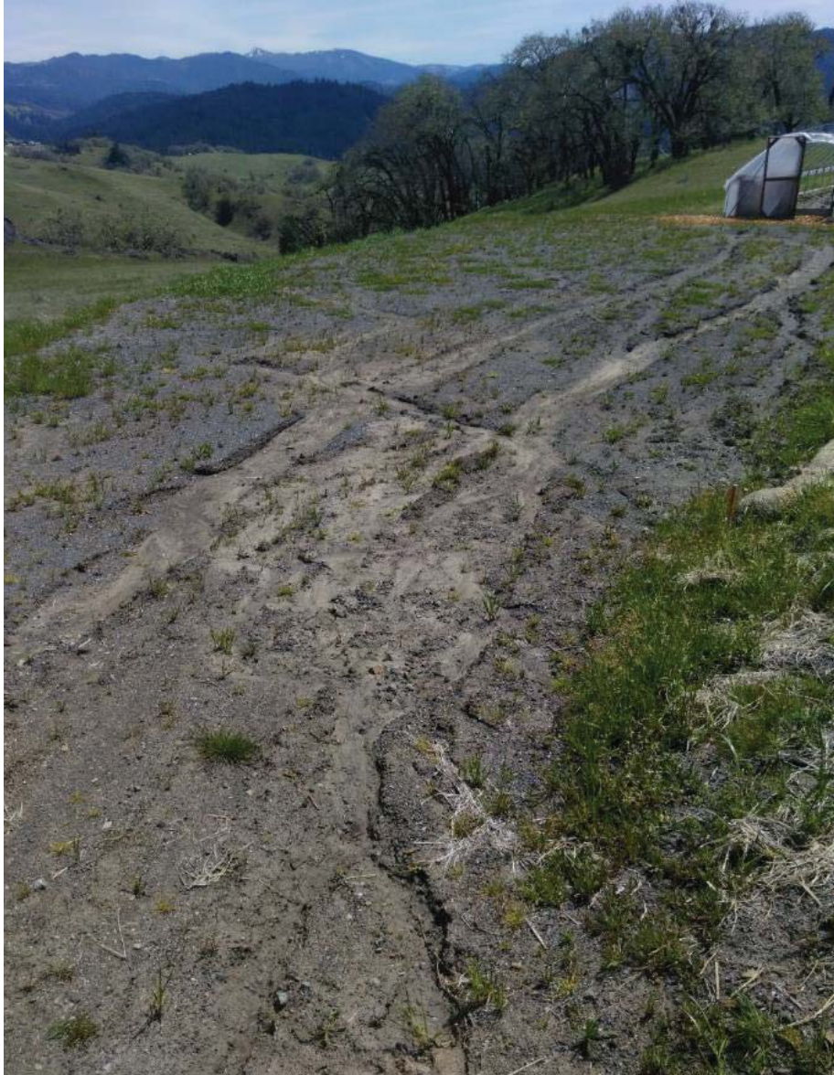
Landing at the NE corner of CA-5 showing channelization and erosion from runoff
