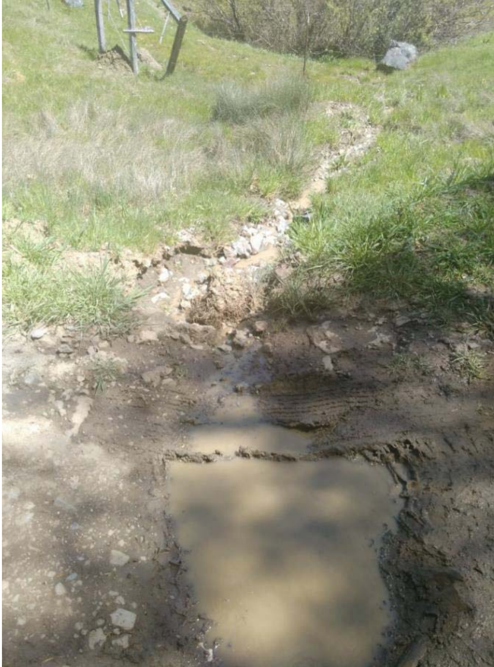
AC-1. Looking downhill from roadway. Inadequate drainage of access road and contributing hillside seeps causing erosion and sediment transport. Road improvements and armored crossing proposed.
