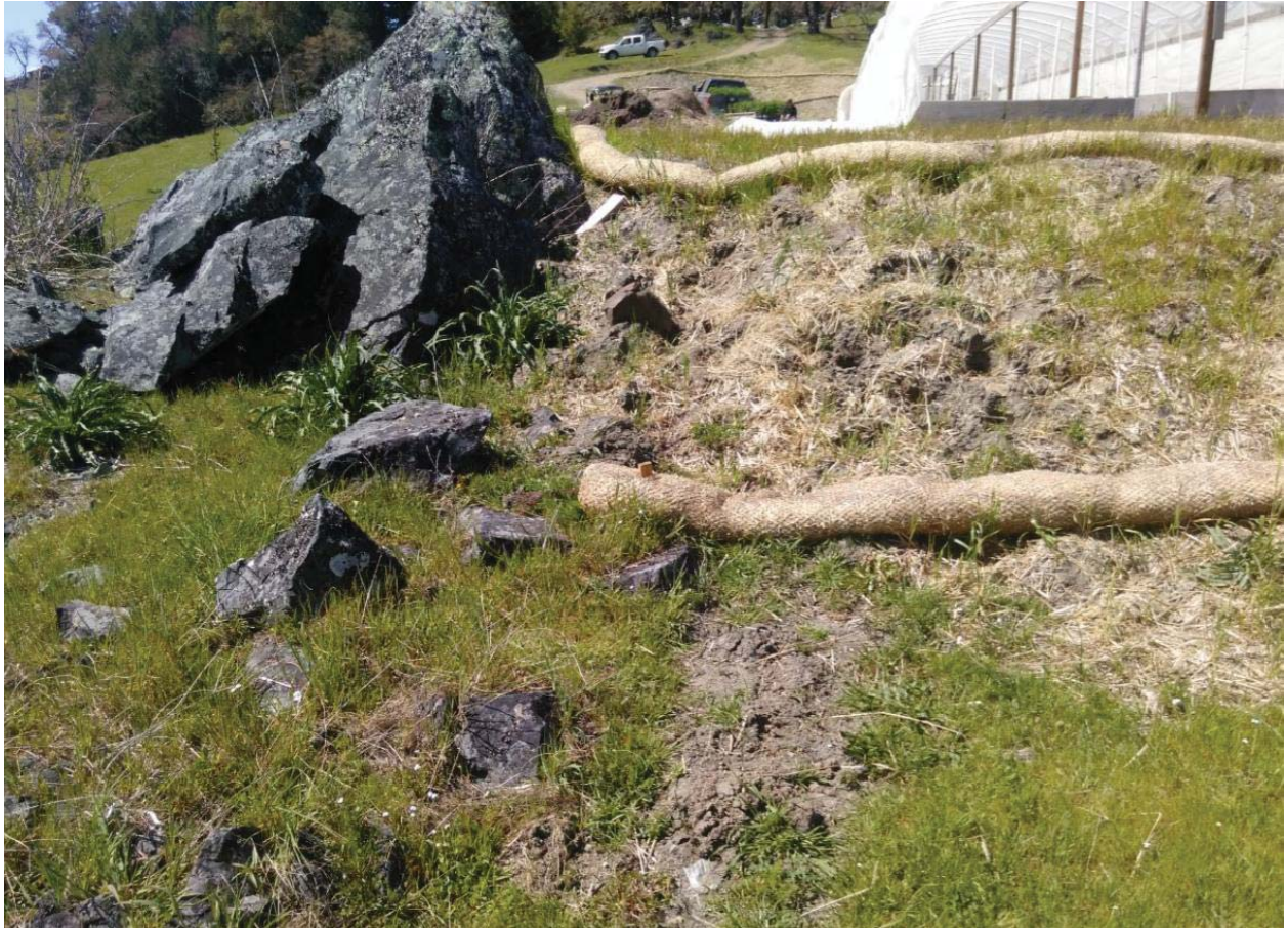
Drainage outlet at SE corner of CA-6. Silt fence to be installed
