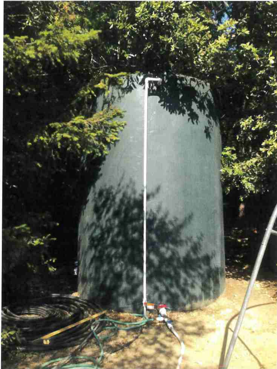
Photo 10: One 5,000 gallon poly storage tank. Photo date 9-8-16
