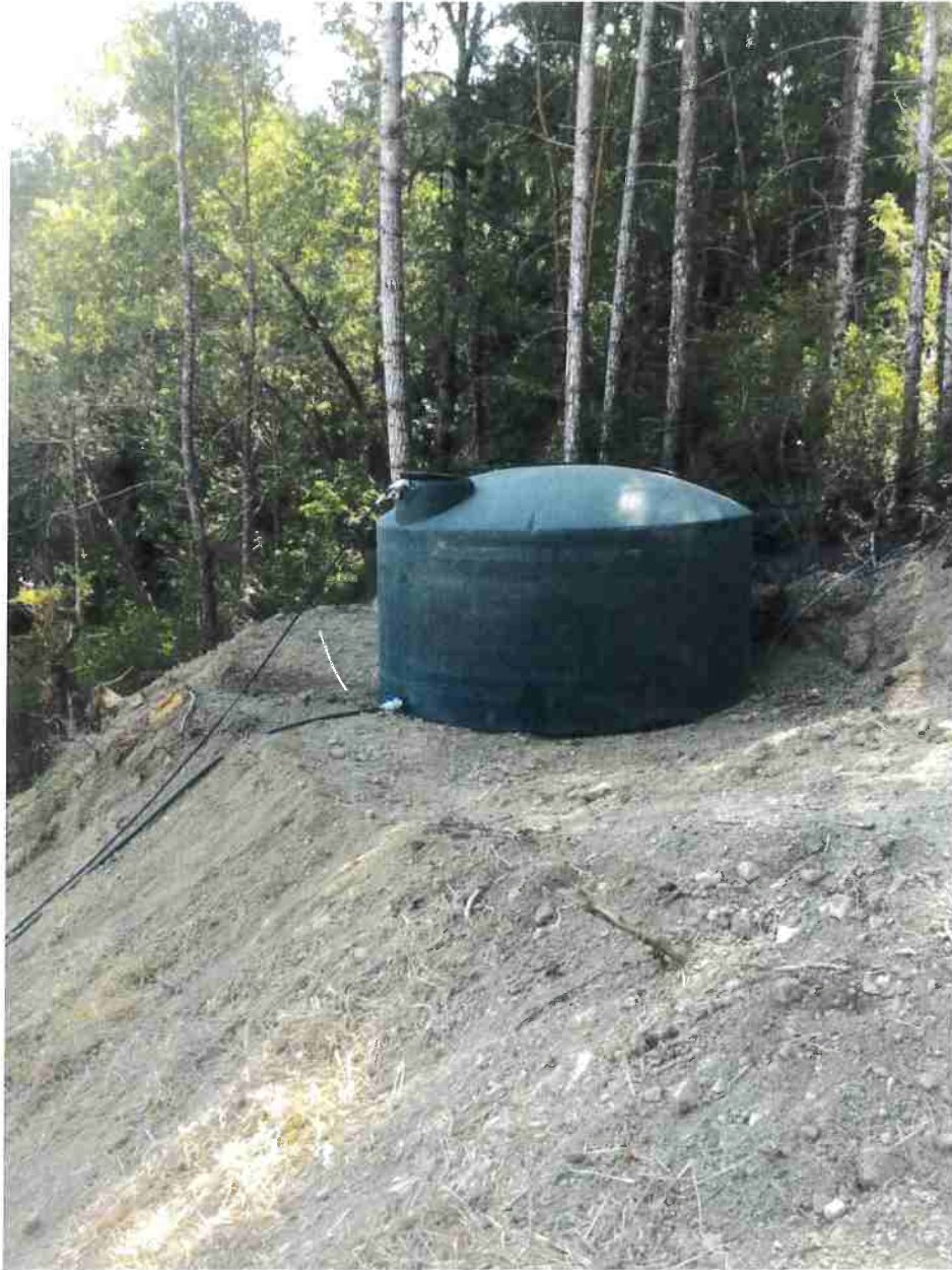
Photo 11: One 5,000 gallon poly storage tank. Photo date 9-8-16
