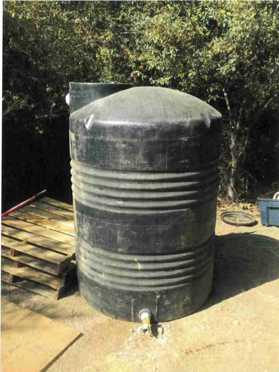
Photo 13: One 500 gallon mixing/feed tank. Photo date 9-8-16
