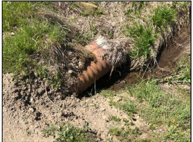
Photo #160 Hidden Valley Rd Partially Clogged 18" Culvert In
