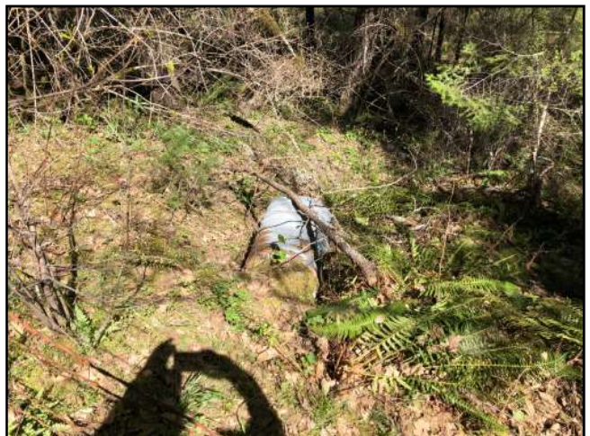
Photo #150 Hidden Valley Rd 18" Culvert Out
