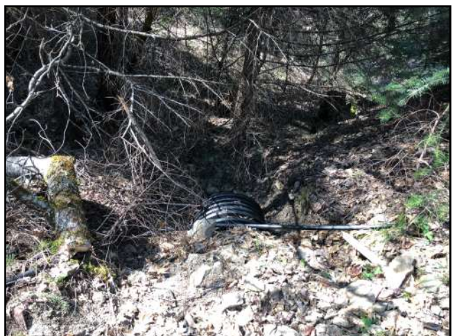
Photo #36 APN 210-074-008 Private Access Rd 18" Culvert Out
