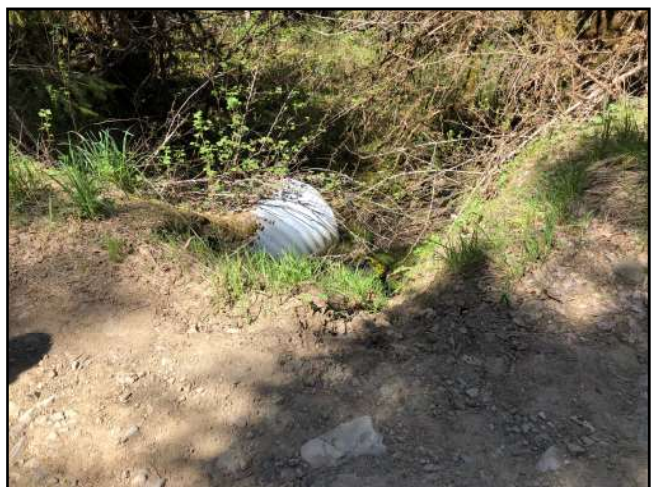
Photo #72 APN 210-074-008 Private Access Rd 18" Culvert Out
