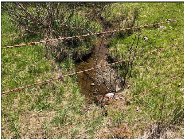
Photo #161 Hidden Valley Rd Partially Clogged 18" Culvert IOut
