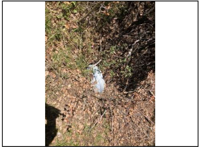
Photo #134 Hidden Valley Rd Partially Clogged 12" Culvert In
