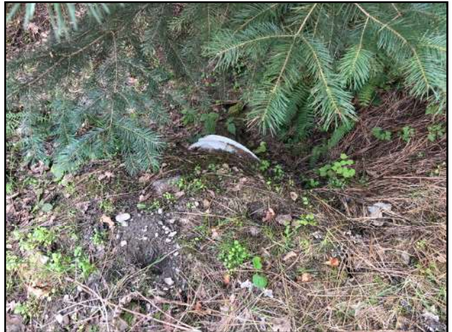
Photo #154 Hidden Valley Rd Partially Clogged 18" Culvert In
