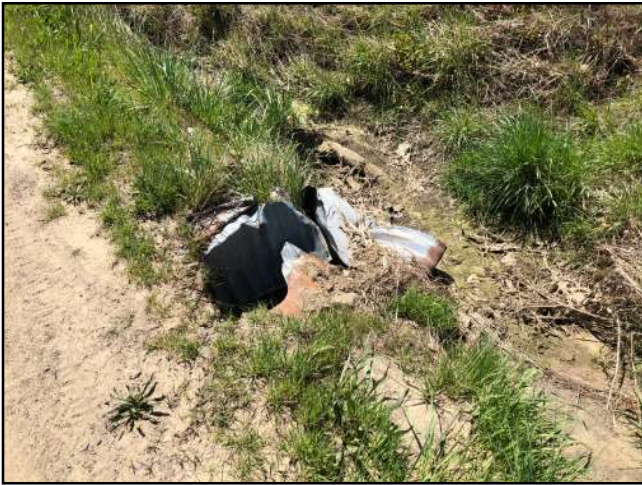
Photo #157 Hidden Valley Rd Clogged & Crushed 18" Culvert In
