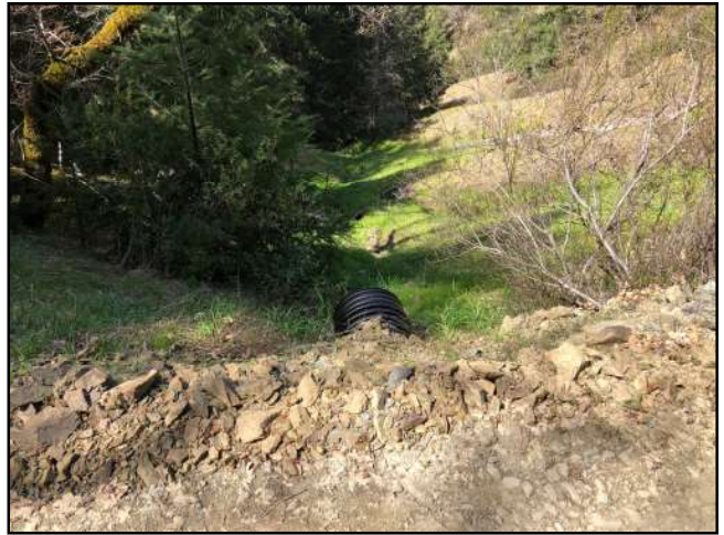
Photo #32 APN 210-074-008 Private Access Rd 18" Culvert Out
