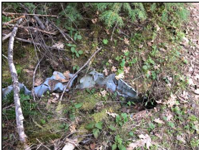
Photo #149 Hidden Valley Rd Clogged & Crushed 18" Culvert In
