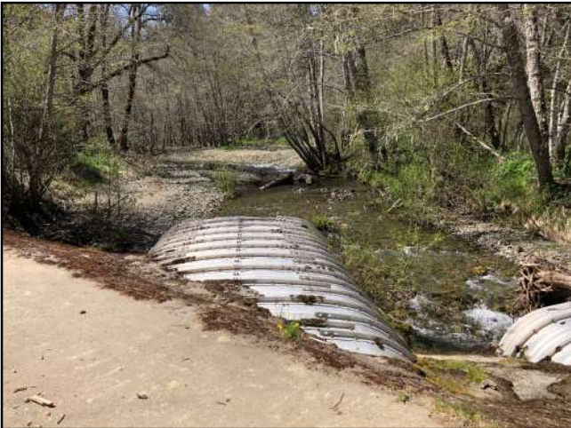
Photo #129 Hidden Valley Rd Double 120" Elliptical Culvert Out
