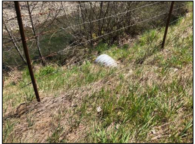
Photo #158 Hidden Valley Rd Partially Clogged 18" Culvert Out
