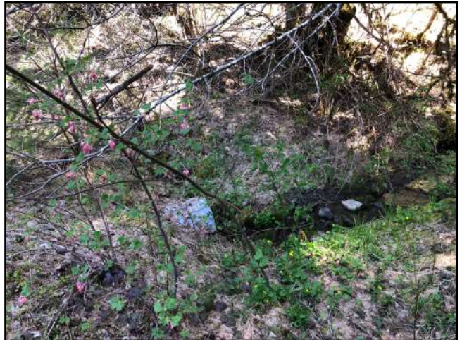
Photo #70 APN 210-074-008 Private Access Rd 18" Culvert Out
