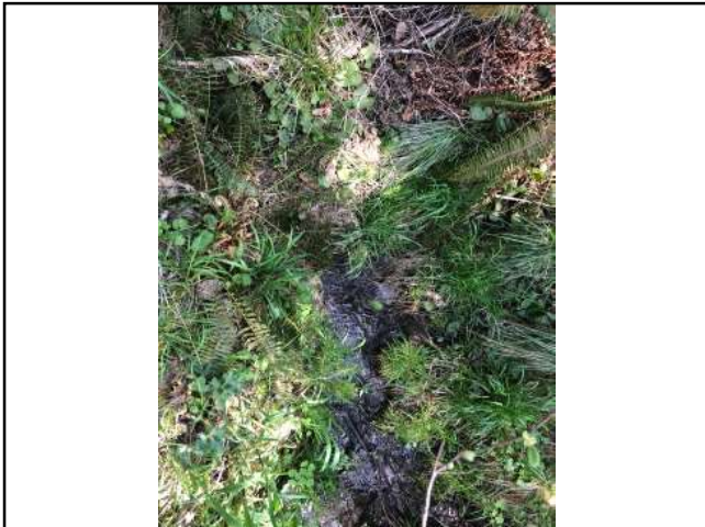
Photo #105 Hidden Valley Rd Partially Clogged 18" Culvert Out
