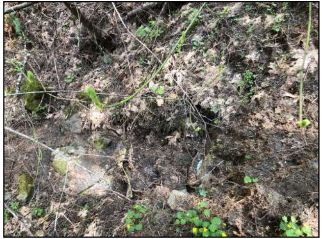
Photo #110 Hidden Valley Rd Partially Clogged 12" Culvert Out
