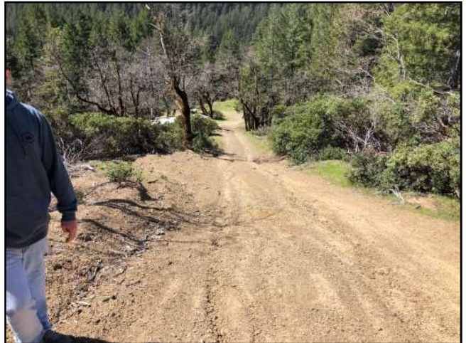
Photo #22 APN 210-074-008 Private Drive @ Turnout Looking SW @ Erosion
