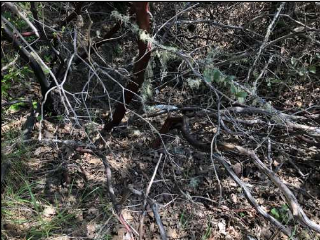
Photo #135 Hidden Valley Rd Partially Clogged 12" Culvert Out
