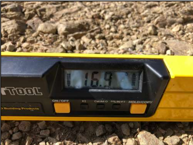
Photo #3 APN 210-074-008 Private Drive Slope 16.9%
