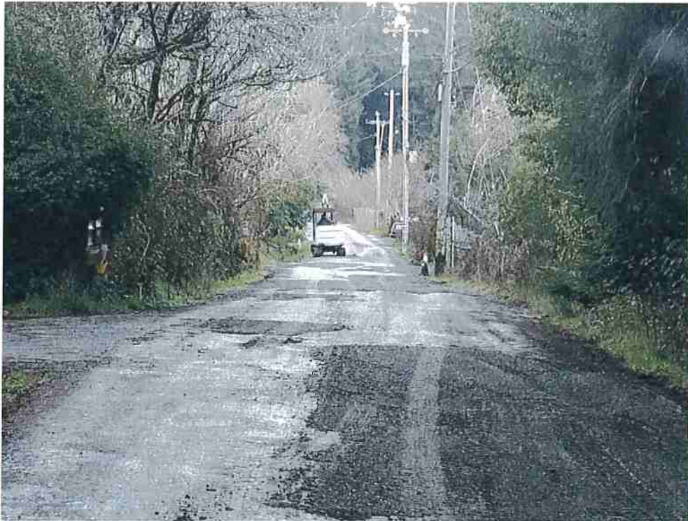
Figure 14: Potholes actively being filled presumably by a community member on January 9 th , 2020 around mile 1.1. Nice Work!
