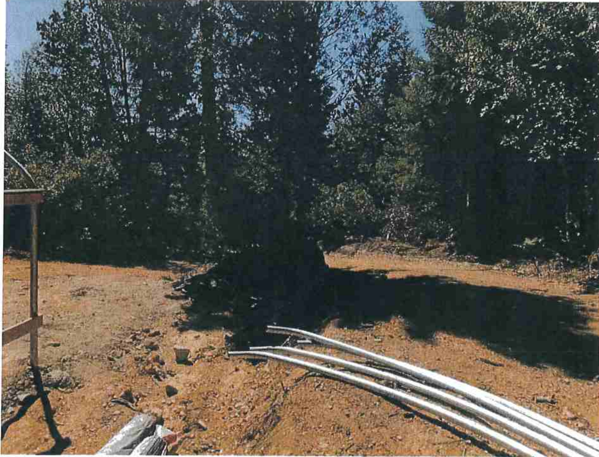
Photo #1: This is an image of the southern extent of Cultivation Area #6 (CA 6), where surface runoff is hydrologically connected to surface waters. The Discharger shall install a pipe at this location that channels the runoff beneath the road at the top right of the image, where it can disperse and infiltrate in the vegetation. Photo Date: 06/06/2017.
