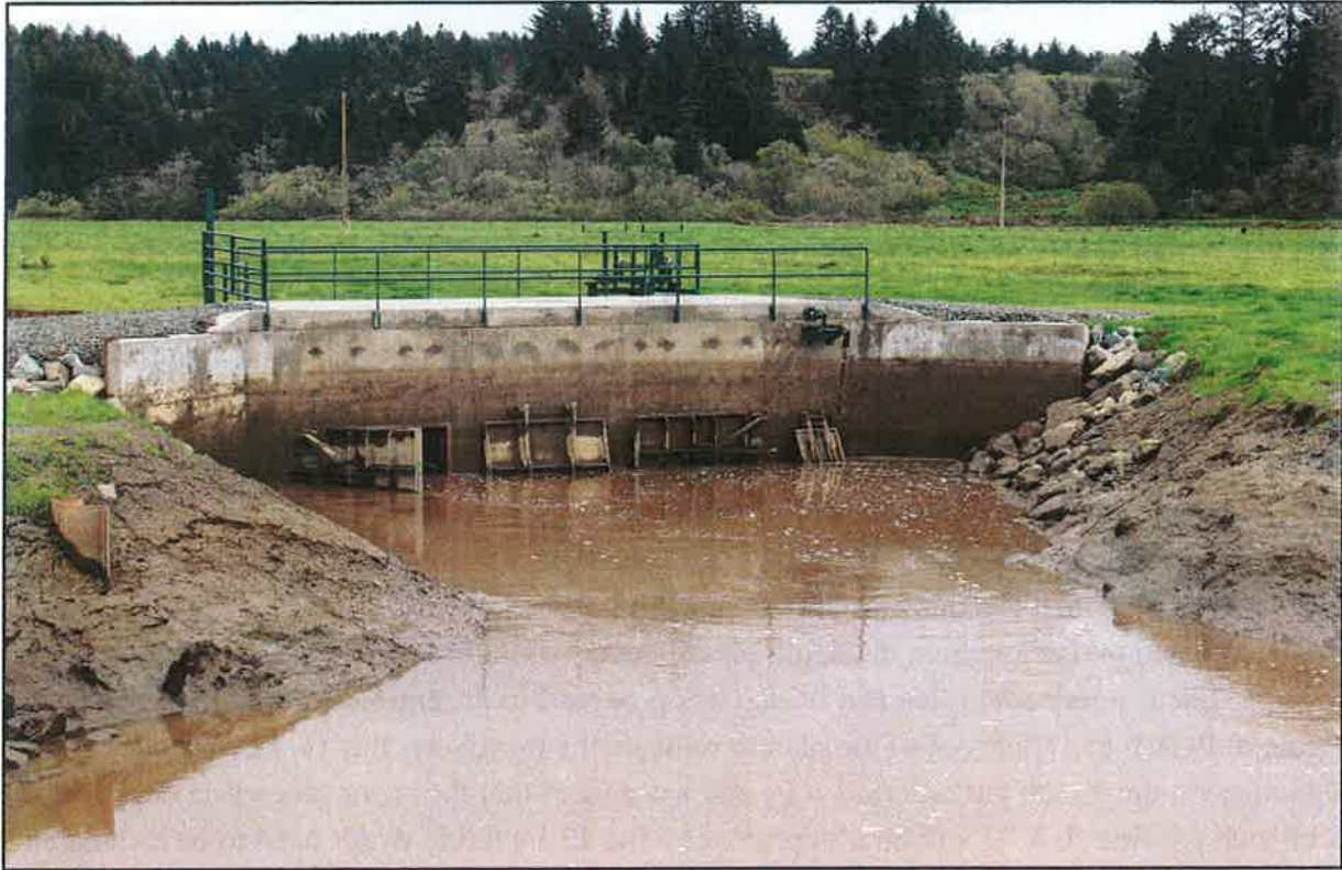
Martin Slough Tide gates, downstream side, showing the three 6' x 6' gates on the center and left and the 2' x 2' "habitat door" on the right.
