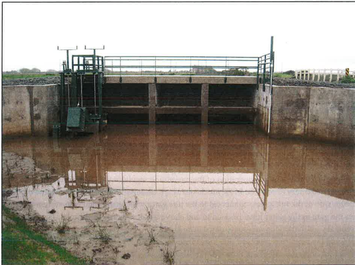
Martin Slough Tide gates, upstream side, showing the two MTR floats at left
