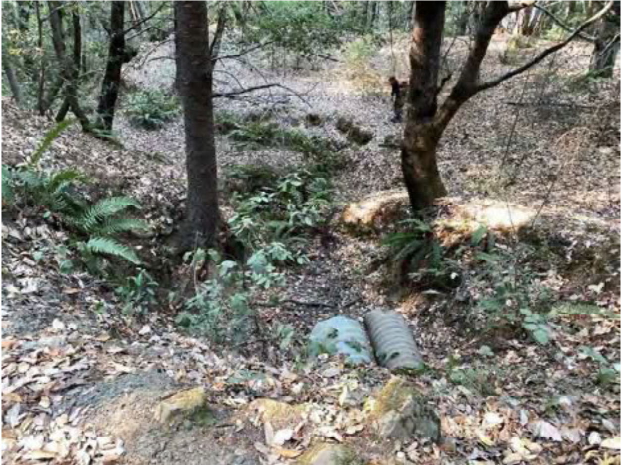
Photo 62: Stream Crossing 23. Looking downstream from the outlet of stream crossing 23. Photo date 9-1-2021.
