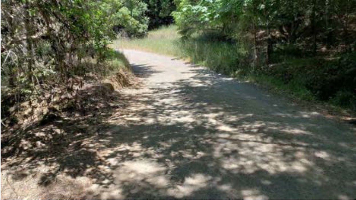
Site 13. Looking up grade at Site 13. A Class III watercourse is diverted down the inside ditch to the right. Re-alignment of this watercourse will consist of a culvert installed diagonally across the road from the grass patch in the upper center right to the lower left of the photo.
