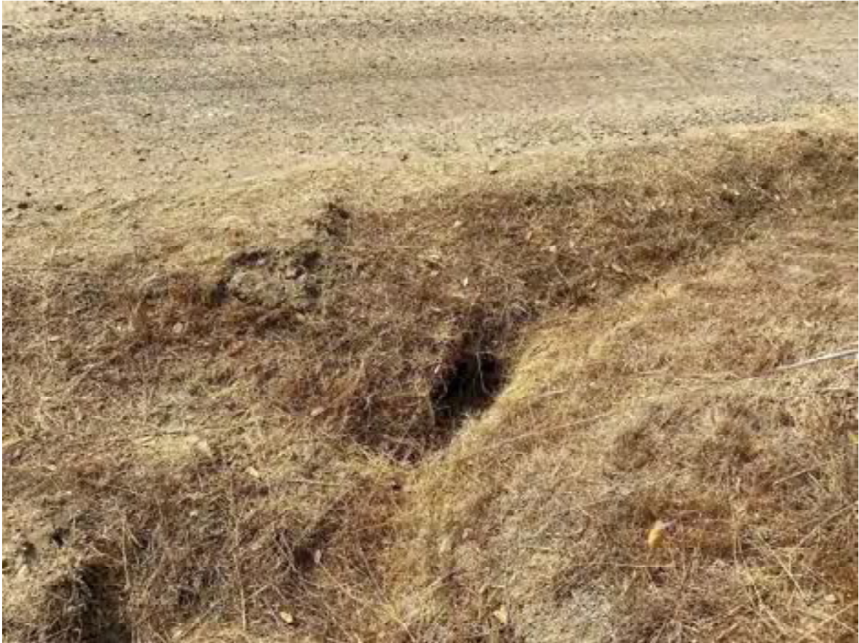
Photo 11: Stream Crossing 04. Looking downstream towards the inlet of the 8-inch diameter culvert at stream crossing 04. Photo date 9-1-2021.
