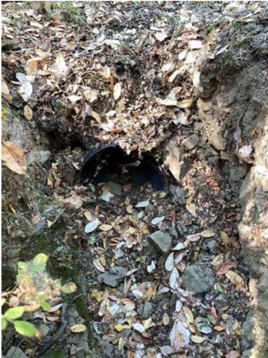
Photo 47: Stream Crossing 17. Looking downstream towards the inlet of the 18-inch diameter culvert at stream crossing 17 that is proposed for removal. Photo date 9-1-2021.
