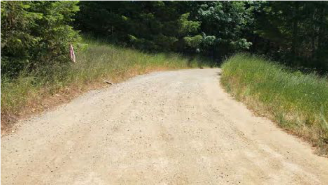
Site 12. Hydrologic disconnect for Sites 13, 14, and 23.
