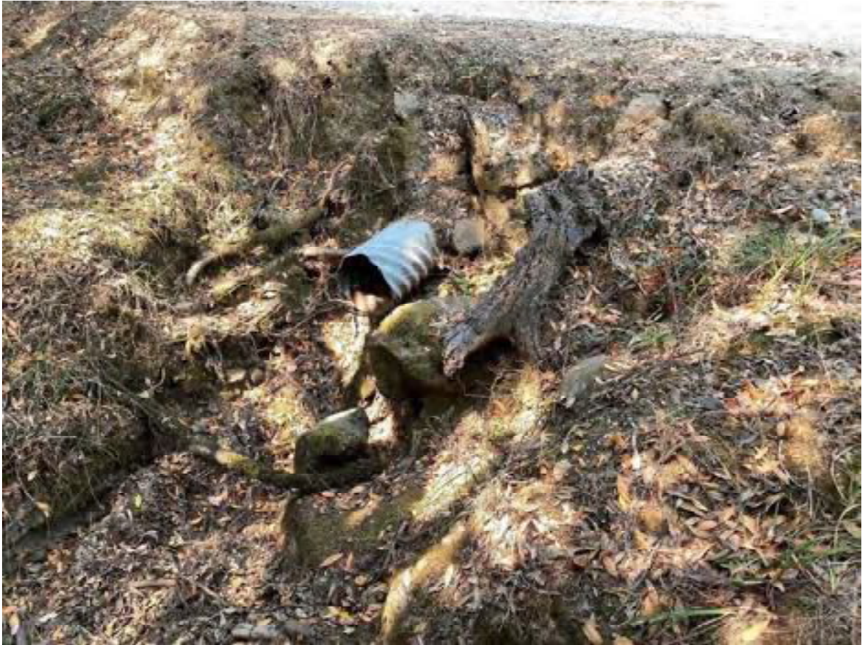
Photo 23: Stream Crossing 06. Looking upstream towards the outlet of the 12-inch diameter culvert at stream crossing 06. Photo date 9-1-2021.
