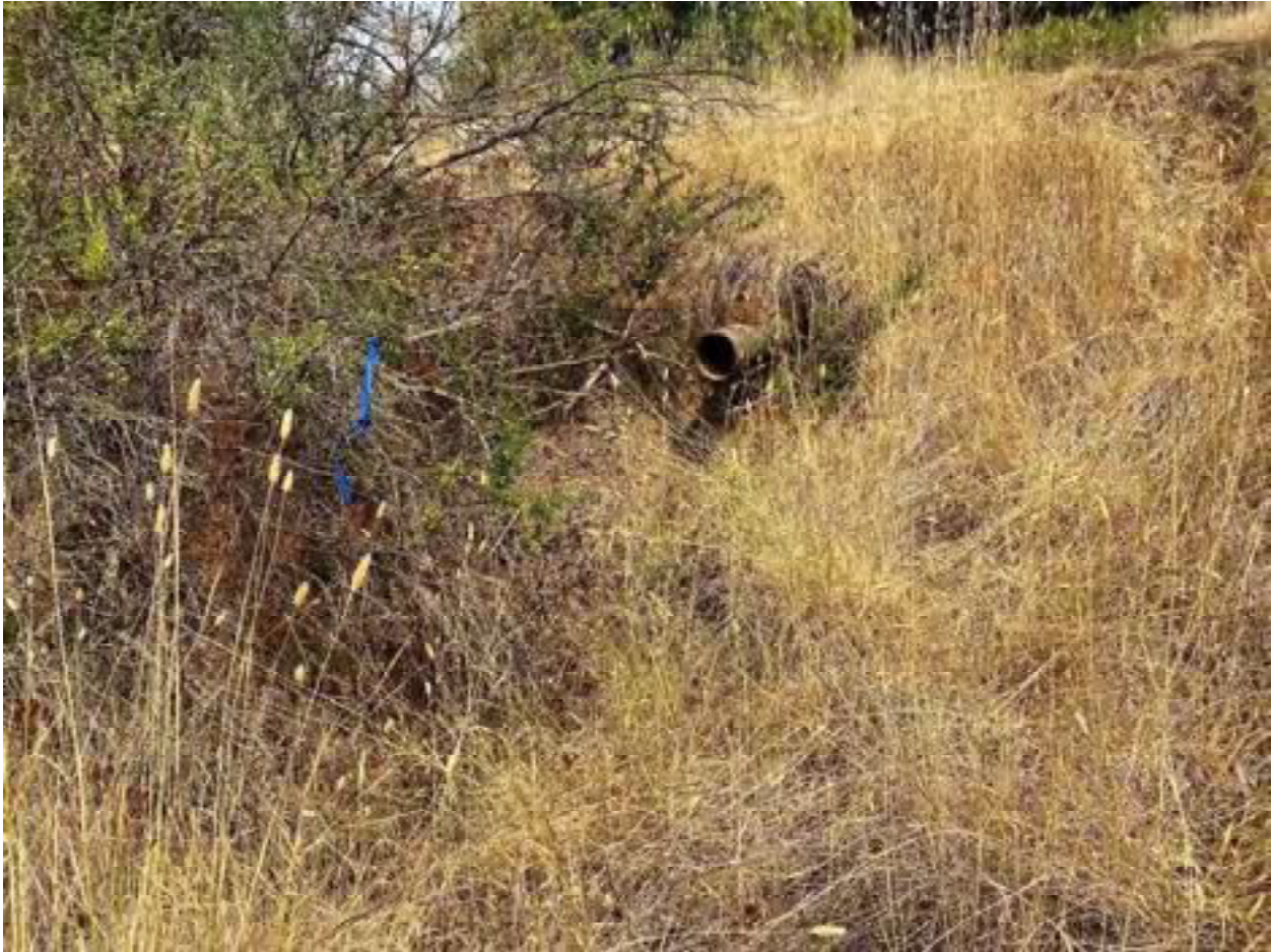
Photo 14: Stream Crossing 04. Looking upstream towards the outlet of the 8-inch diameter culvert at stream crossing 04. Photo date 9-1-2021.
