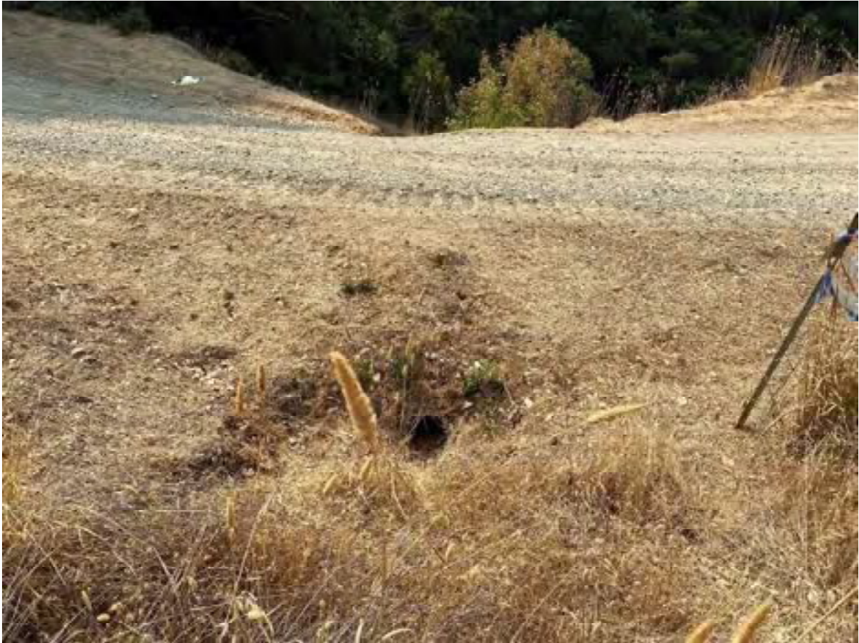
Photo 6: Stream Crossing 03. Looking downstream towards the inlet of the 8-inch diameter culvert at stream crossing 03. Photo date 9-1-2021.
