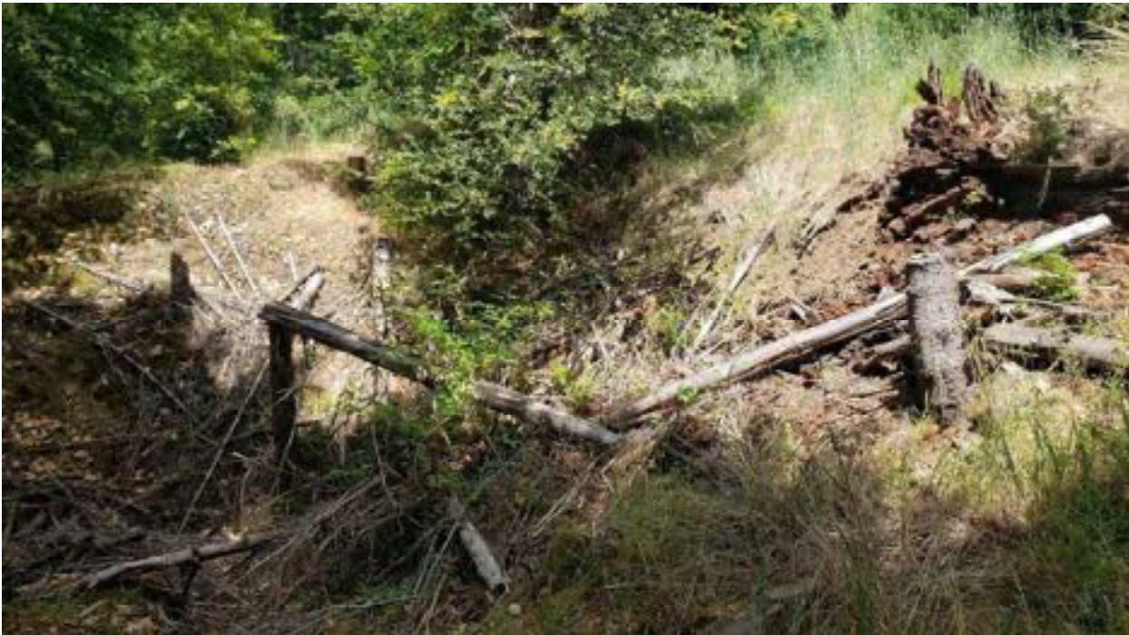
Site 19. Photo of the southeastern embankment of G5/G6/G, immediately down stream of the outlet of the watercourse crossing at Site 19. Note vegetation and rotted tree in the upper right. Indicative that this location has been in this condition for many years and was not recently created.
