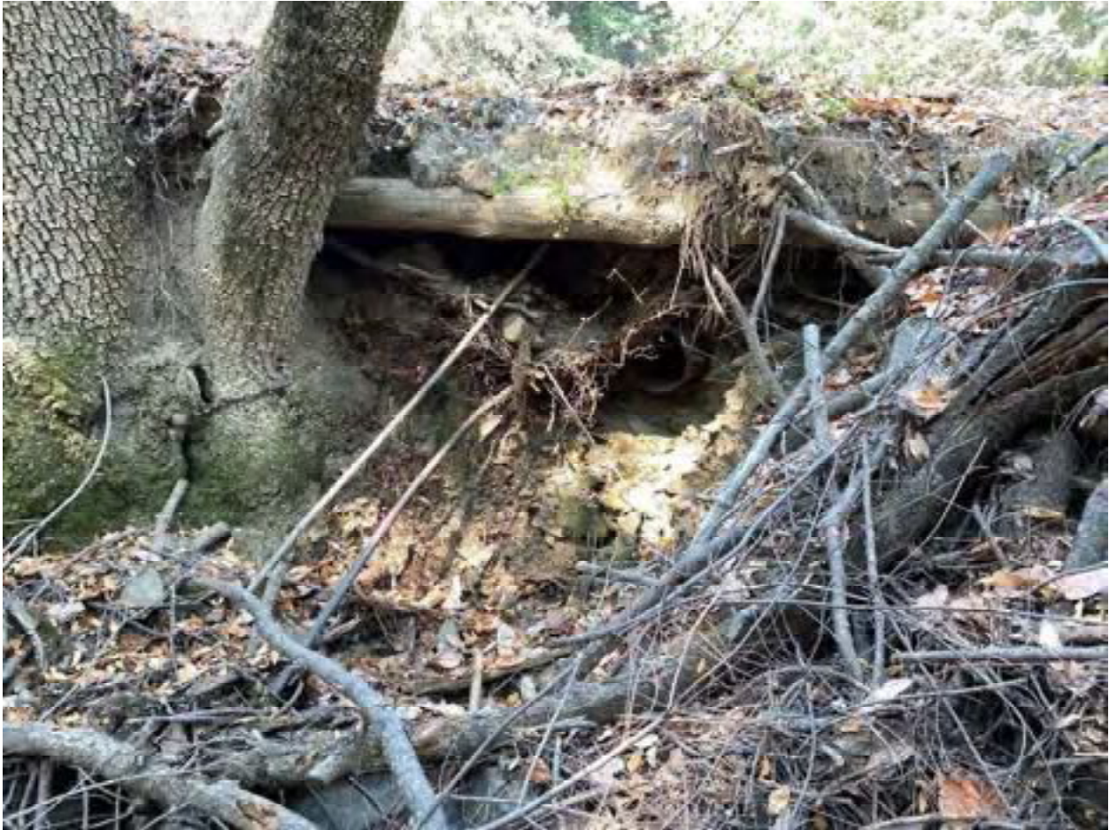
Photo 28: Stream Crossing 07. Looking upstream towards the outlet of the 12-inch diameter culvert at stream crossing 07. Photo date 9-1-2021.
