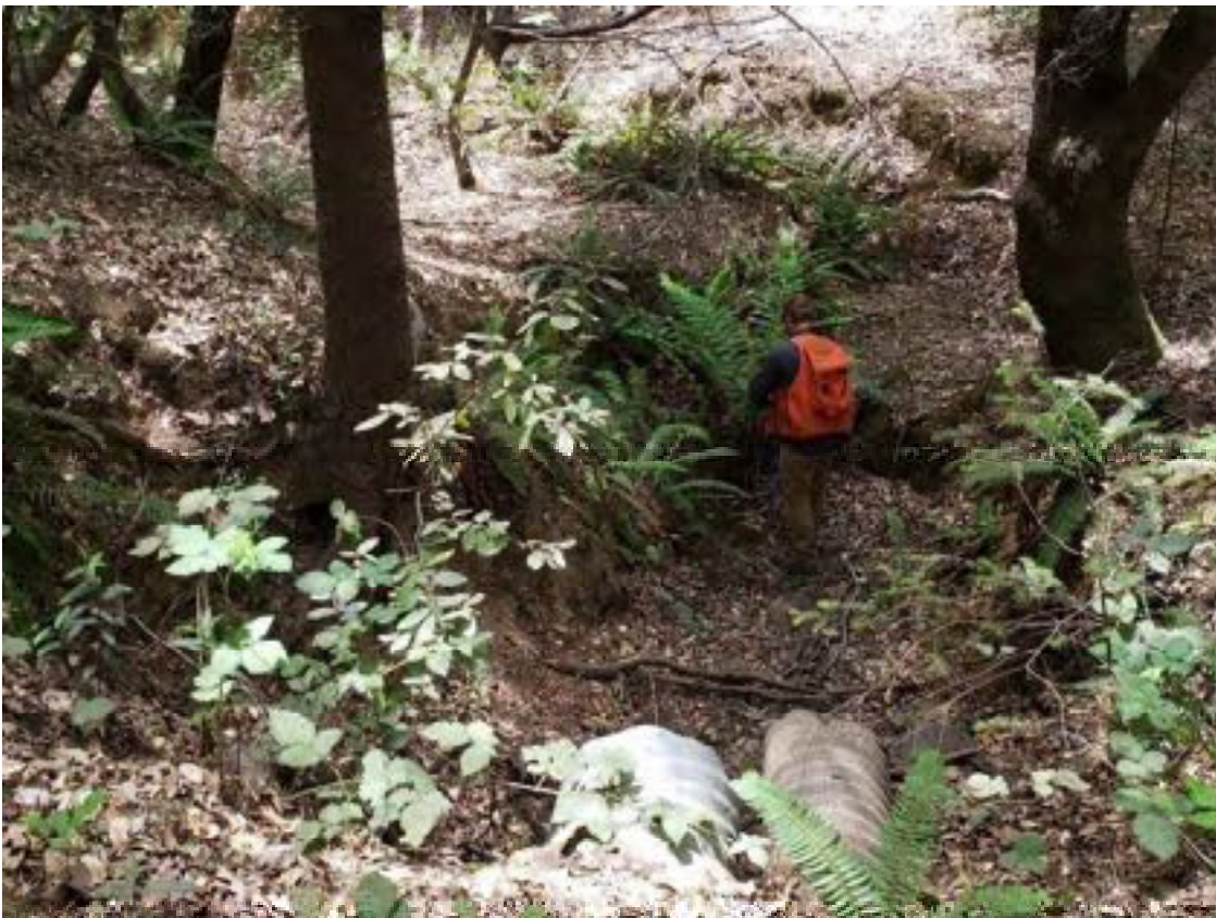
Site 23. Looking down channel from the outlet. The upgraded culvert will outlet approximately where the blue flag is being hanged.
