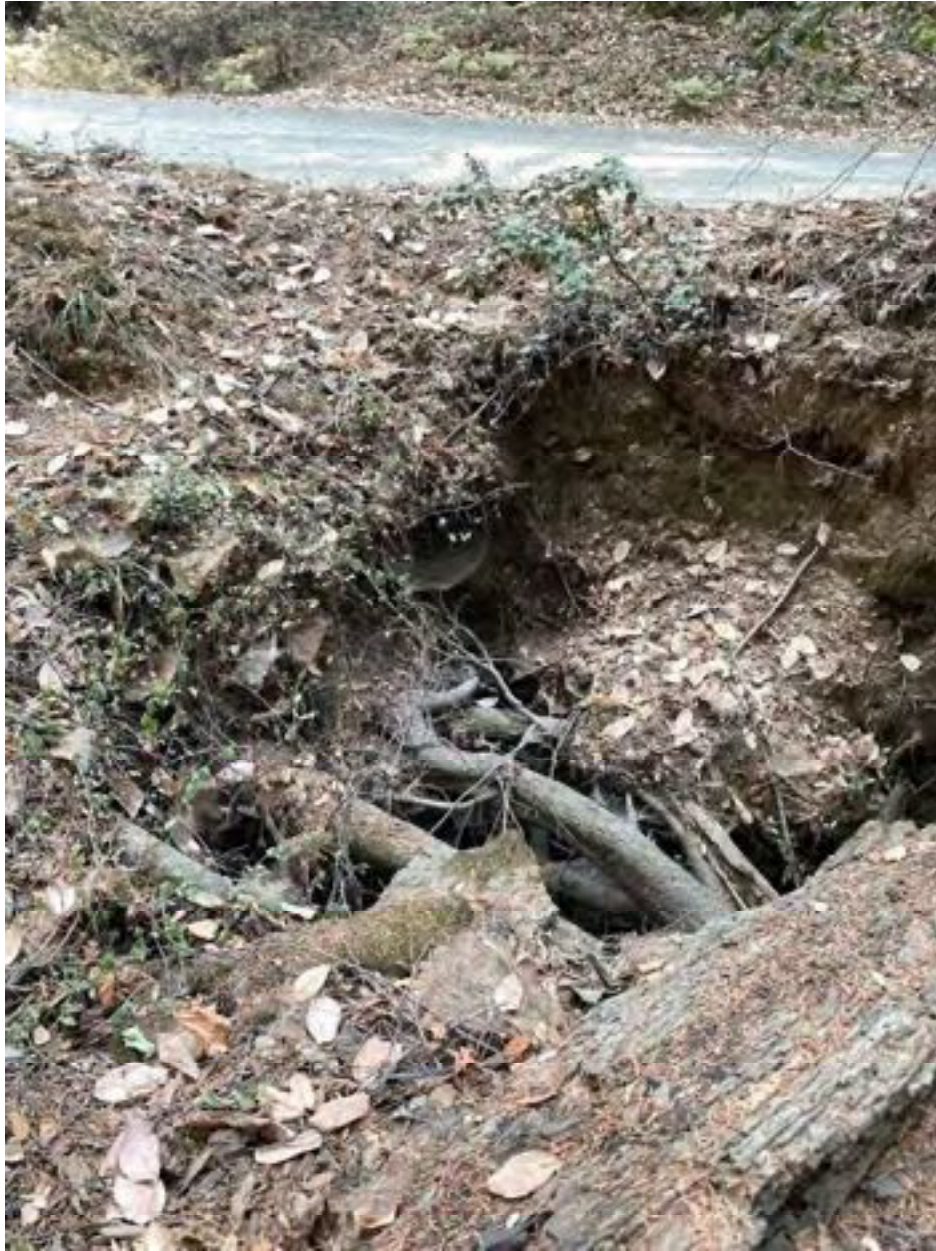
Photo 66: Stream Crossing 24. Looking upstream towards the outlet of the 18-inch diameter culvert at stream crossing 24. Photo date 9-1-2021.
