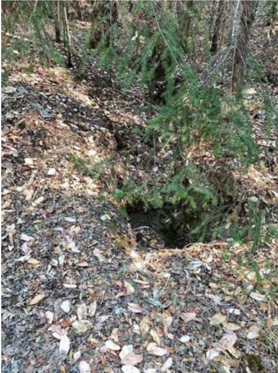
Photo 51: Stream Crossing 17. Looking downstream from the outlet of the 18-inch diameter culvert at stream crossing 17 that is proposed for removal. Photo date 9-1-2021.
