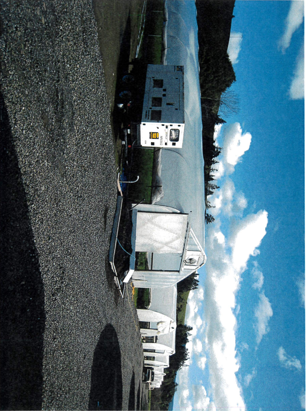
2 and 4 and Generator
