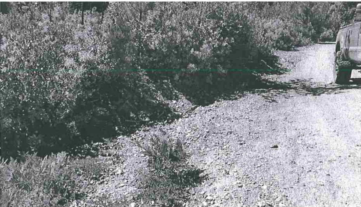
Road Point 3(top) & Road Point 4(bottom): A water bar has been installed in these two locations to direct road runoff. Owner will monitor and maintain the water bars so that road runoff is adequately diverted. 7/12/2016
