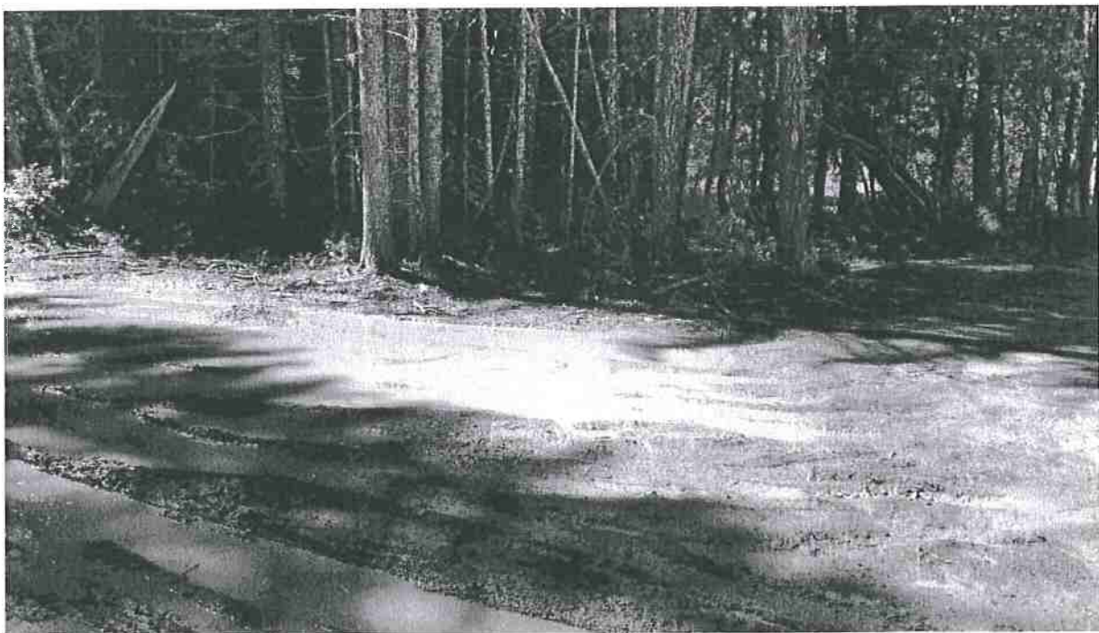
Road Point 1: Poor road drainage resulting in pooling of water on the road way. The area will be rocked and a drainage trench will be installed to collect and drain waters into the forest and duff. Photo date 7/12/2016
