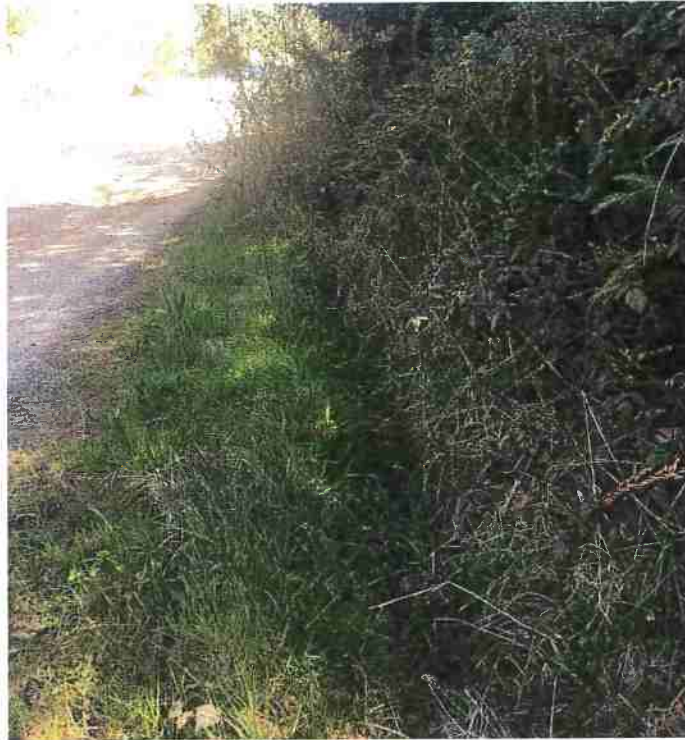
Figure 9: RP5. Inlet of 12' ditch relief culvert. Image shown facing east; away from Dows Prairie Rd.
