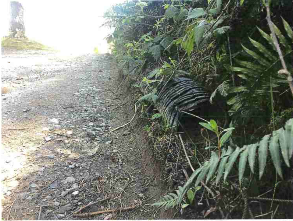
Figure 5: RP3. 16' graveled road width; Inboard ditch with failing culvert and location of lead-out ditch. Image shown facing east.
