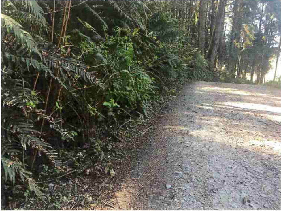
Figure 7: RP4. Outlet of 12' ditch relief culvert. Image shown facing east; away from Dows Prairie Rd.
