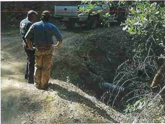
Figure 14. This fill slope erosion was caused by a plugged cross-drain inlet that diverted ditch flow over the road surface. Photo: Angela Wilson, Central Valley Regional Water Quality Control Board.
