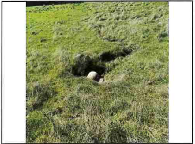
Photo #234 Blue Rock Rd Looking @ 18" Partially Clogged Culvert Out
