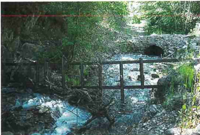
Figure 24. A trash rack installed upstream to protect a culvert from plugging. Source: Keller and Sherar 2003.
