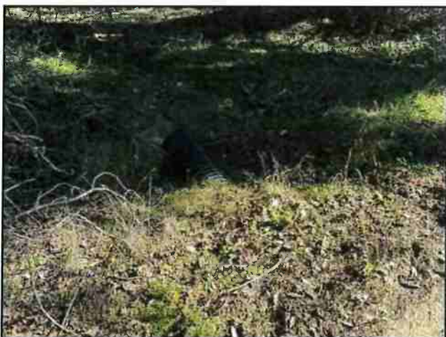
Photo #161 Blue Rock Rd 18" Culvert Out
