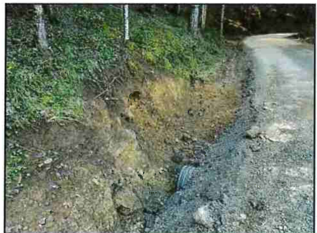
Photo #186 Blue Rock Rd Looking@ 18" Culvert In Causing Sediment Transport
