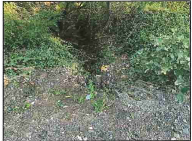
Photo #130 Blue Rock Rd Looking @ Short/ Clogged Culvcert Out Size Unknown
