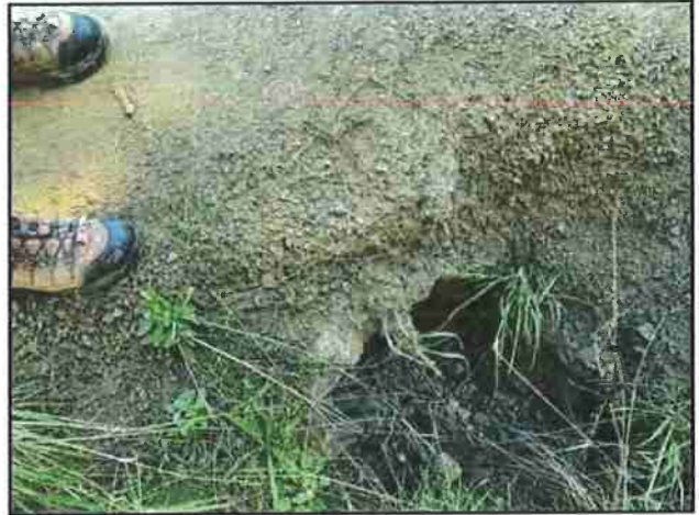
Photo #116 Blue Rock Rd Looking@ Partially Crushed/Short 12" Culvert In
