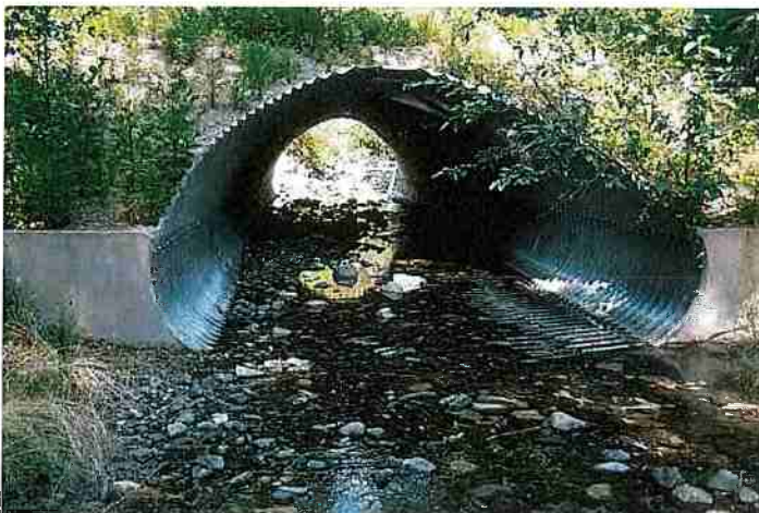
Figure 28. An arched pipe installed on a fish-bearing stream to minimize impacts on fish habitat and migration. Source: Keller and Sherar 2003.
