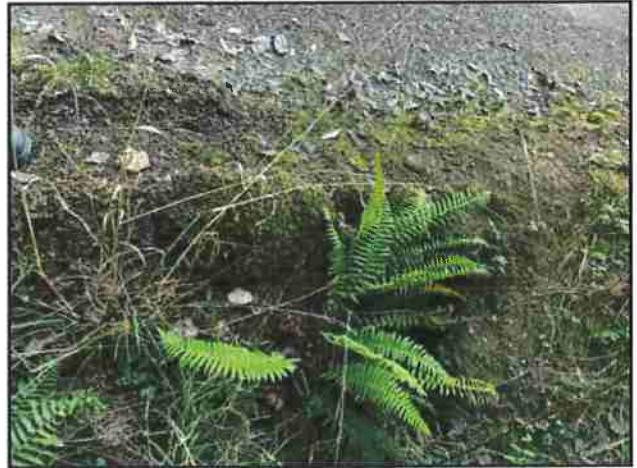
Photo #142 Blue Rock Rd Looking@ Partially Clogged/Short Culvert In Size Unkown
