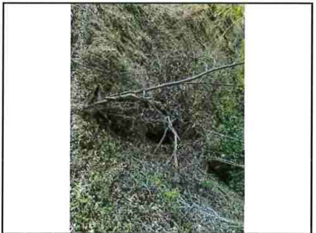
Photo #42 APN #223-034-005 Private Access Rd Looking@ Partially Clogged 12" Culvert In
