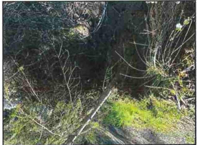
Photo #118 Blue Rock Rd Looking@ Partially Crushed/Short 12" Culvert Out
