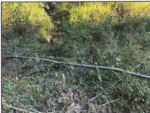
Photo #143 Blue Rock Rd Looking @ Partially Clogged Culvert In Size Unkown
