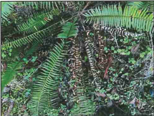
Photo #129 Blue Rock Rd Looking@ Clogged Culvert In Size Unknown
