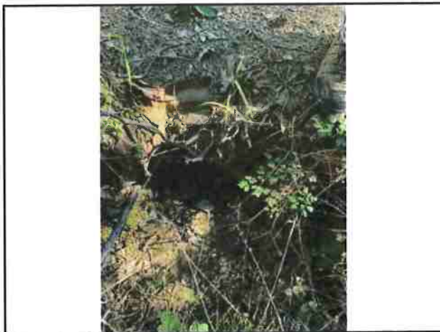
Photo #167 Blue Rock Rd Looking@ Short/Partially Clogged 12" Culvert In
