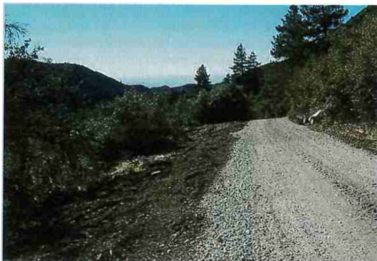
Figure 1. Low-volume road that has been newly graded and out-sloped, San Bernardino County. Photo: Richard Harris.
