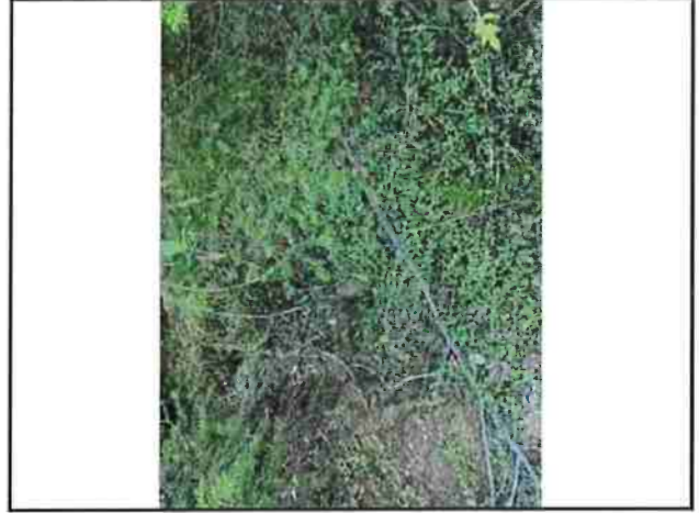
Photo #14 APN #223-034-005 Private Access Rd Looking@ Clogged 12" Culvert Out
