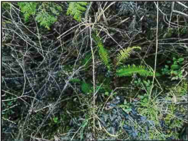
Photo #99 Blue Rock Rd Looking @ Clogged Culvert In Size Unknown
