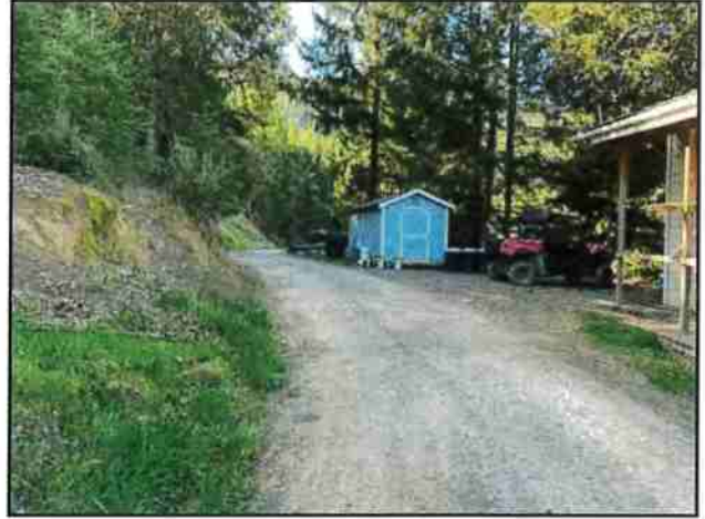
Photo #26 APN #223-034-005 Private Access Rd Looking@ Clogged Culvert In Out Not Found
