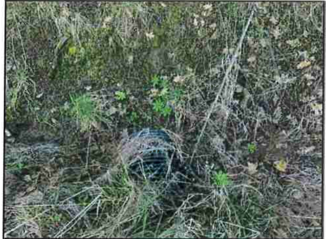
Photo #194 Blue Rock Rd Looking@ Partially Clogged 18" Culvert In
