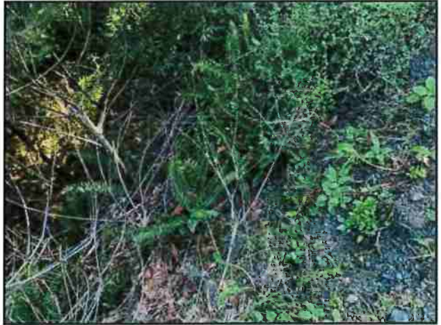
Photo #100 Blue Rock Rd Looking @ Clogged Culvert Out Size Unknown
