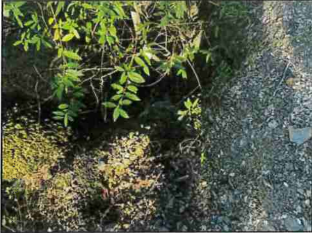
Photo #49 APN #223-034-005 Private Access Rd Looking@ Partially Clogged 12" Culvert Out
