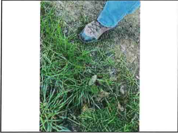
Photo #25 APN #223-034-005 Private Access Rd Looking@ Clogged Culvert In Out Not Found
