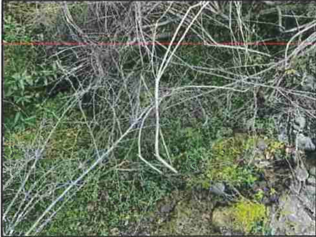
Photo #7 APN #223-034-005 Private Access Rd Looking@ Clogged Culvert In Out Not Found
