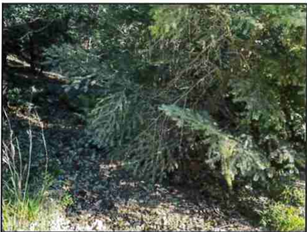
Photo #173 Blue Rock Rd Looking @ Partially Clogged 12" Culvert Out.
