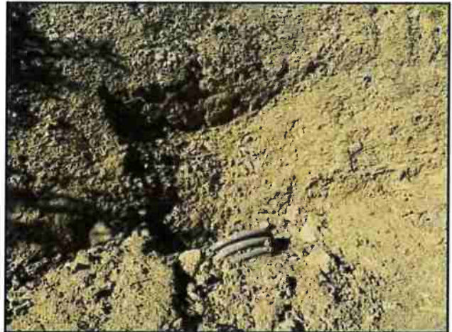
Photo #172 Blue Rock Rd Looking @ 12" Culvert w/ Exposed Sediment Transport
