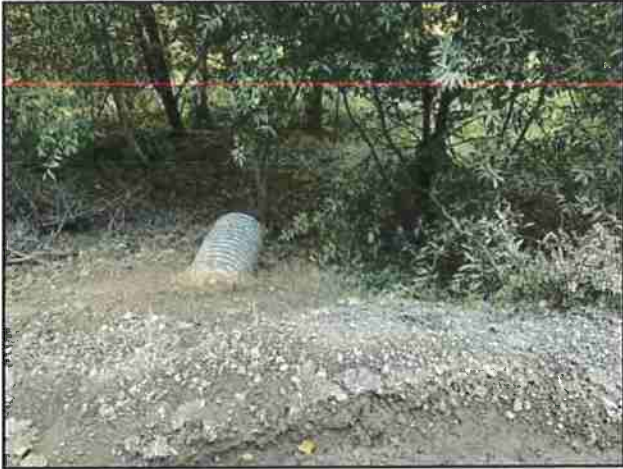
Photo #187 Blue Rock Rd Looking@ 18" Culvert Out Causing Sediment Transport
