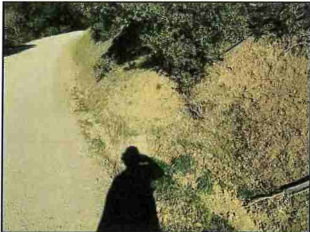
Photo #255 Blue Rock Rd Looking @ Partially Clogged 18" Culvert In
