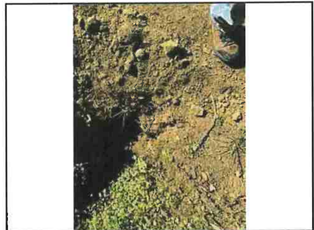
Photo #168 Blue Rock Rd Looking@ Short/Partially Clogged 12" Culvert Out
