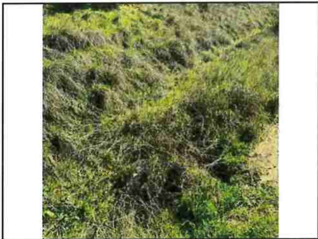
Photo #233 Blue Rock Rd Looking @ 18" Partially Clogged Culvert In
