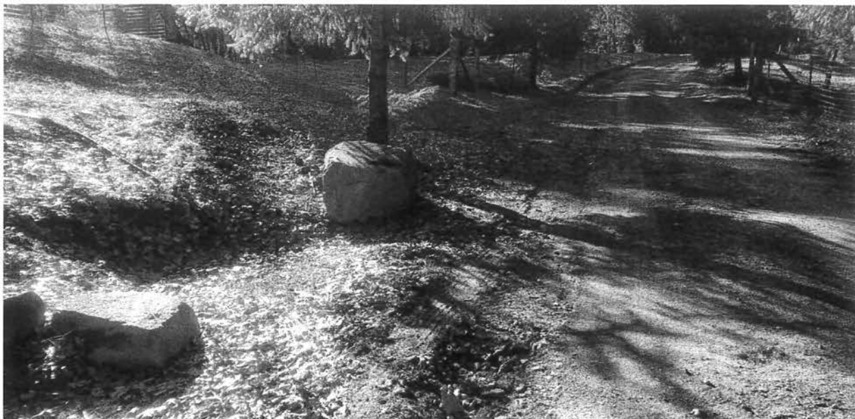
Photo looking at the inlet of the plugged ditch relief culvert at Site 02.
