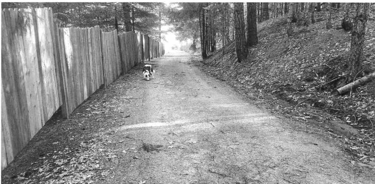
Photo looking down grade at Site 04. The ditch flows are jumping out of the inside ditch at this location.
