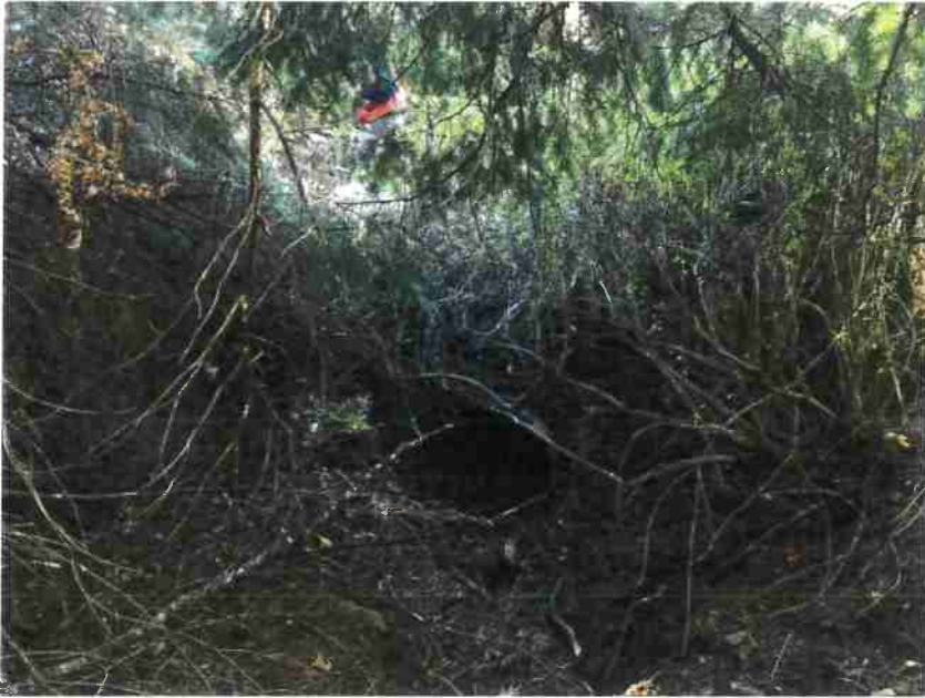
Photo 9, MP#6 – SC#4 , view of rusted 24-inch diameter culvert inlet on a Class III stream (Photo November 2018).
