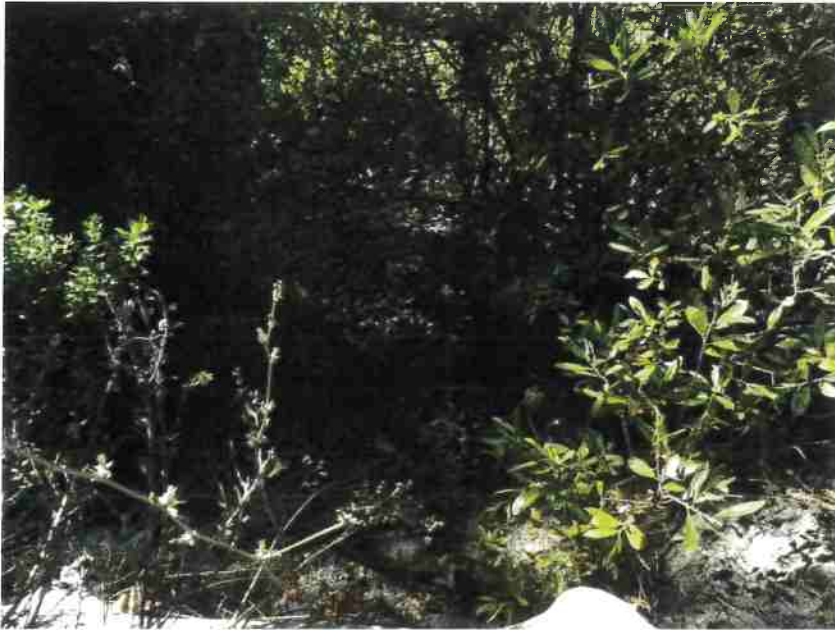
Photo 19, MP#12 – SC#10 , rusted 18-in culvert on a Class III stream, placed high in the fill, view looking downstream from road toward outlet (Photo September 2016).
