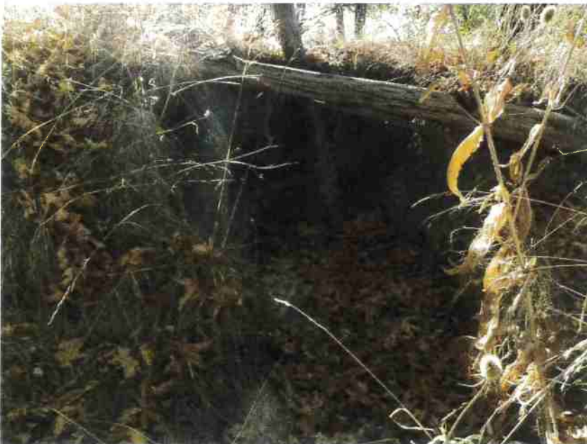
Photo 22, MP#14 – SC#12 , rusted 12-inch culvert on a Class III stream, view looking downstream at inlet (Photo September 2016).
