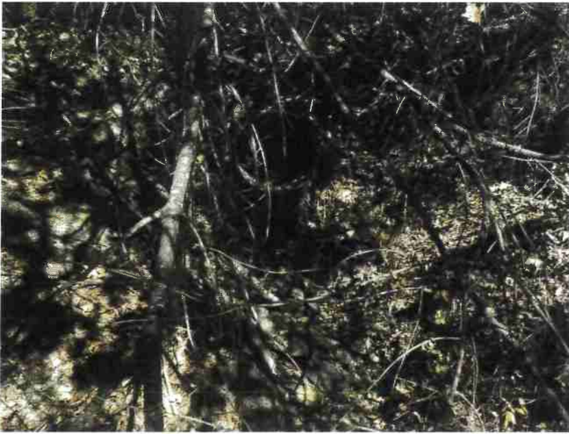
Photo 11, MP#7 – SC#5 , rusted through 12-inch diameter culvert on a near origin Class III stream placed high in the fill, view looking downstream at outlet (Photo September 2016).
