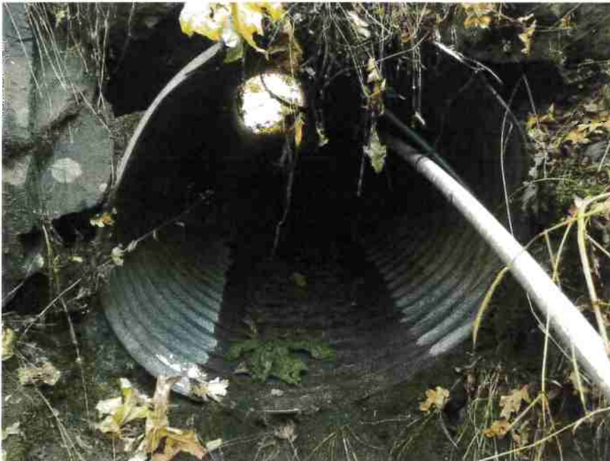
Photo 4, MP#3 – SC #1, rusted 36-inch diameter culvert on a near origin Class III stream, view looking upstream at outlet (Photo September 2016).
