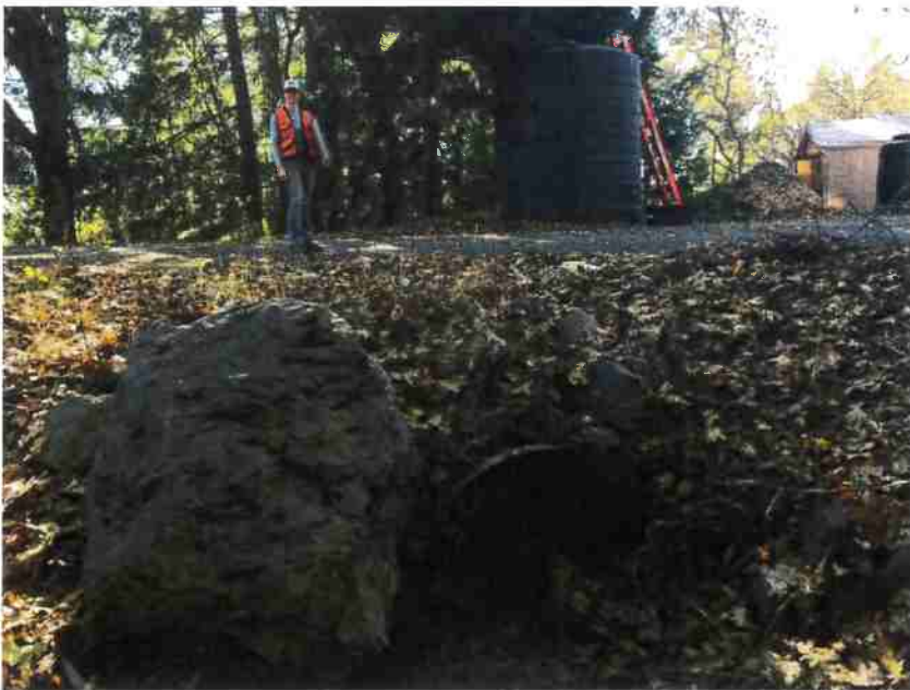
Photo 12, MP#8 – SC#6 , rusted 36-inch culvert on a Class III stream, placed high in the fill, view looking downstream at inlet (Photo November 2018).
