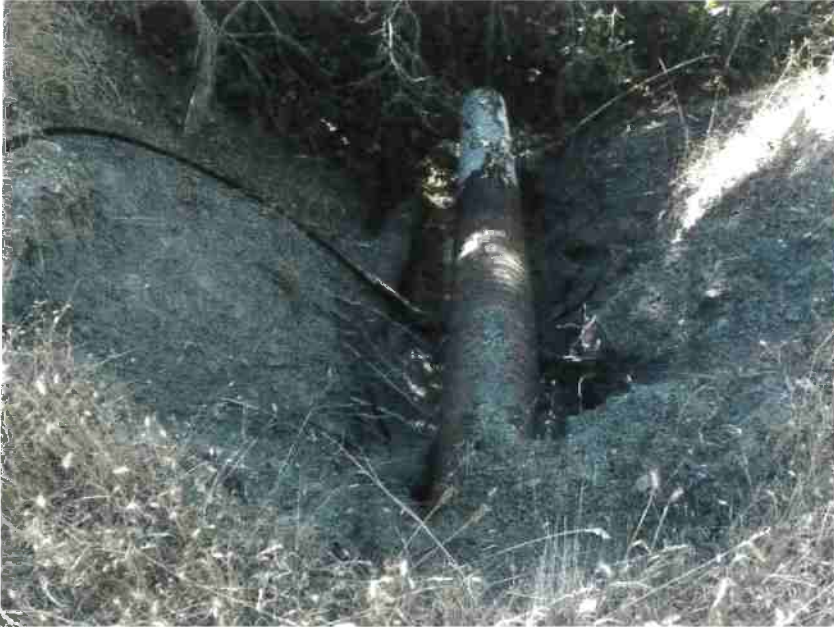
Photo 15, MP#10 – SC#8 , view of two culverts (18-inch dia. and 15-inch dia.) on a Class III stream, placed high in the fill, view looking downstream at the culvert outlets (Photo September 2016).
