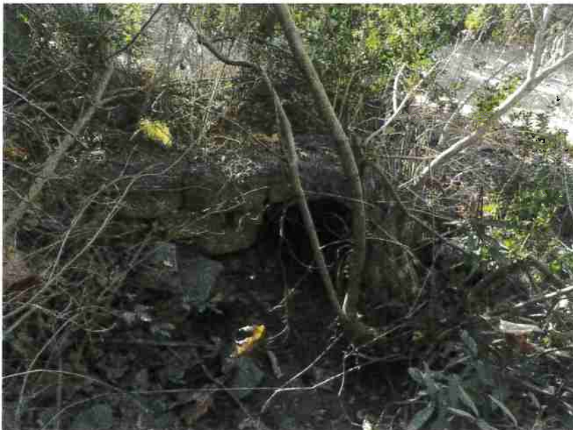
Photo 20, MP#13 – SC#11 , rusted 18-in culvert on a steep and rocky Class III stream, placed high in the fill, view looking downstream at inlet (Photo September 2016).
