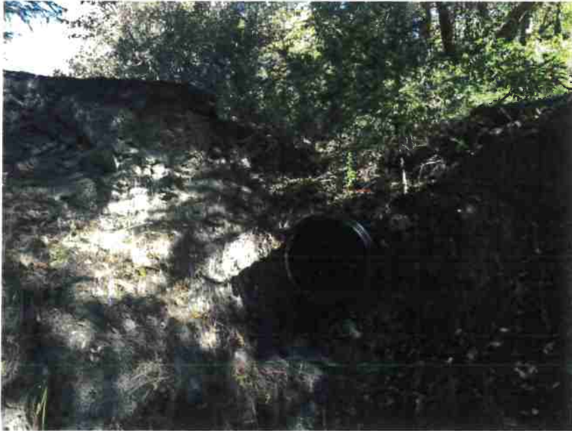
Photo 17, MP#11 – SC#9 , 24-inch plastic culvert on a Class III stream, placed high in the fill, view looking upstream at outlet (Photo November 2018).
