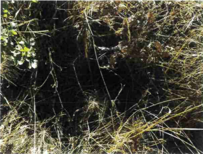
Photo 1, MP #1 – DRC#1, 12-inch diameter ditch relief culvert, view looking downslope at inlet (Photo September 2016).
