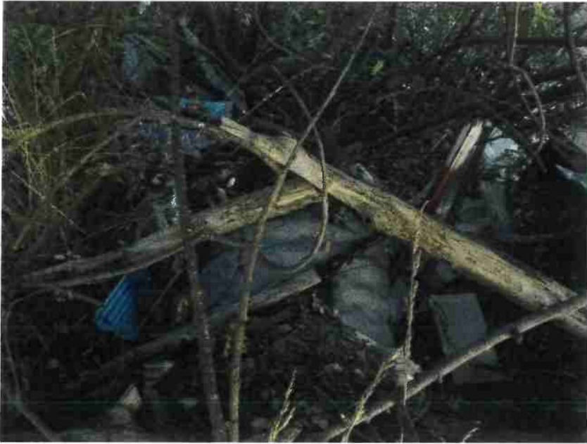
Photo 21, MP#13 – SC#11 , rusted 18-in culvert on a steep and rocky Class III stream, placed high in the fill, view looking downstream at outlet and trash in the channel (Photo September 2016).
