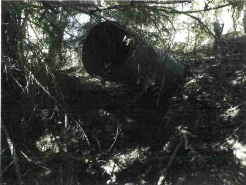
Photo 13, MP#8 – SC#6 , rusted 36-inch culvert on a Class III stream, placed high in the fill above 2 older buried culverts, view looking upstream at outlet (Photo September 2016).
