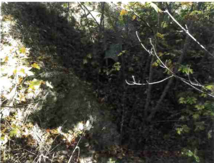
Photo 2, MP #2 – DRC#4, 18-inch diameter ditch relief culvert, view looking upslope at outlet (Photo September 2016).
