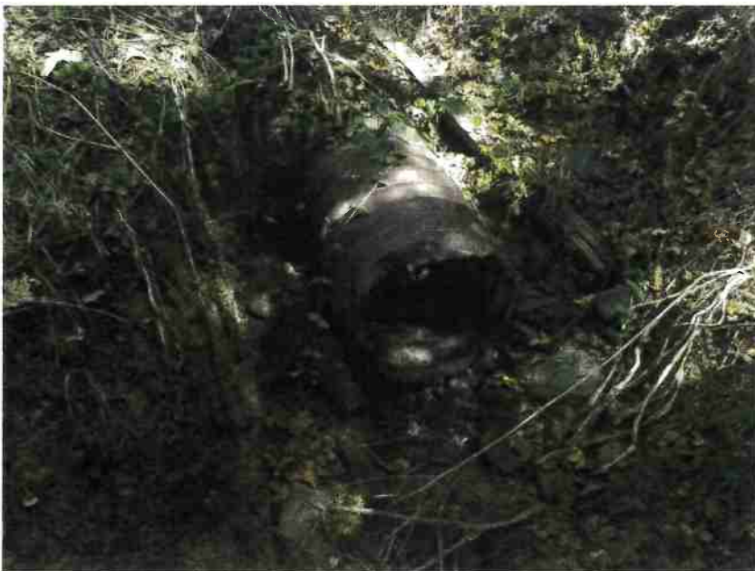
Photo 6, MP#4 – SC#2 , rusted through 15-inch diameter culvert on a near origin Class III stream, view looking upstream at outlet (Photo September 2016).
