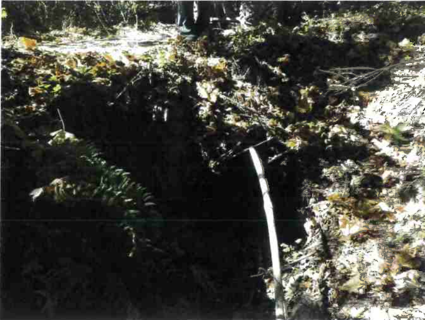
Photo 3, MP#3 – Stream Crossing (SC) #1, rusted through 36-inch diameter culvert on a near origin Class III stream, view looking downstream at inlet (Photo September 2016).
