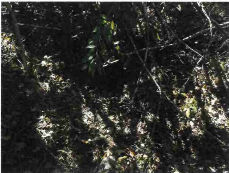
Photo 10, MP#7 – SC#5 , rusted 12-inch diameter culvert on a near origin Class III stream, view looking downstream at inlet (Photo September 2016).
