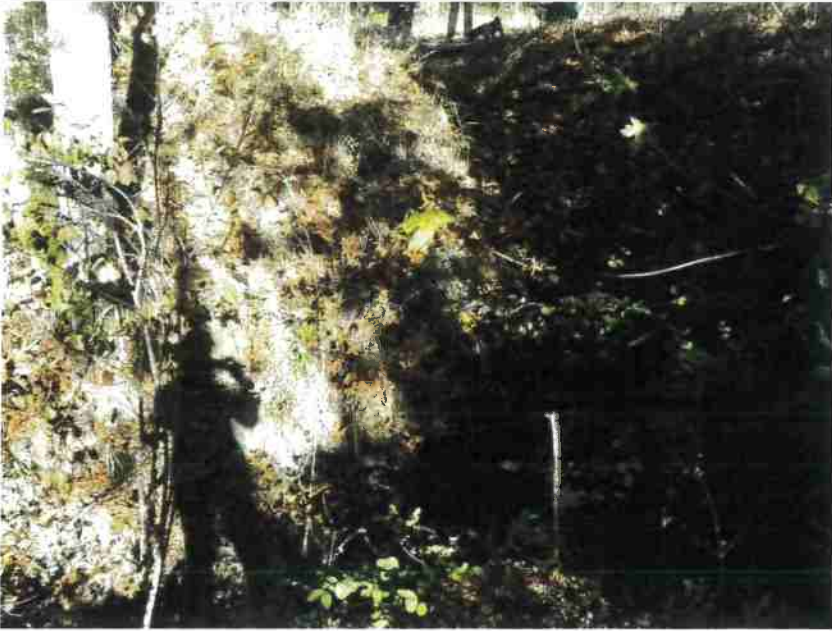
Photo 23, MP#14 – SC#12 , rusted 12-inch culvert on a Class III stream, view looking upstream at inlet (Photo September 2016).
