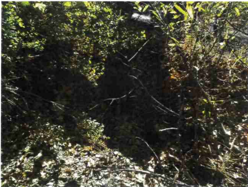
Photo 18, MP#12 – SC#10 , rusted 18-in culvert on a Class III stream, placed high in the fill, view looking downstream at plugged inlet (Photo September 2016).
