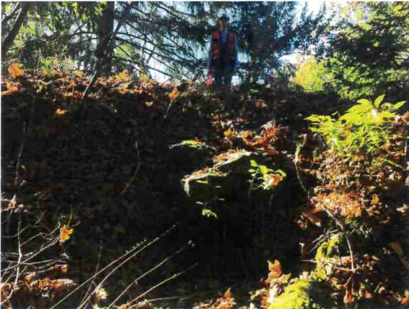
Photo 16, MP#11 – SC#9 , 24-inch plastic culvert on a Class III stream, placed high in the fill, view looking downstream at inlet (Photo September 2016).
