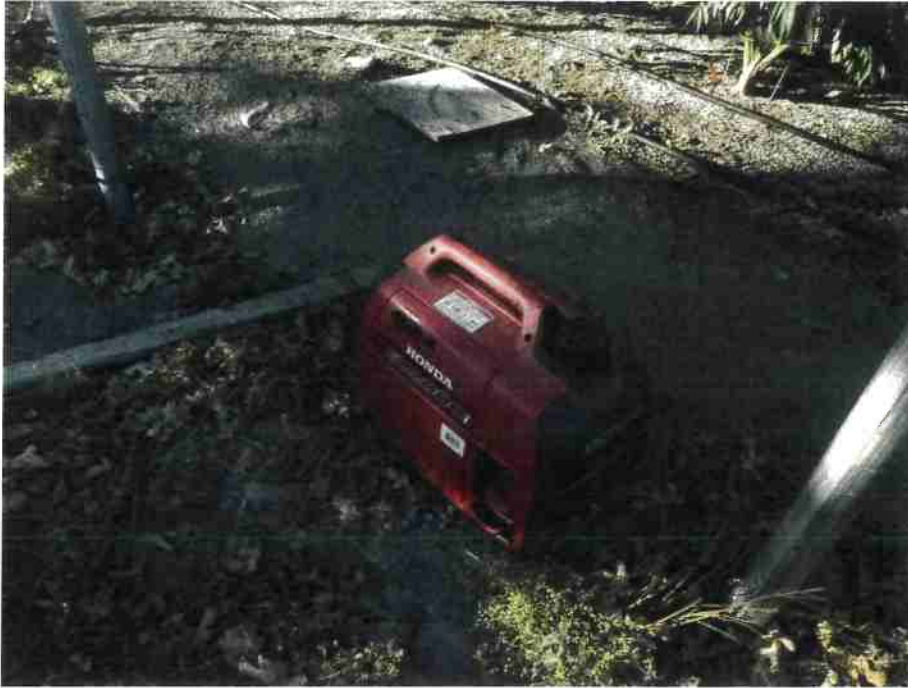
Photo 31, MP#25 – View of gas powered generator near CA#7 (Photo September 2016).
