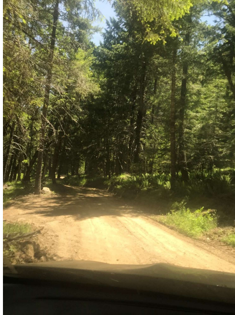
Figure 10: Image #6965. Typical section of road segment 13. Note pinch point ahead with turnout areas to the left and right on approach.
