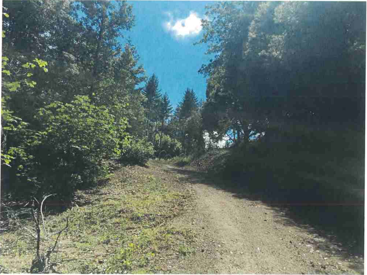
Photo 5. Access road between Conversion Area #1 and #2. A rolling dip on this road segment will improve drainage.
