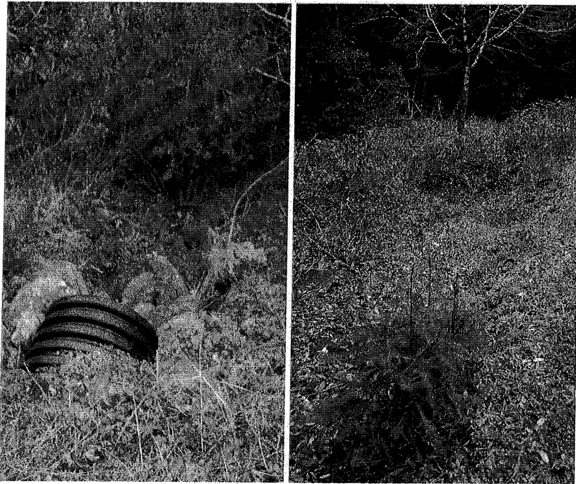
Pictures 2 and 3: The picture on the left is the culvert inlet at Map Point 01. The picture on the right is the broad, inside ditch that contains the Class III flow for approximately 60 feet prior to reaching the inlet. Photo date 2/26/2016
