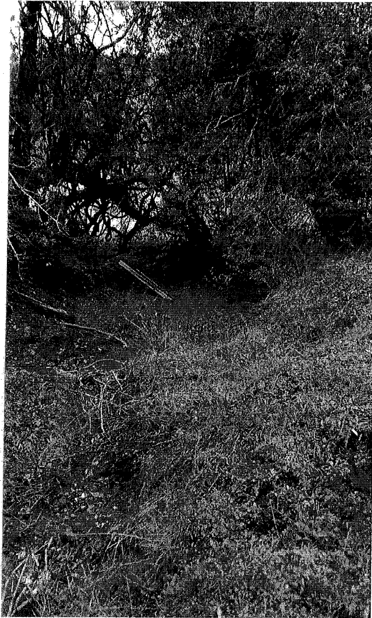
Picture 5: This is a picture looking down stream of the outlet of the 24 inch culvert at Map Point 01. Sediment deposited from high Mattole River flows can be seen at the far end of the picture. The light area beyond the tree cover is the Mattole River. Photo date 2/26/2016
