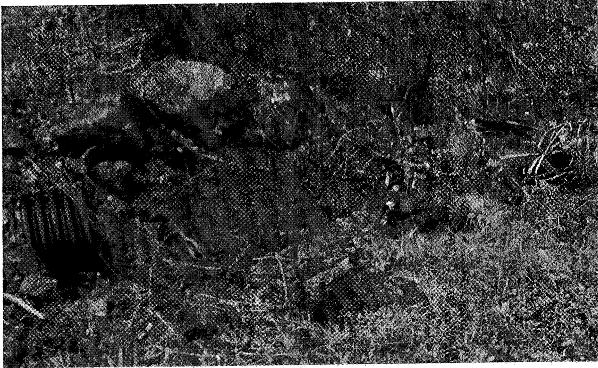
Picture 4: This is a picture of the outlet of the 24 inch culvert at Map Point 01. Photo date 2/26/2016
