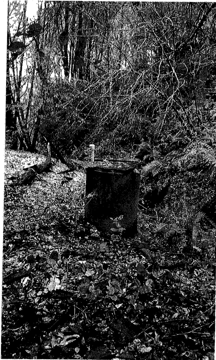
Picture 13: This is a picture of the shallow well structure located next to the watercourse near the present point of diversion. It is old and is not connected or being used currently. Photo date 2/26/16.
