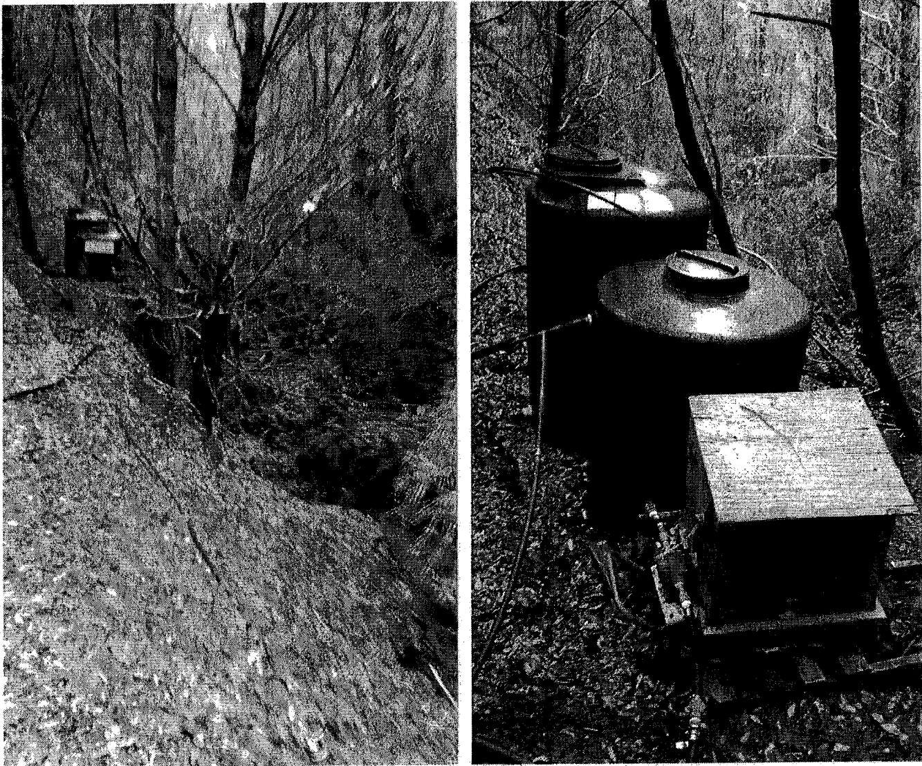
Picture 14 and 15: The picture on the left shows the holding tanks and gas-powered water pump situated on the overhanging bank above the Class II Watercourse. The picture on the right is a close up of the holding tanks and the water pump. Photo date 2/26/16.
