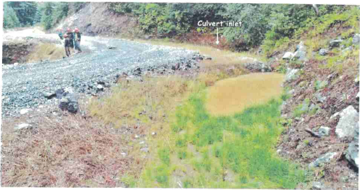
FIGURE 238. Traffic and surface runoff from graveled roads often produces surface erosion, turbid runoff and fine sediment transport that can be delivered to streams. Where ditches can't be eliminated, sediment traps and roadside settling basins can be installed to capture and remove most of the eroded sediment. This settling basin has been constructed along the inside ditch just before a stream crossing culvert inlet (see arrow). Eroded sediment from the road and ditch are deposited in the basin before flow is released to the stream. Fine sediments have filled about 1/3 of this basin and vegetation is now growing. Sediment basins require periodic maintenance to maintain their storage capacity.
