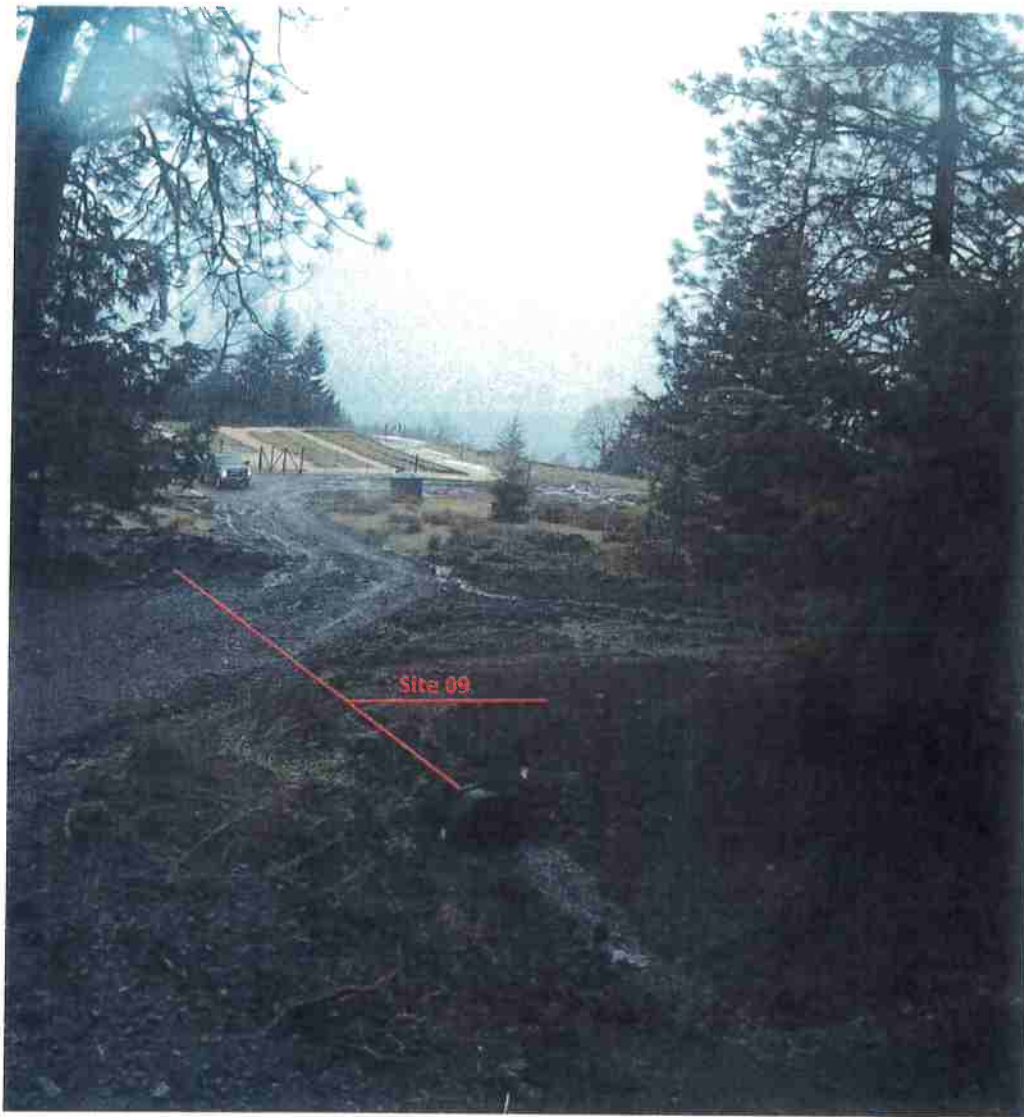
This photograph references Site 09 a 24" ditch relief culvert. Cultivation Area A is in the background.
