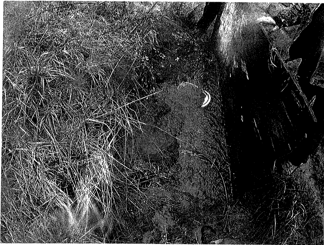
Point of diversion. 5 gallon bucket burried with a 1" poly line gravity fed to holding tank. Utilized for domestic use.
