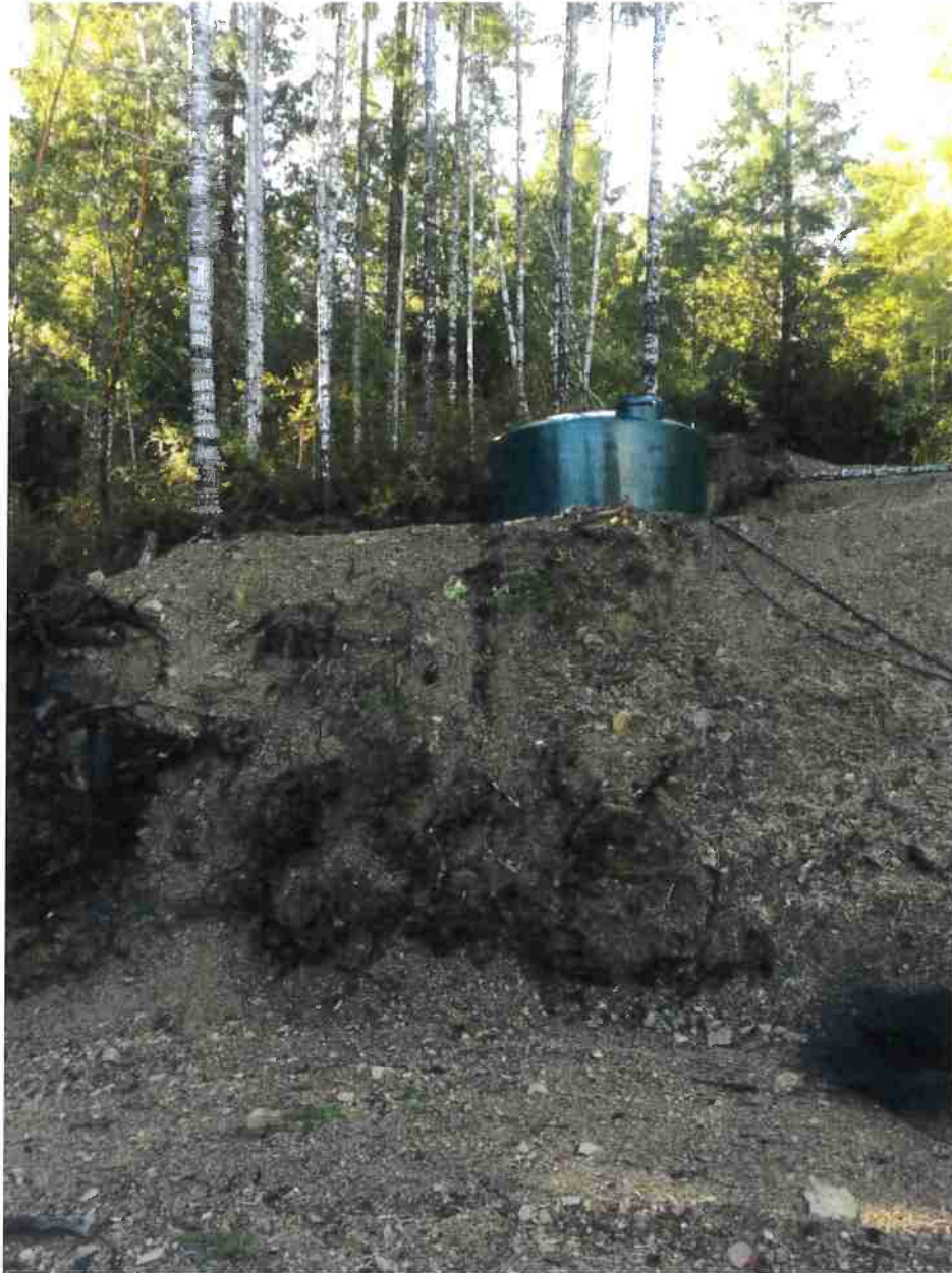
Photo 14: Erosion on fill slope of pad for 5,000 gallon water tank (Map Point F).
