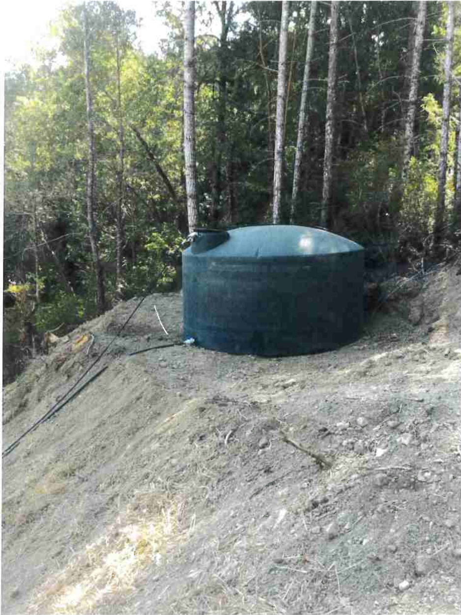
Photo 11: One 5,000 gallon poly storage tank. Photo date 9-8-16
