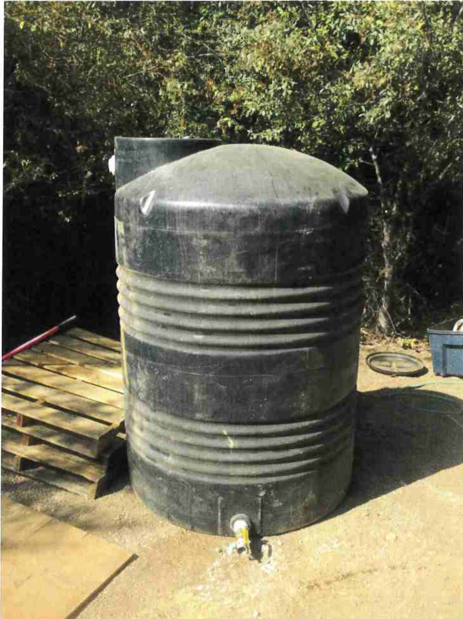
Photo 13: One 500 gallon mixing/feed tank. Photo date 9-8-16
