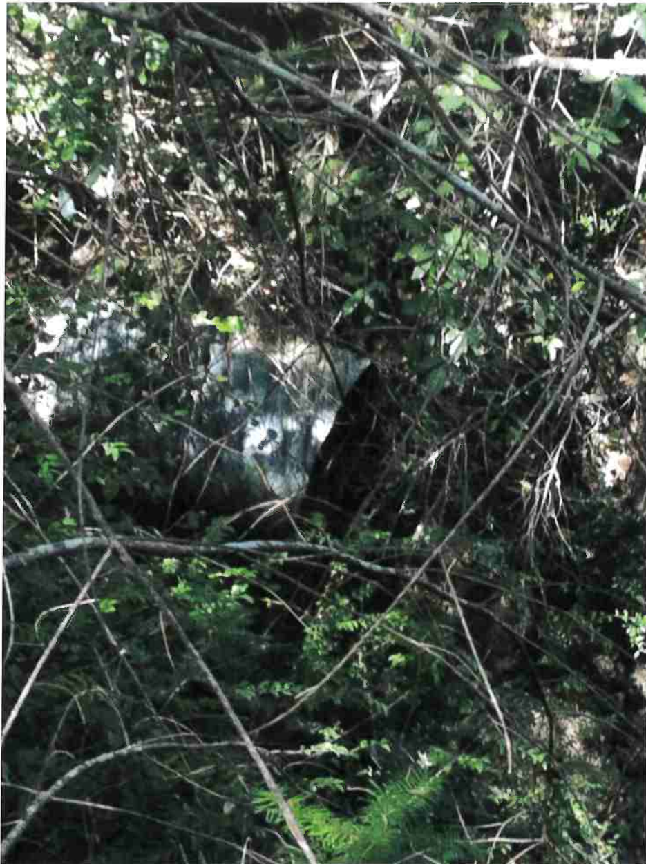
Photo 7: Crossing #1 outlet, requires energy dissipater (Map Point G). Photo date 9-8-16
