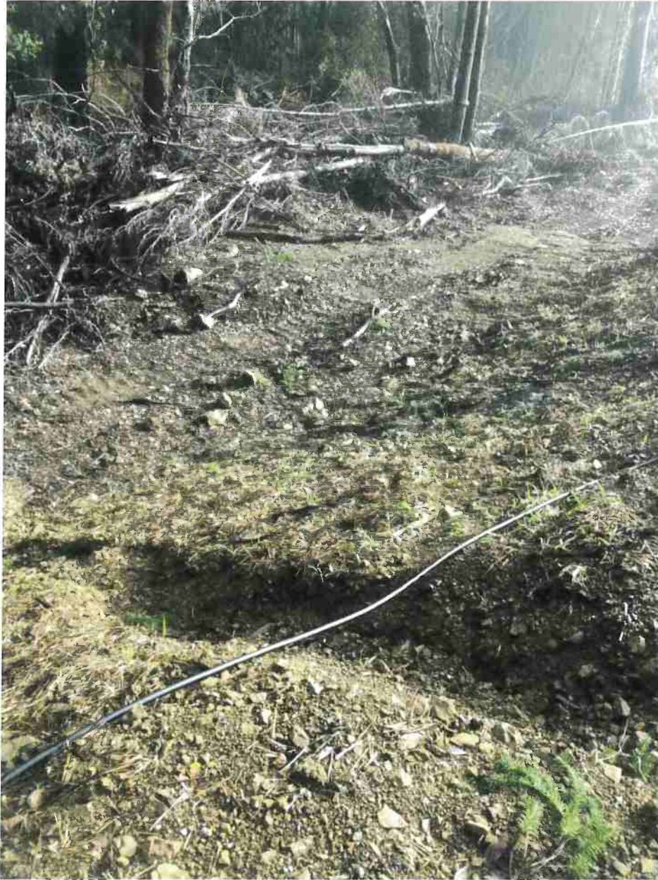
Photo 3: Erosion of fill slope of outdoor cultivation pad (Map Point C). Photo date 1-24-17
