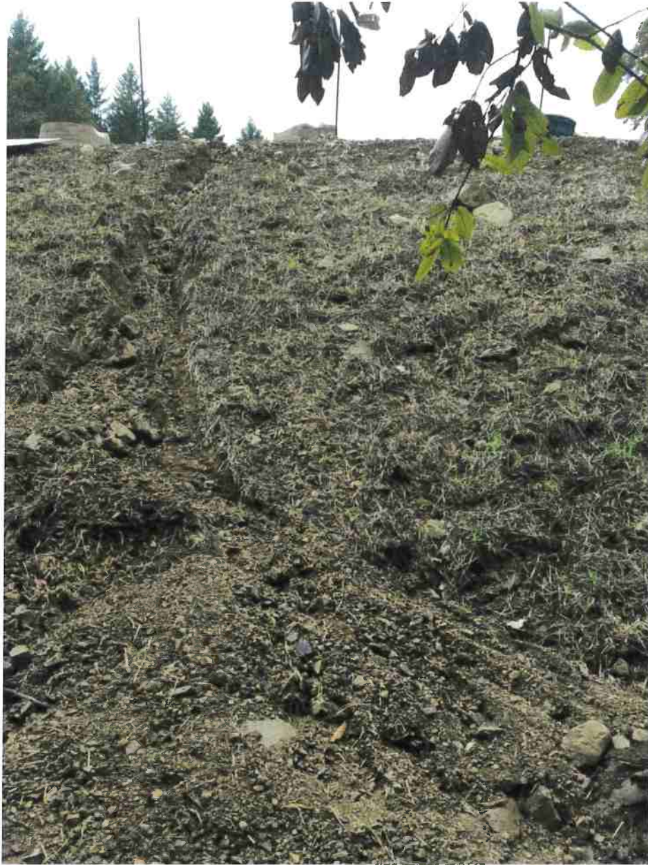
Photo 5: Erosion and transport of sediment from fill slope of outdoor cultivation pad (Map Point A). Photo date 11-11-16
