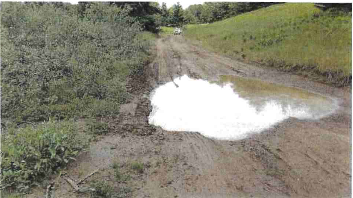
Road Point 3: Road runoff is bypassing a failing rolling dip, resulting in erosion of the surface of the road past the rolling dip and sediment discharge to a Class III watercourse. Install a rocked rolling dip per attached specifications and rock the surface of the road to Road Point 2. Install a shallow inside ditch leading up to Road Point 2 and slope the road into the inside ditch. Place rock and install wattles at the outflow of the rocked rolling dip.
