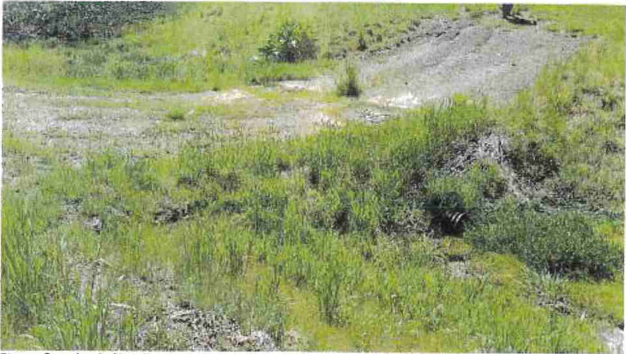
Stream Crossing 2: Class III watercourse crossing consisting of a 12-inch diameter plastic culvert on a seasonal access road. This crossing is significantly undersized and shall be upgraded to a minimum 30-inch diameter culvert installed per the attached specifications.
