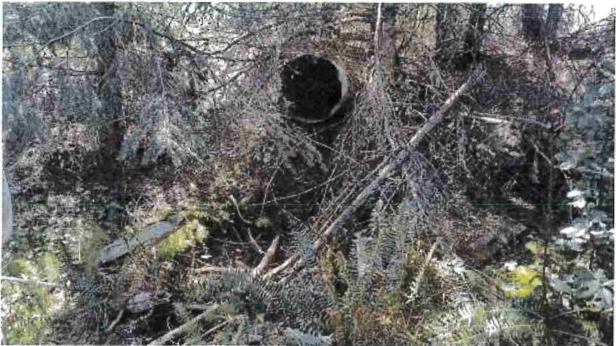
Stream Crossing 4/Lake Overflow: Class III watercourse crossing/lake overflow consisting of a 24-inch diameter steel culvert. The culvert is lacking an energy dissipater at the outflow. Install an energy dissipater at the outflow of the culvert.
