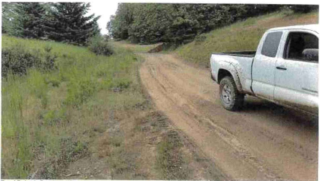
Road Point 2: Road runoff is bypassing a failing rolling dip, resulting in erosion past the rolling dip and sediment discharge to a Class III watercourse. Install a rocked rolling dip per attached specifications and rock the surface of the road. Place rock and install wattles at the outflow of the rocked rolling dip.
