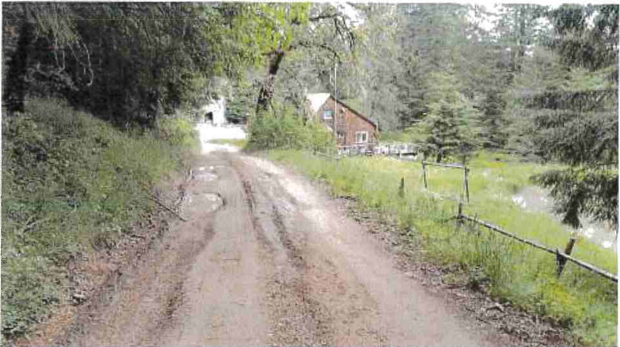
Road Point 5: Storm waters are not being drained off the surface of the road. Install a rolling dip per attached specifications.
