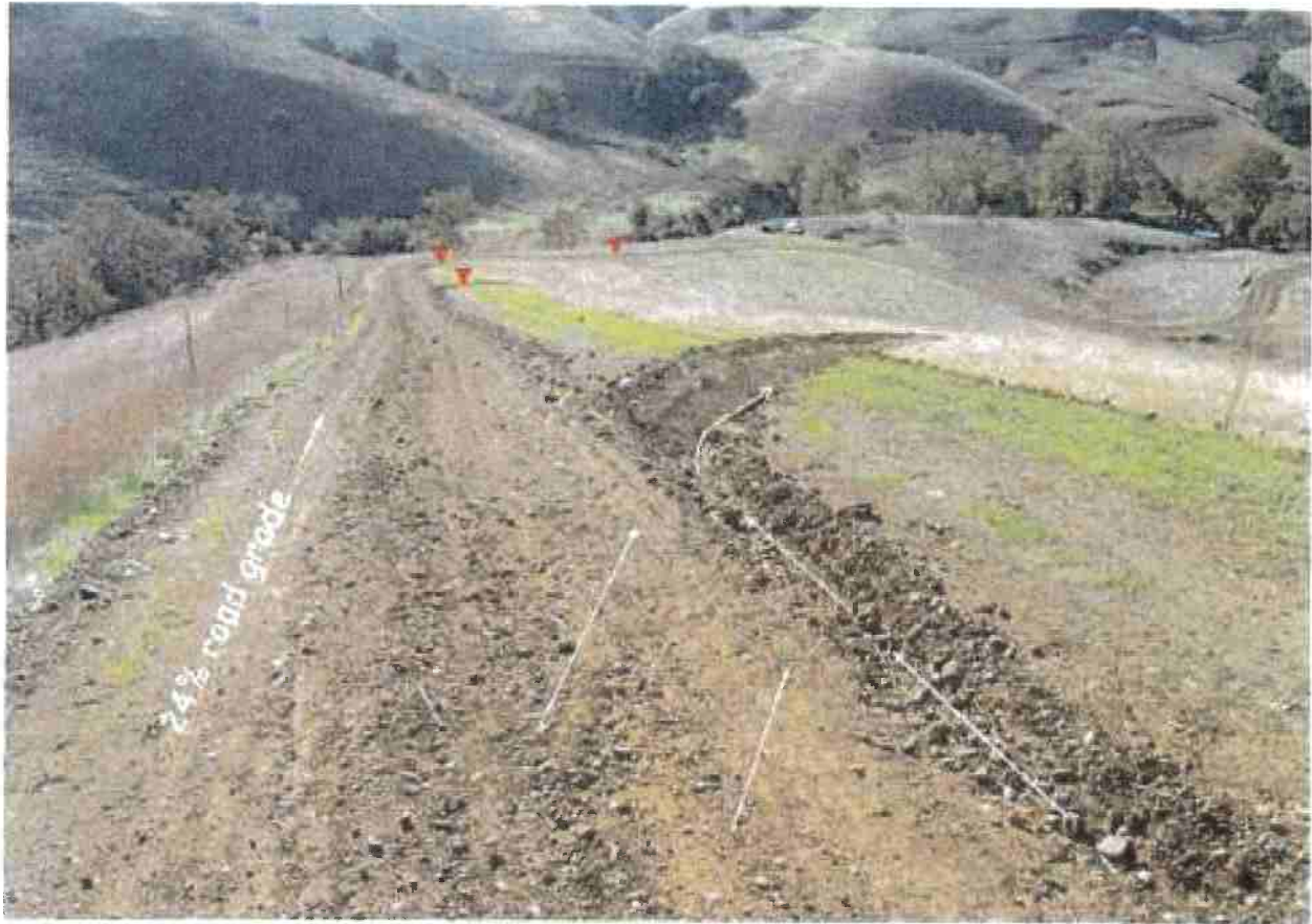
FIGURE 56. Steep roads that go straight up or down a hillside are very difficult to drain. This steep, fall line road developed a through cut cross section that was drained using lead out ditches to direct runoff off the road and onto the adjacent, vegetated hillside. The road was "outloped" to drain runoff to the right side, and the lead out ditch was built slightly steeper than the road grade, to be self-cleaning. Four lead out ditches have been constructed at 100-foot intervals to the bottom of the hillside.
