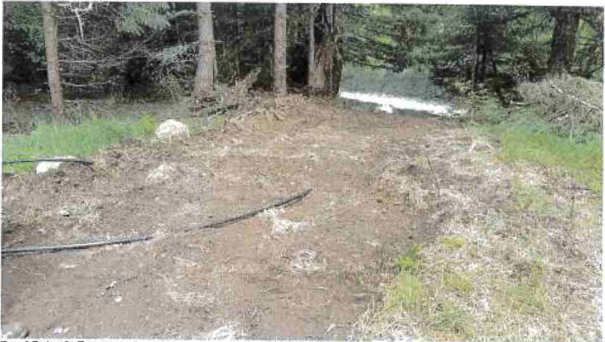
Road Point 9: Recent work on the access trail to the point of diversion's water works has resulting in disturbed soils on a slope into the lake. Seed and mulch the disturbed ground and install staked wattles.
