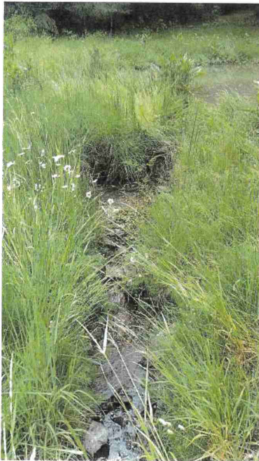
Pond Overflow (cont.): The pond's outlet is showing signs of minor erosion. Install large cobbles and small boulders along the pond's outlet.
