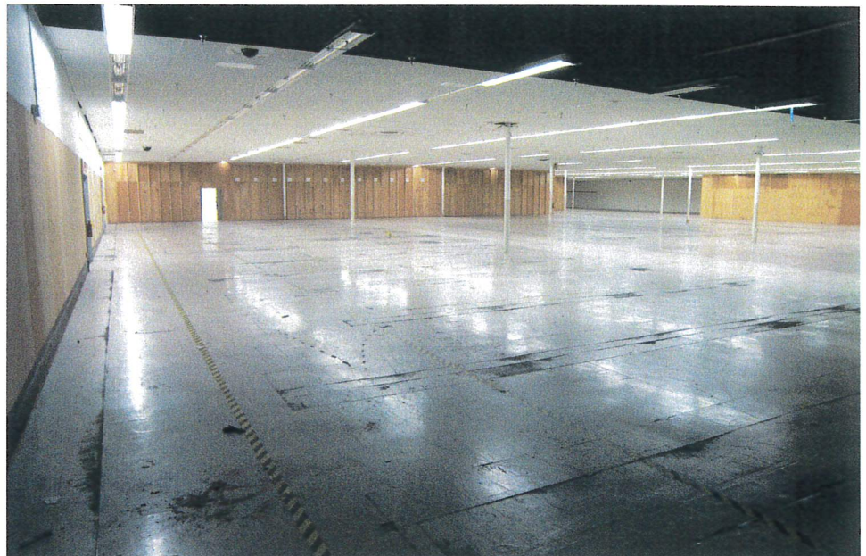
Looking southerly along rear or eastern portion of former retail sales area. Once again, notice the transition from removal of ceiling and lights with original straight ahead.
