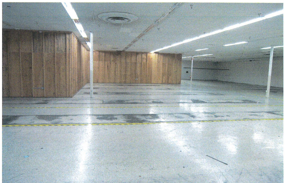
Looking southerly near middle of open retail sales area. Two additional wood frame demising walls were installed by the prior owner.
