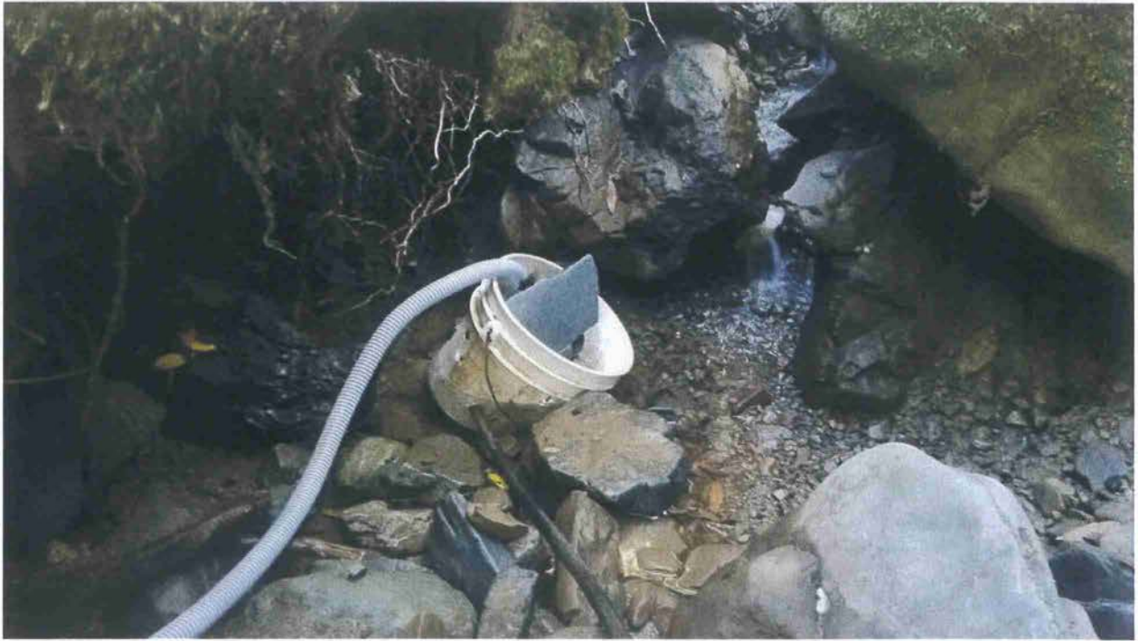
Picture 2: The Point of Diversion on a Class II watercourse. Photo date 7-06-2017.
