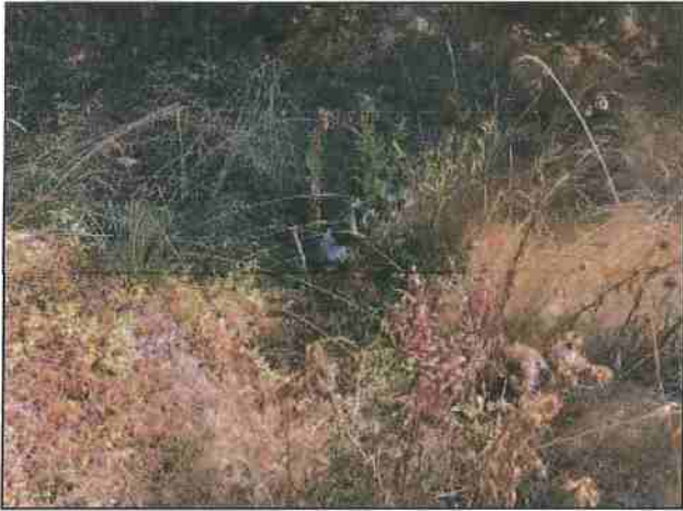
Photo #754 Private Access Rd Looking @ Partially Clogged 18" Culvert In
