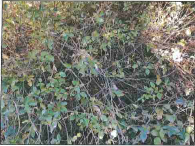
Photo #139 River Rd Looking @ Partially Clogged 36" Culvert In
