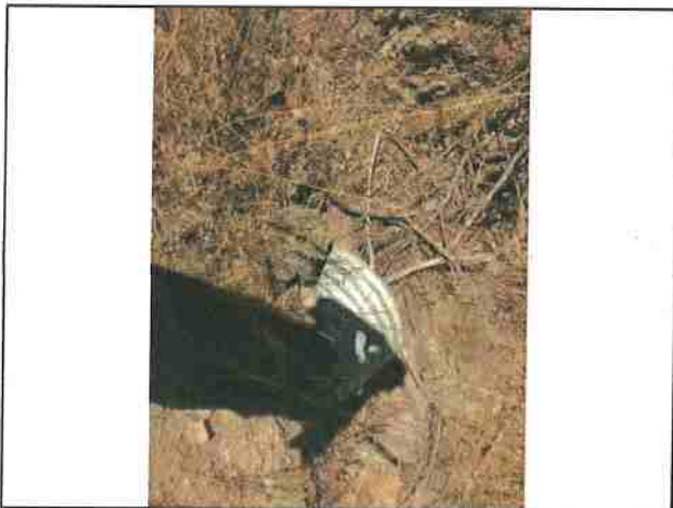
Photo #179 River Rd Looking @ Partially Clogged 36" Culvert In
