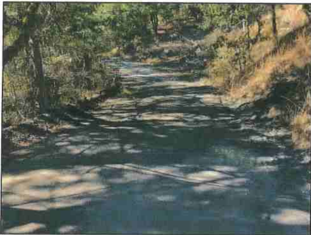
Photo #99 River Rd Looking NW @ Drainage Problem
