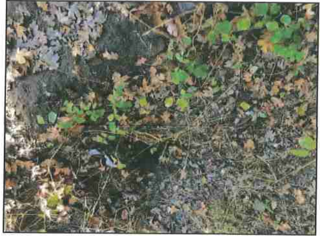
Photo #26 River Rd Looking @ Clogged 12" Culvert Out
