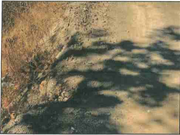
Photo #145 River Rd Looking @ Erosion Issue From Lack of Functioning Culvert
