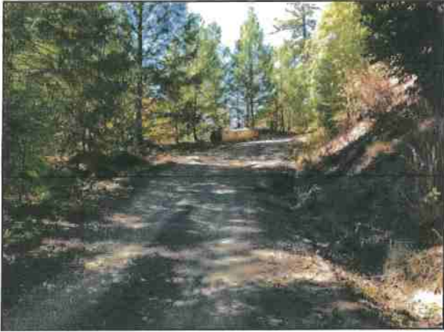
Photo #157 River Rd Looking West @ Curve w/ Turnout & Old Culvert Seen In Photo 155
