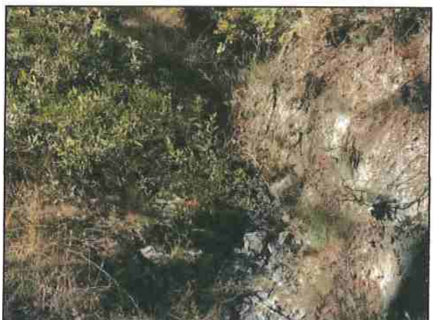
Photo #90 River Rd Looking @ Clogged 24" Culvert In
