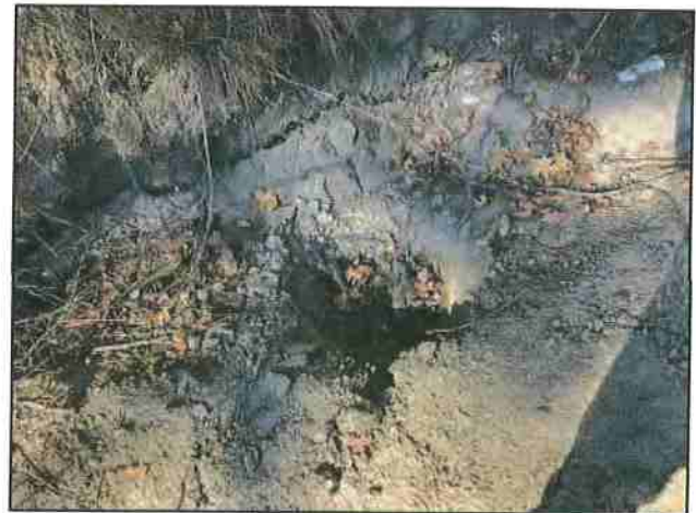
Photo #114 River Rd Looking @ Erosion Issue
