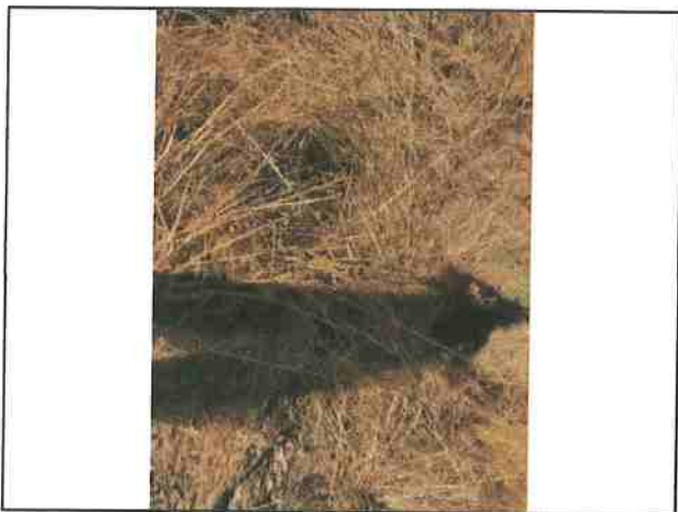
Photo #29 River Rd Looking @ Clogged 12" Culvert In
