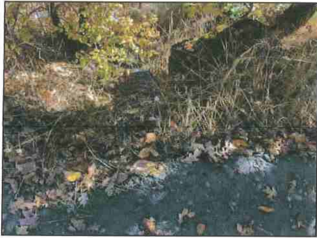
Photo #49 River Rd 12" Culvert Out
