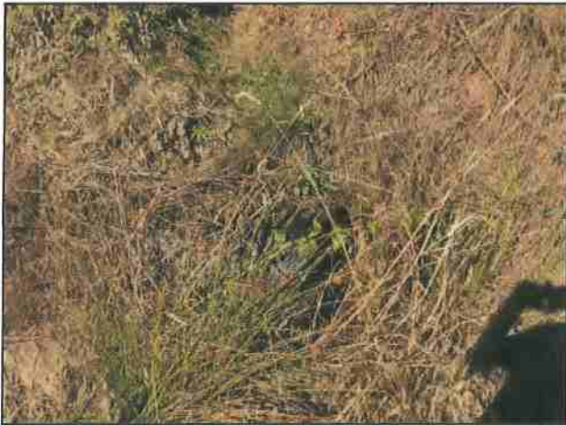
Photo #171 River Rd Looking @ 24" Culvert Out Under Approach Running East to West
