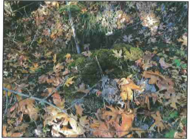
Photo #104 River Rd Looking @ Partially Clogged 36" Culvert In
