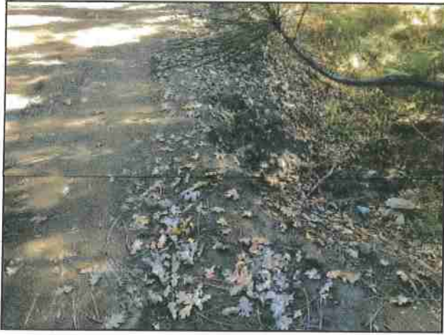
Photo #25 River Rd Looking @ Clogged 12" Culvert In
