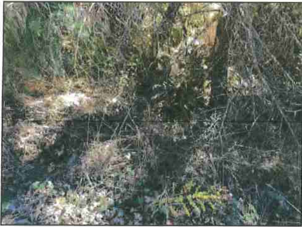
Photo #61 River Rd Looking @ Clogged Culvert In
