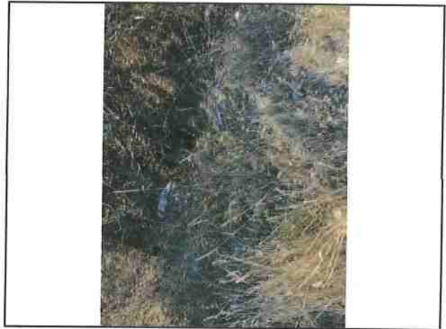
Photo #28 River Rd 12" Clogged 12" Culvert Out
