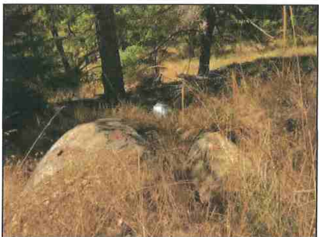
Photo #747 Private Access Rd @ 18" Culvert Out. Culvert In Was Not Found
