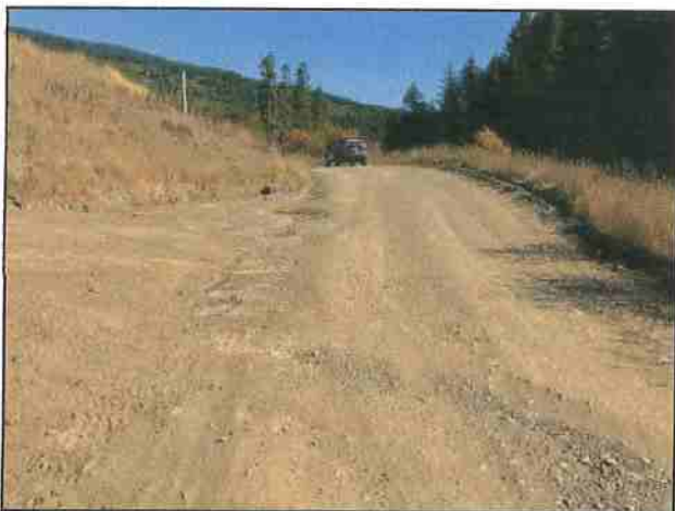
Photo #41 River Rd Looking East @ Curve w/ Pullout & Approach w/ Erosion from Drainage
