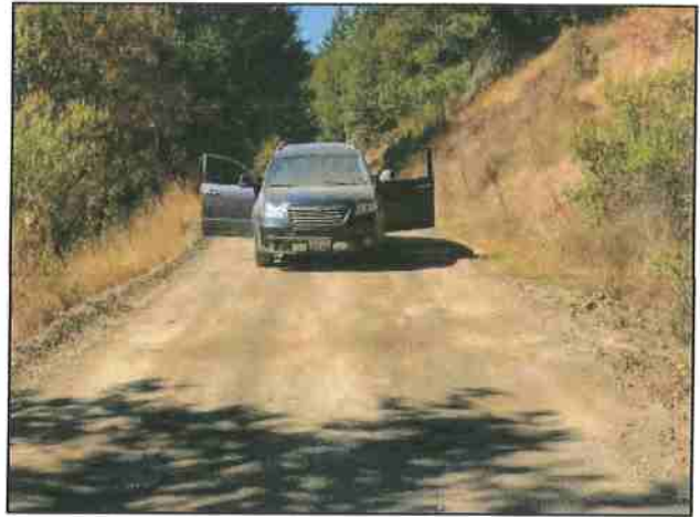
Photo #140 River Rd Looking West @ Drainage Issue
