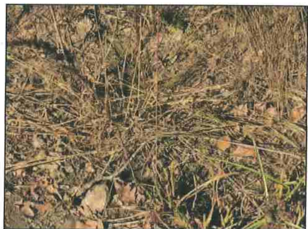
Photo #144 River Rd Looking @ Potential Clogged Culvert Inlet. Outlet Was't Found
