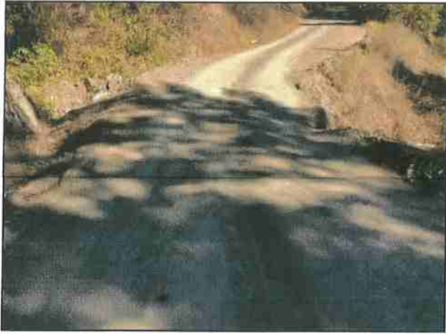
Photo #127 River Rd Looking @ Culvert Location In Photos 126 & 125 Erosion Area
