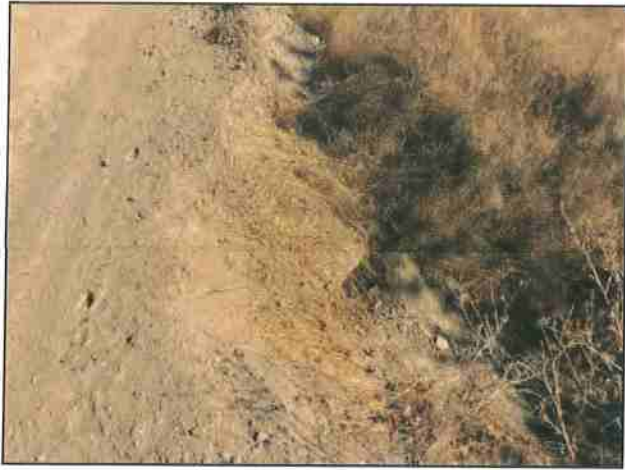
Photo #31 River Rd Looking SE Closeup @ Erosion
