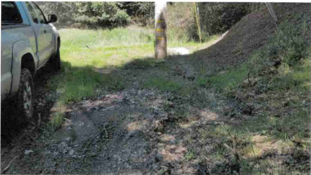
Road Point 1: An inside ditch is discharging into the inlet of a Class II watercourse crossing. Install five wattles or rock check dams in the inside ditch and dispersal field of the inside ditch leading up to the Class II watercourse.
