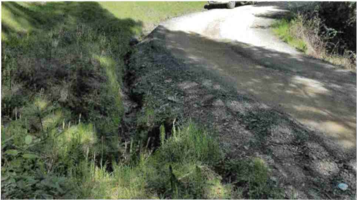
Road Point 11 & 12: Two inside ditches are discharging into a Class III watercourse. Install five wattles or rock check dams in the inside ditch and dispersal field of the inside ditch leading up to the Class III watercourse. (There is no photo for Road Point 11)
