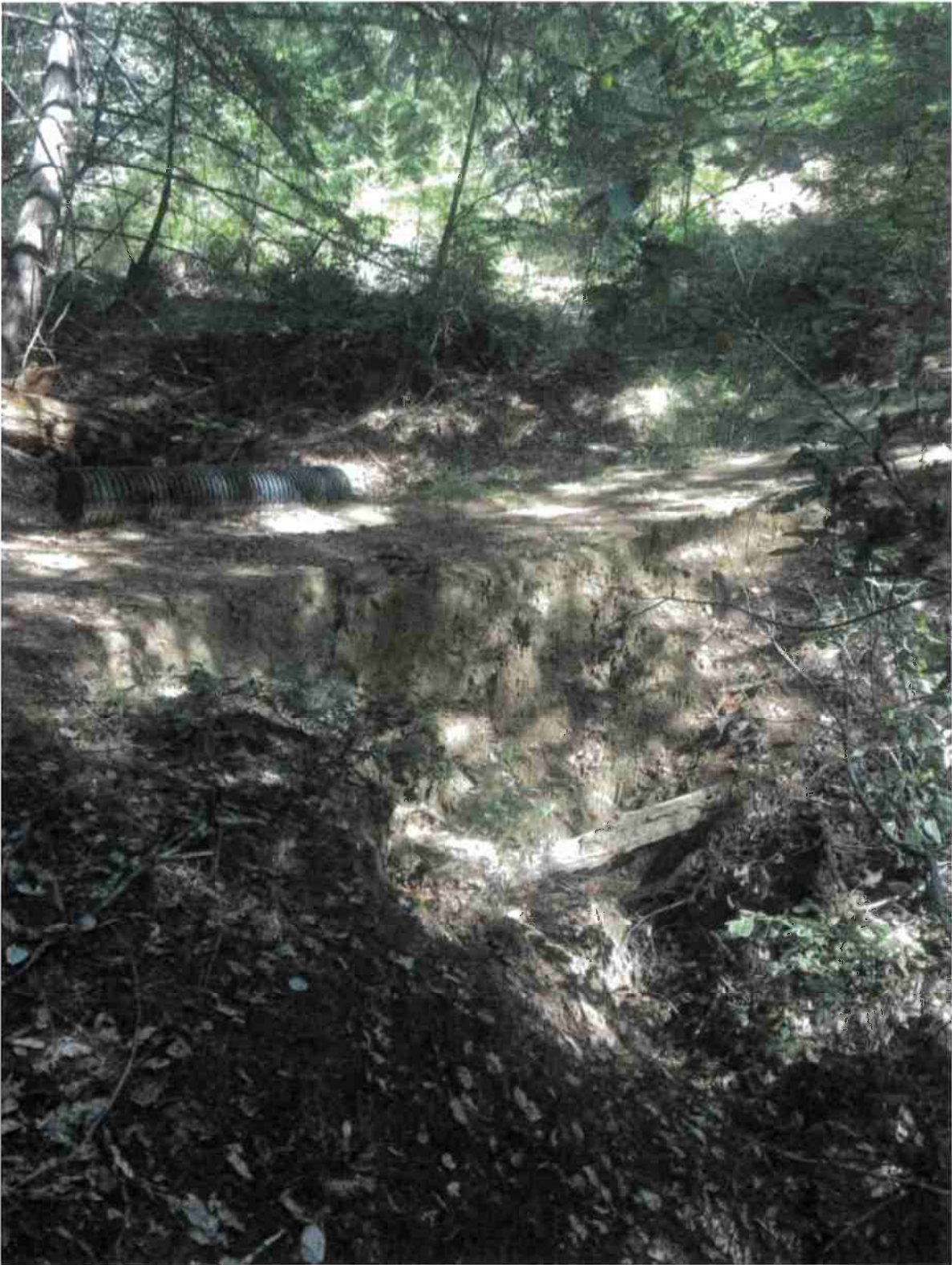
Stream Crossing 7: Class III watercourse dirt ford crossing. Install a 24" diameter culvert per attached specifications.
