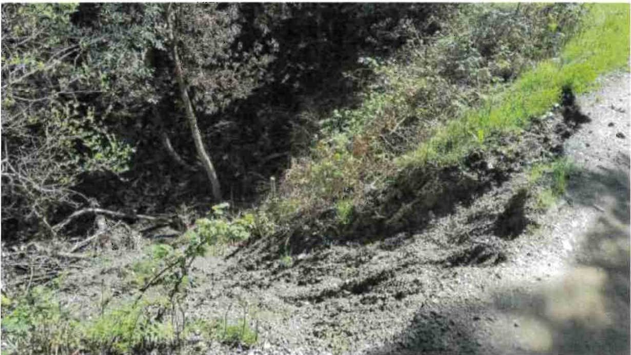
Road Point 8: The road's fill slope is wasting down onto the stream flood plain below. Re-establish the road by installing an armored fill and rock armoring the fill slope.
