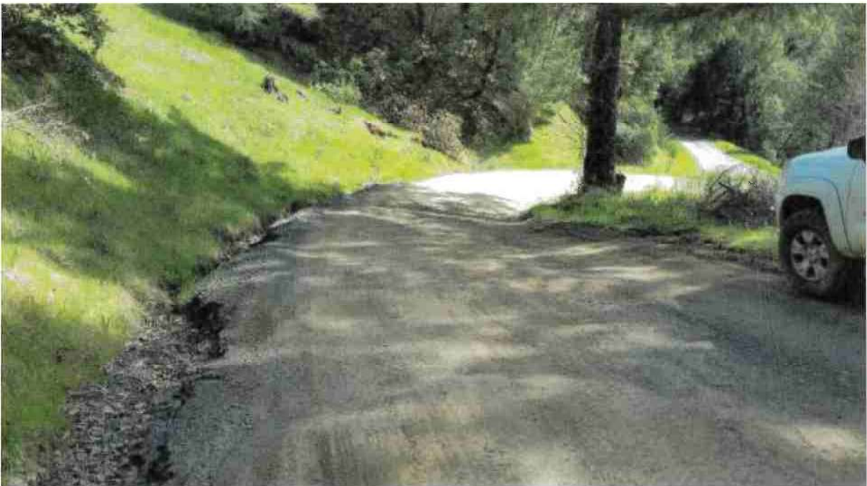
Road Point 10: Steep through cut segment of the road where the inside ditch has been filled in by soft road surface soil and rock. Clear and rock line the inside ditch and rock the adjacent road with 4 – 6" crushed angular rock approximately 120' above and below Road Point 10.
