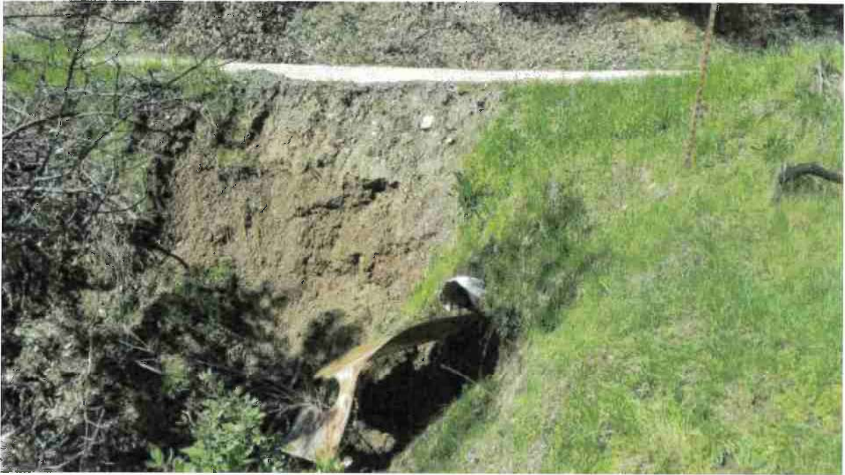
Ditch Relief Culvert 3: 12" diameter ditch relief culvert. The inlet is becoming plugged from road surface debris, mud and vegetation. Clear the inlet of mud, debris, and vegetation and rock armor the inlet and outlet per attached specifications. Also remove the metal sheet that is attached to the outlet of the culvert.
