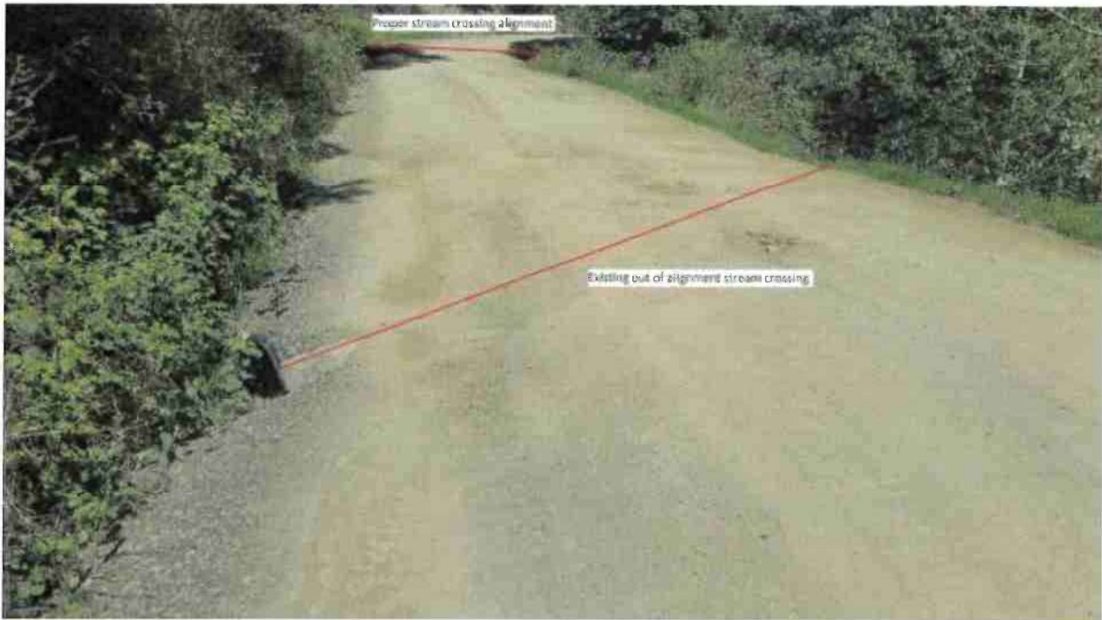
Stream Crossing 3: Class III watercourse crossing with a 36" diameter smooth-walled pipe placed out of alignment of the watercourse. Install a minimum 24" culvert approximately 80' down the road in the natural historic channel per attached specifications. The approximate location of the new crossing installation is represented as "NEW SC 3" on the attached maps.
