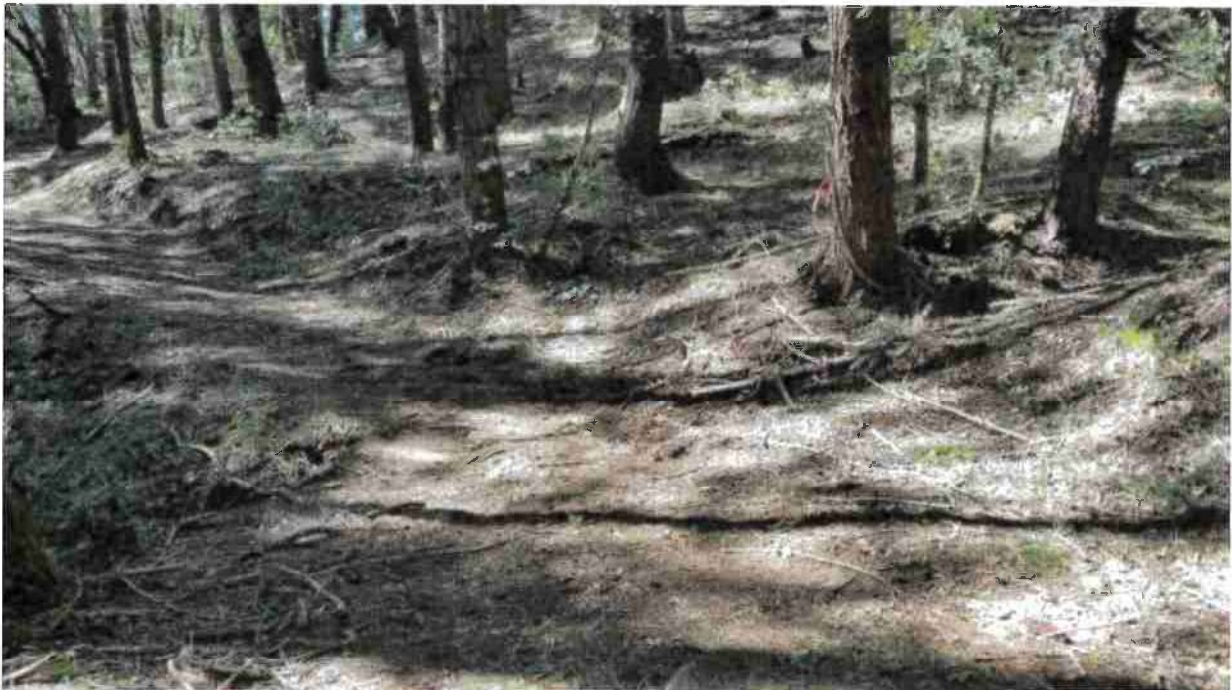
Stream Crossing 6: Class III watercourse dirt ford crossing. Install a rocked ford per attached specifications.
