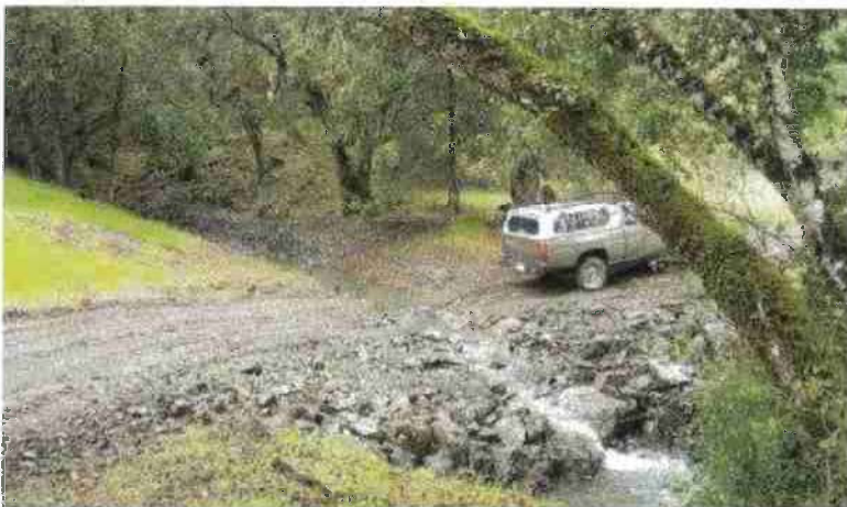
FIGURE 121F. The same armored fill as it appeared after the first winter flood flows. No maintenance was required to reopen the road. It is also clear that no stream diversion is possible at this stream crossing site, and the volume of fill within the crossing has been reduced to the minimum amount needed to maintain a relatively smooth driving surface on this low volume road.
