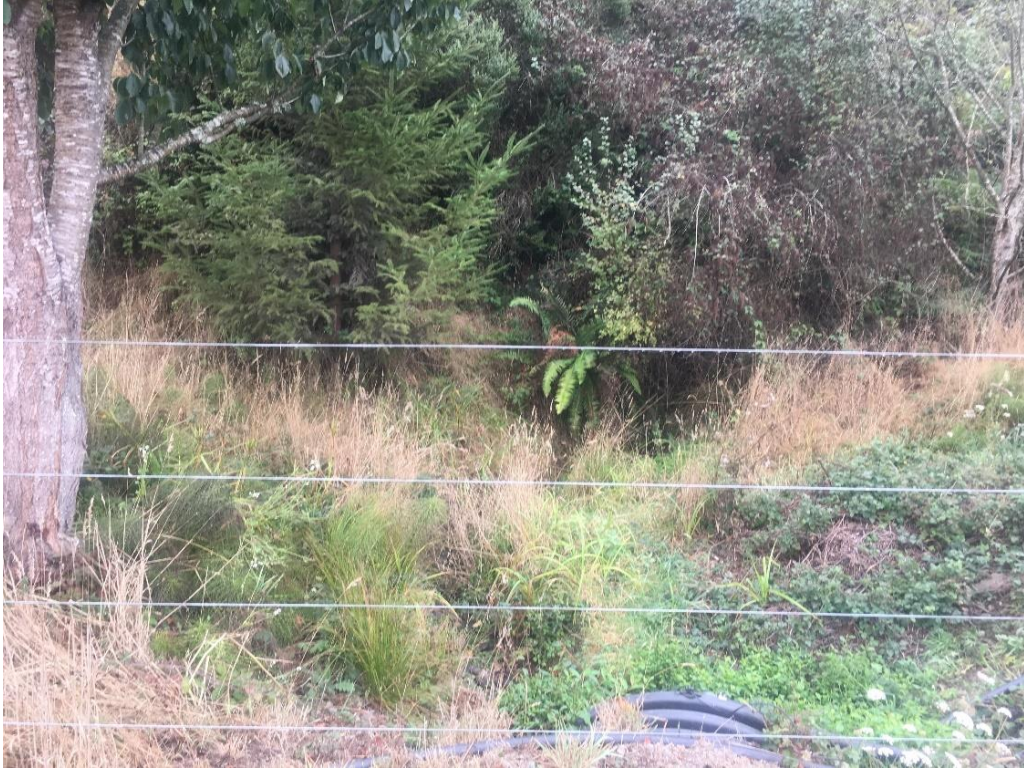
Photo 5. View south of the inlet side of Gravelly Point Creek drainage (dry since July)
