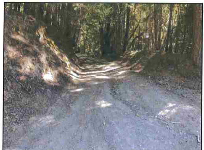
Photo #615 Mad River Trail @ Turnout Location Looking SE @ Curve w/ Rutting (Poor Drainage)
