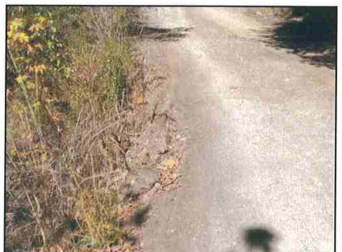
Photo #270 River Rd Looking @ Drainage & Erosion Issue
