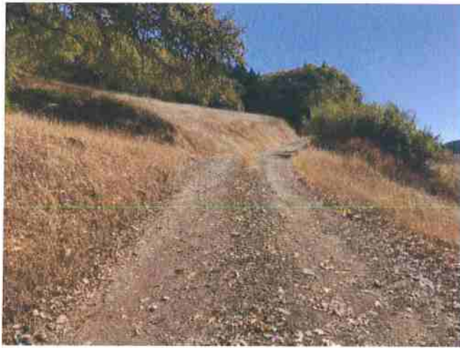
Photo #600 Mad River Trail Looking SE @ Hill-side Slip & Drainage Issue
