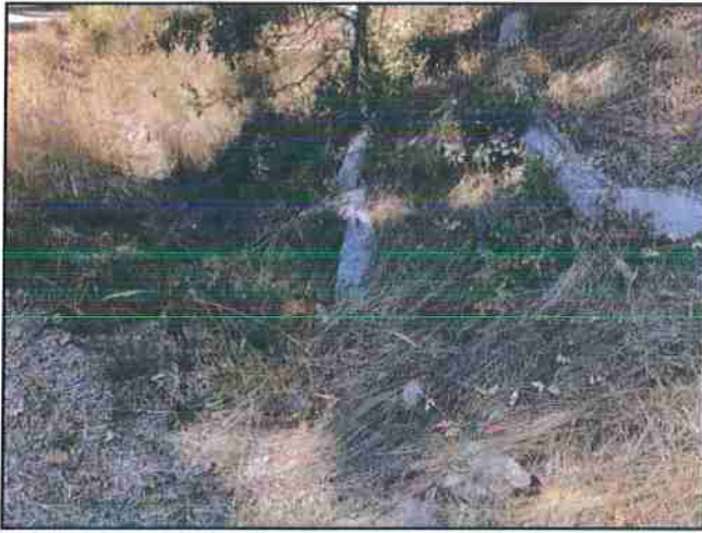
Photo #169 River Rd Looking @ Partially Clogged 24" Culvert Under Approach Running E to W
