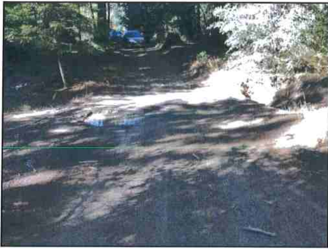
Photo #439 River Rd @ Turnout Location Looking NW @ Drainage Issue
