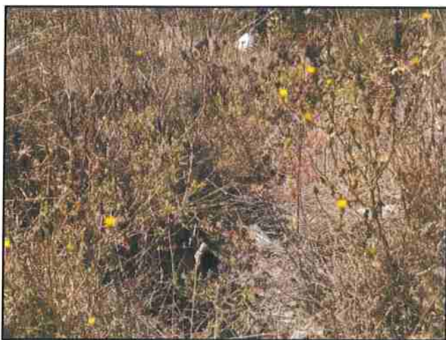
Photo #257 River Rd Clogged Culvert Out (Size Unknow)
