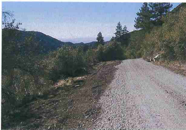
Figure 1. Low-volume road that has been newly gravelled and out-sloped, San Bernardino County. Photo: Richard Harris.
