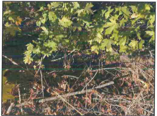
Photo #224 River Rd Looking @ Partially Clogged 24" Culvert In
