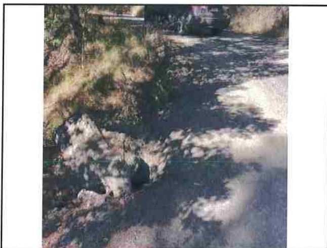
Photo #239 River Rd Looking NW @ Erosion Issue @ Curve
