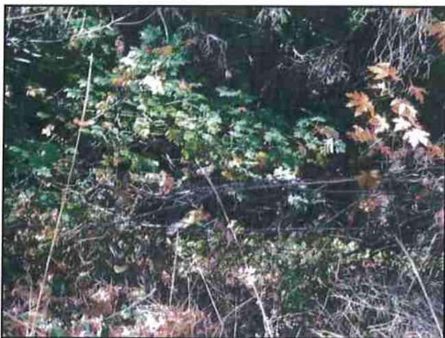
Photo #269 River Rd Looking @ Clogged Culvert Out (Size Unknown)
