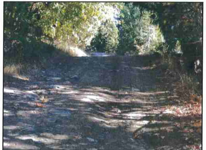
Photo #322 River Rd Looking NE @ Rutted Area Due to Poor Drainage
