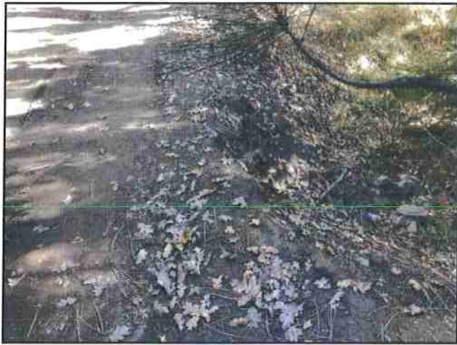
Photo #25 River Rd Looking @ Clogged 12" Culvert In
