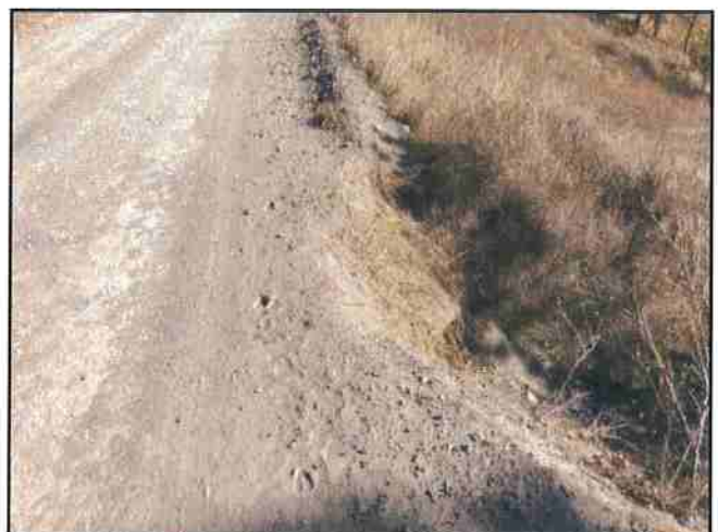
Photo #30 River Rd Looking SE @ Erosion
