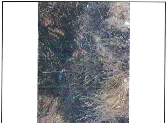
Photo #28 River Rd 12" Clogged 12" Culvert Out
