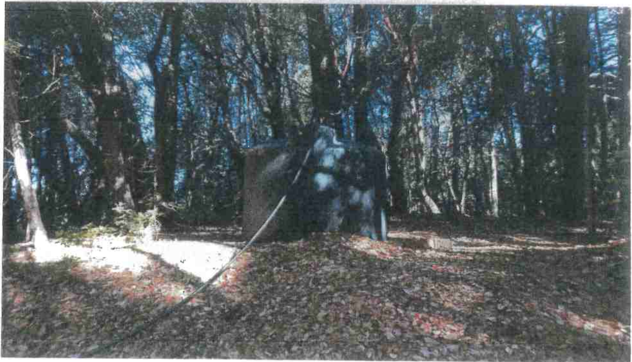
Picture 3 & 4: Six 5,000-gallon and one 2,500-gallon water storage tanks. Photo date: 8/22/2019.
