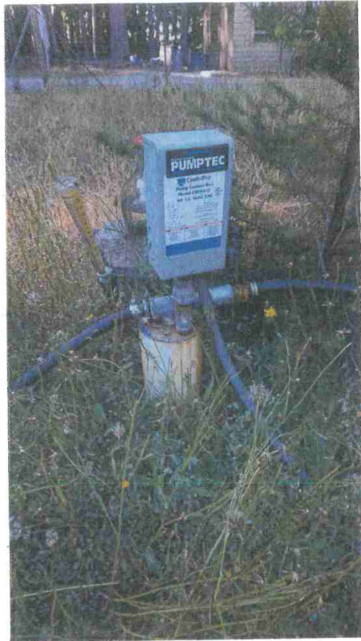
Picture 2: Groundwater well which supplies all water on the property. Photo date: 8/22/2019.
