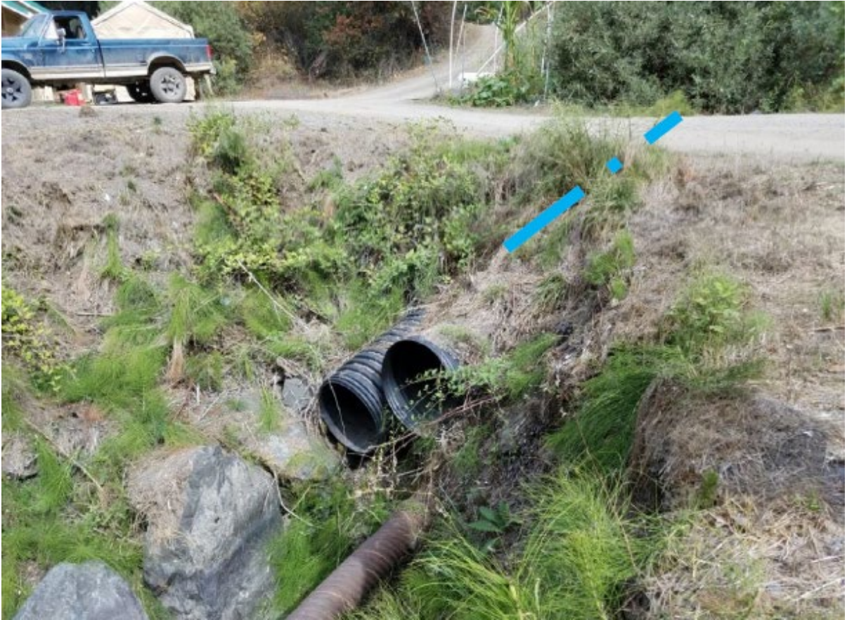
Photo 3: Stream crossing (STX-2) - two 30-inch plastic culverts to be upgraded.
