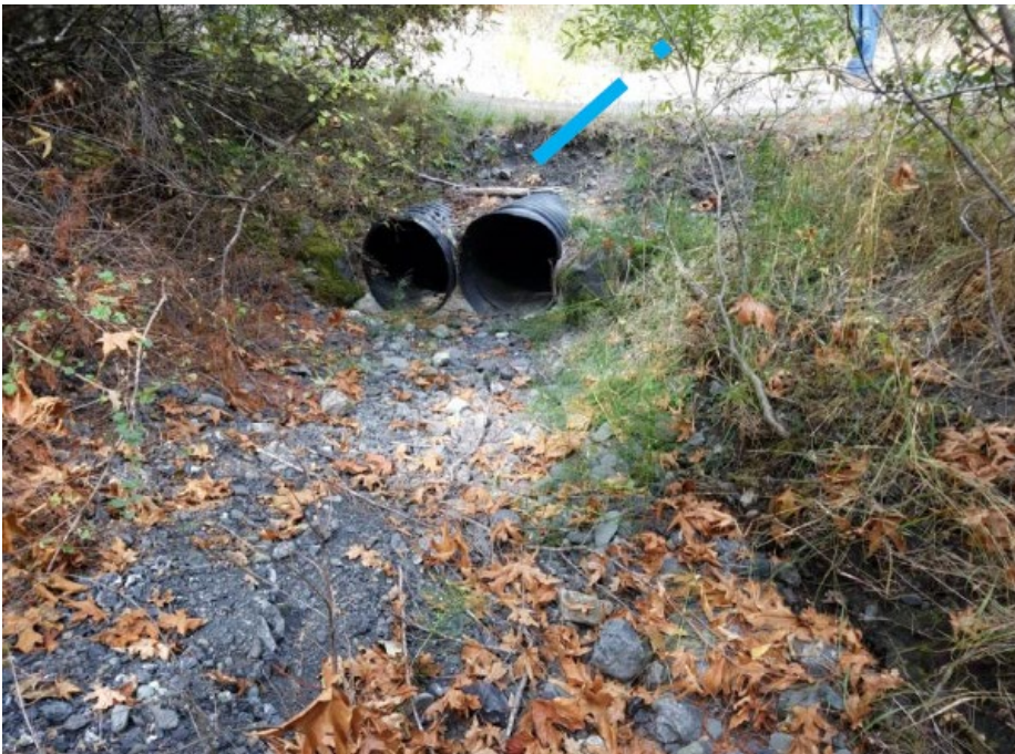
Photo 2: Stream crossing (STX-1) - two 30-inch plastic culverts to be upgraded.
