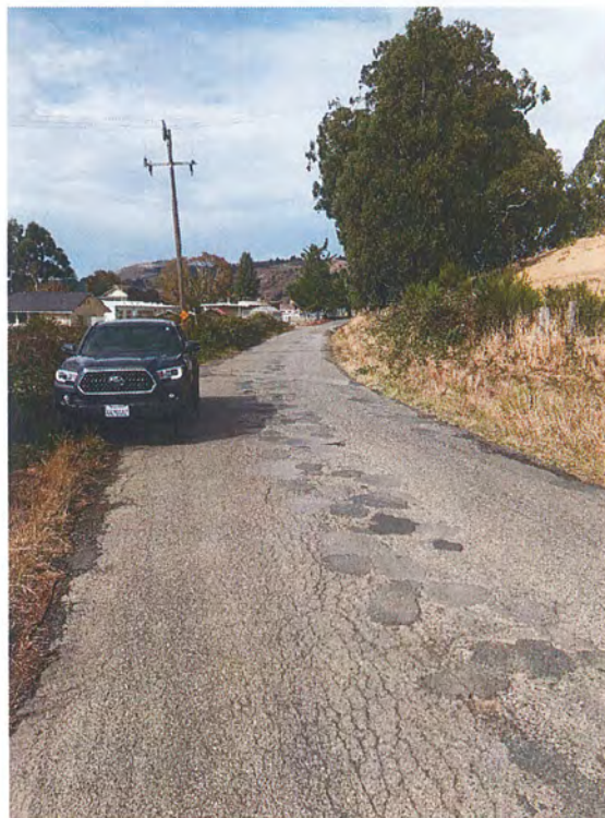
Figure 4: RP 2. Typical section of Chambers Rd (County maintained. State Road No.: FC010). Vehicle traveling east, photo taken facing west.
