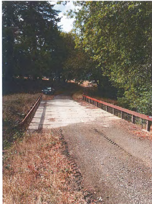
Figure 28: RP 11. Two-Lane Bridge. Vehicle parked in turnout. Vehicle traveling east, photo taken facing west.
