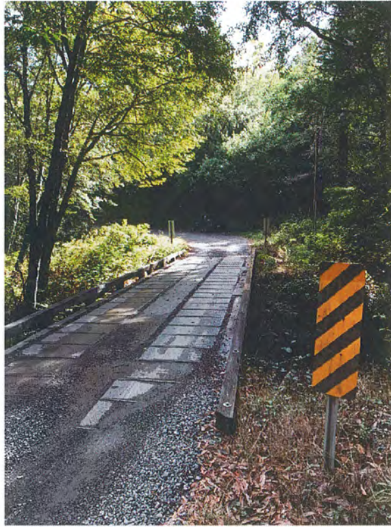
Figure 9: RP 4. Single-Lane Bridge. Vehicle traveling east (parked in large turnout east of bridge), photo taken facing east.
