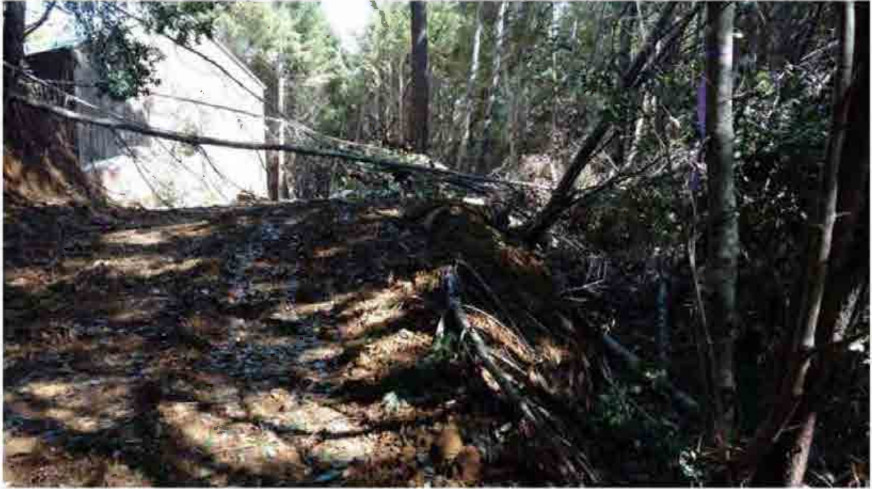
Figure 13. Site number 13, road drainage needed, rolling dip location
