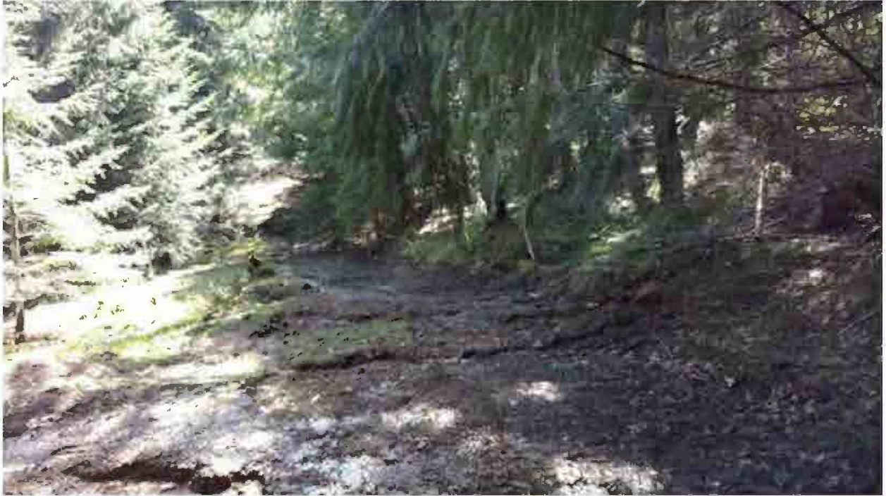
Figure 8. Site number 7, fill crossing on a Class III Watercourse part of flow diverted down the road to Site 6
