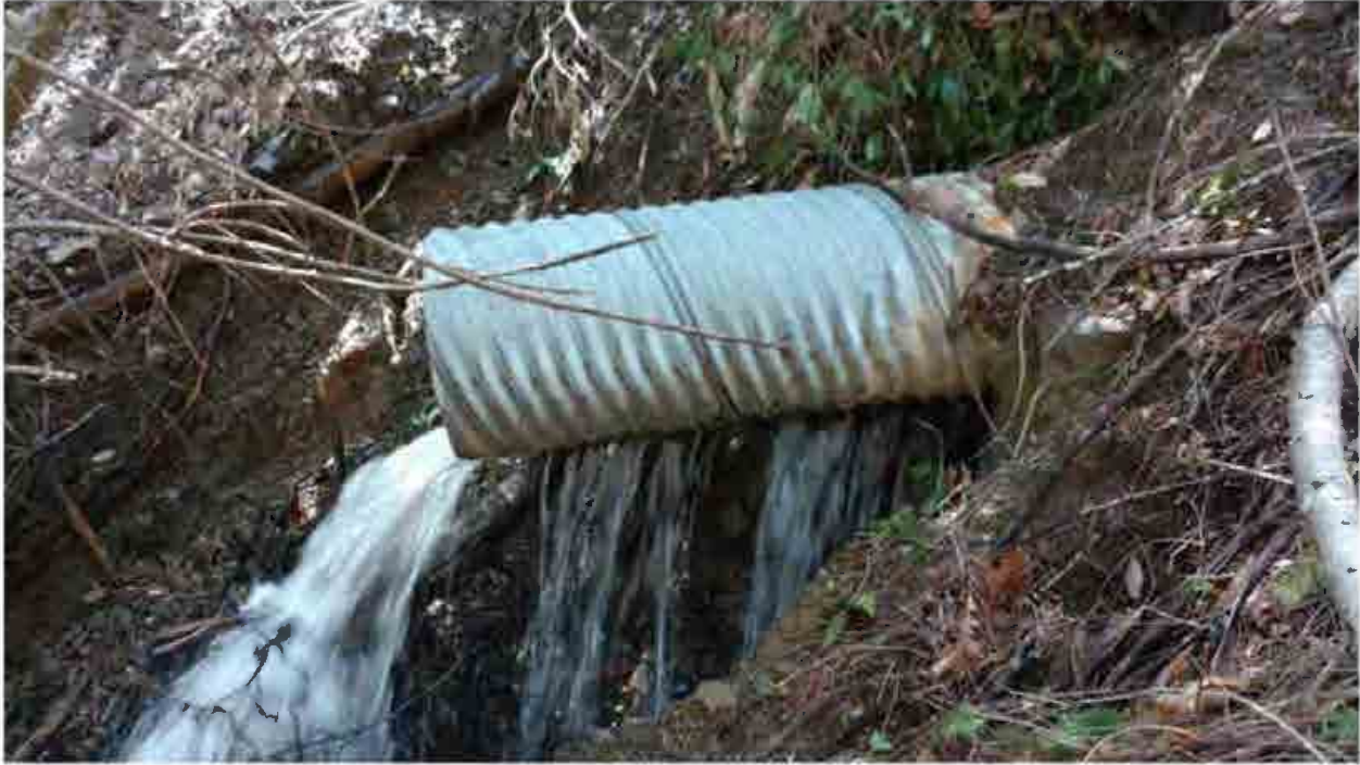
Figure 32. Site number 31, culvert outlet is above stream grade and rusted through in multiple places
