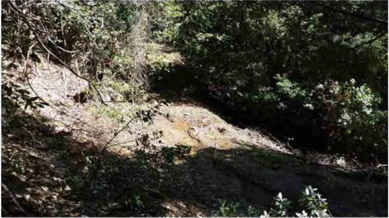
Figure 9. Site number 8, road drainage needed, rolling dip location
