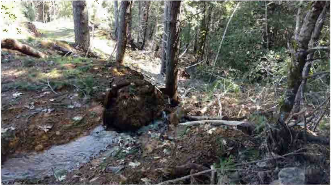
Figure 23. Site number 22, fill material eroding into the Class III watercourse at the point it leaves the inboard ditch
