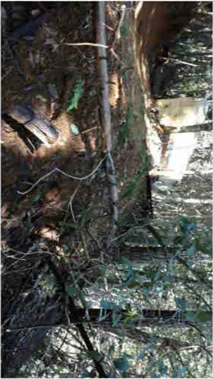
Figure 3. Site number 3, perched fill outside the WLPZ but above Class II Stream
