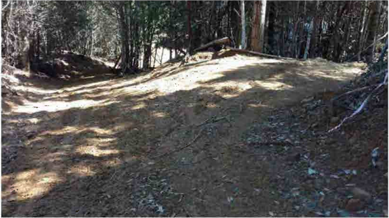
Figure 17. Site number 16, road drainage needed, rolling dip location
