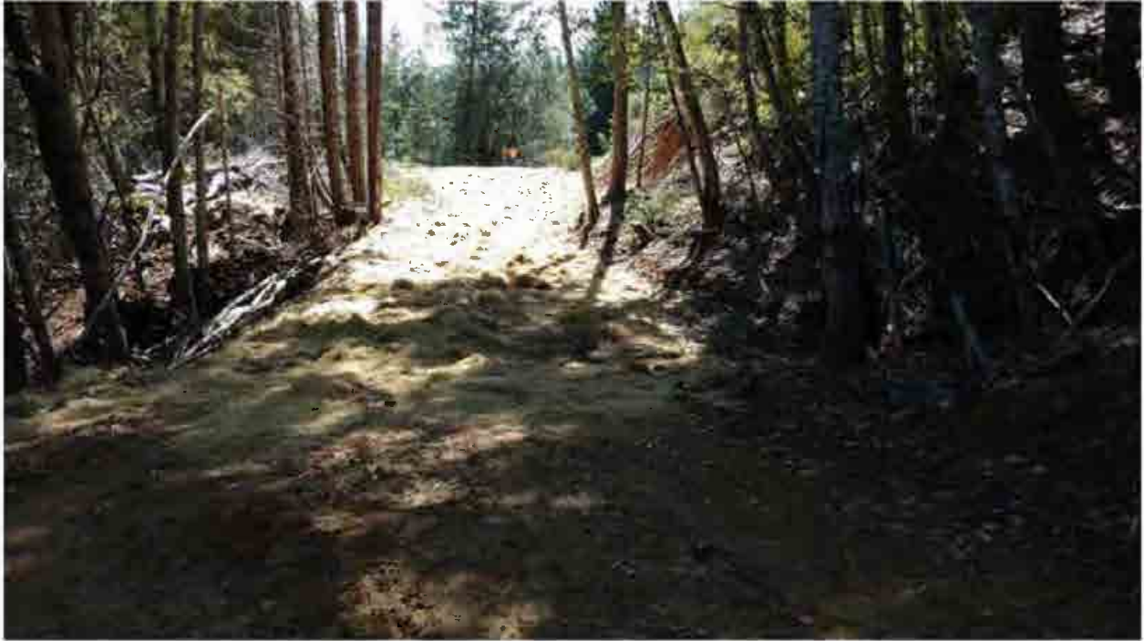
Figure 18. Site number 17, road drainage needed, rolling dip location
