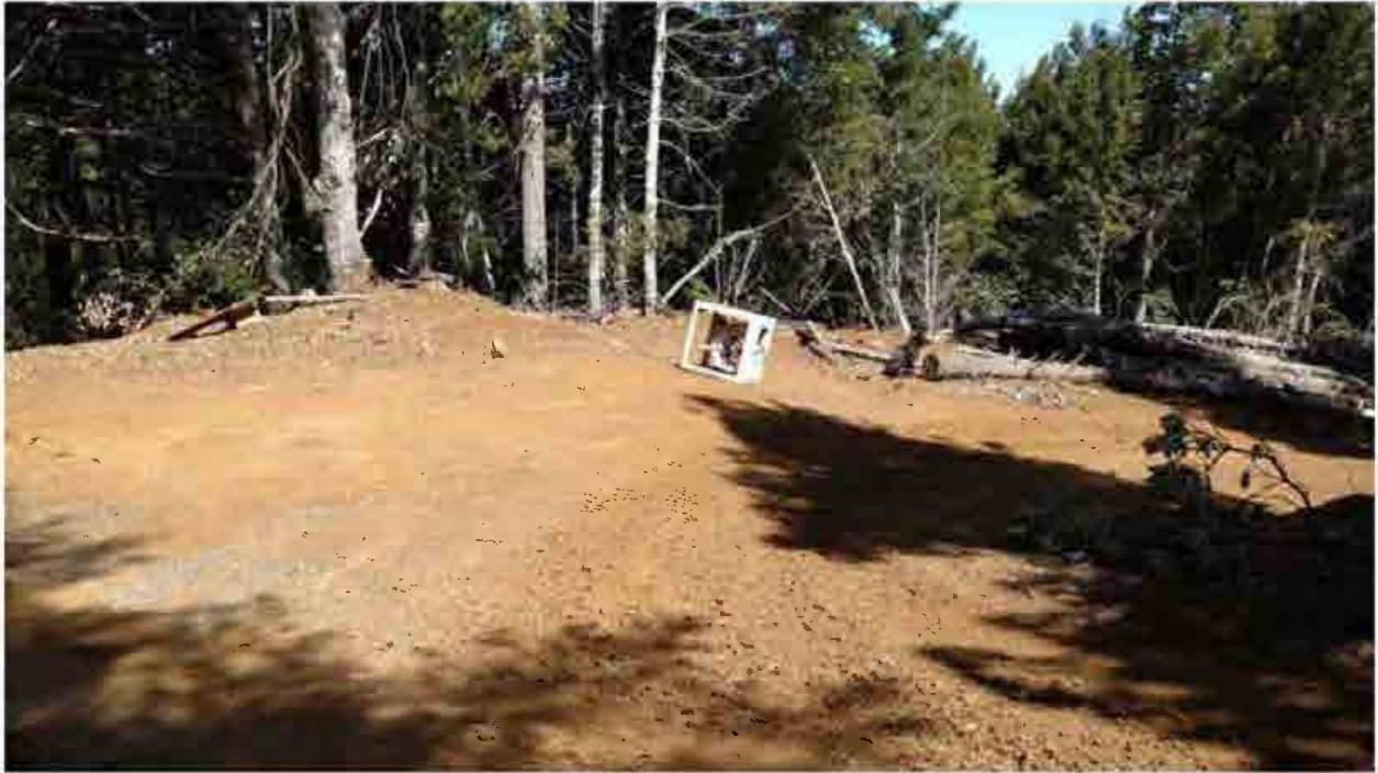
Figure 26. Site number 26, road drainage needed, rolling dip location
