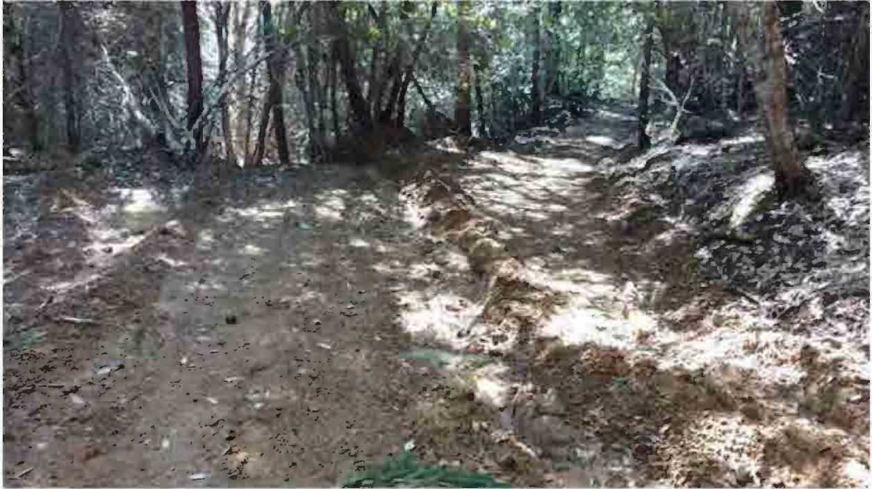
Figure 10. Site number 9, road drainage needed, rolling dip location
