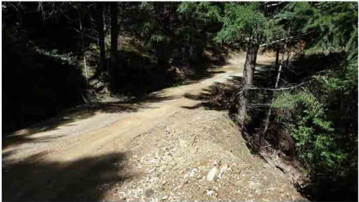
Figure 31. Site number 31 as seen from the road, the Class II crossing currently contains a 24" by 50' long culvert that is rusted at the outlet. The Culvert is currently functional but is likely to fail in the future if left as is. Crossing shall be replaced with a 40" by 60' long culvert
