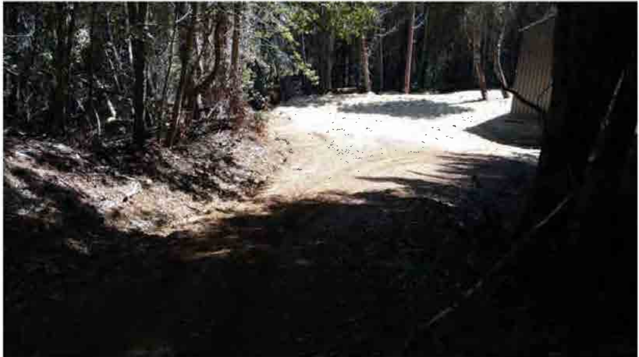
Figure 16. Site number 15, road drainage needed, Install 18" ditch relief culvert.
