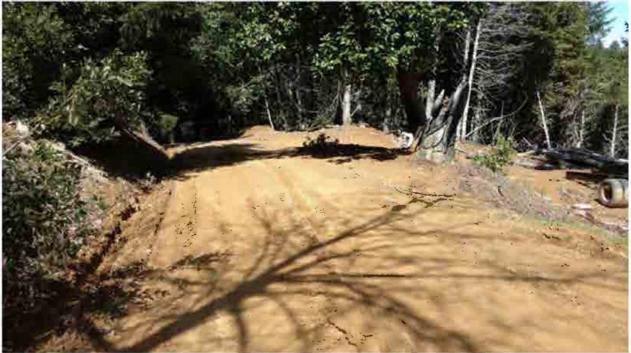
Figure 29. Site number 29, road drainage needed, rolling dip location
