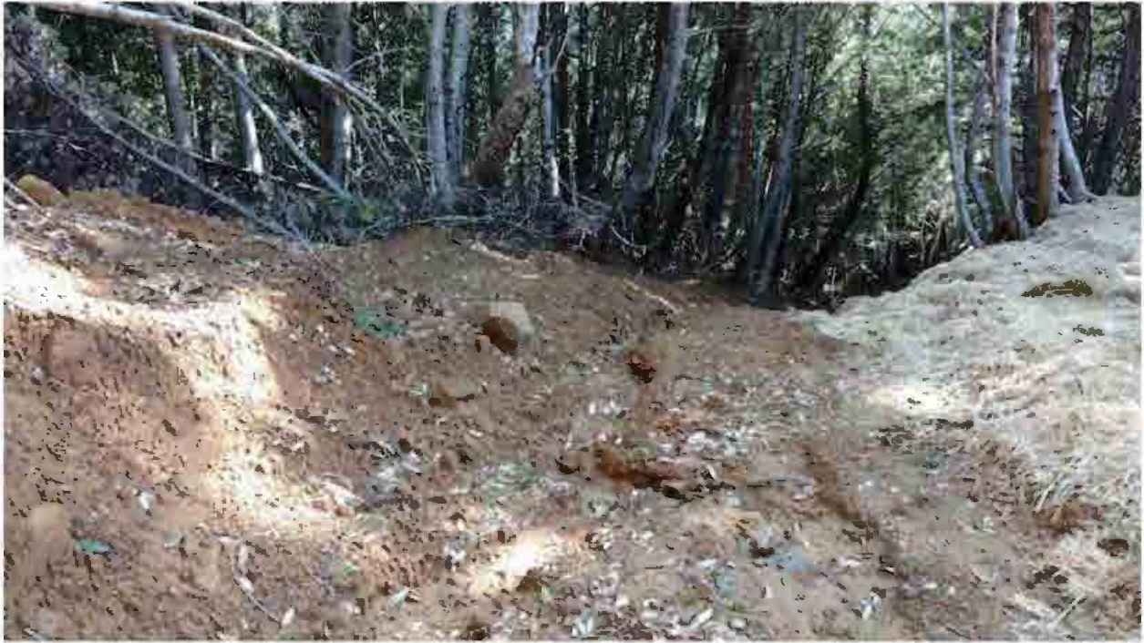
Figure 11. Site number 11, road drainage needed; rolling dip location the bank on the left side of the photo will need a ditch excavated through it.
