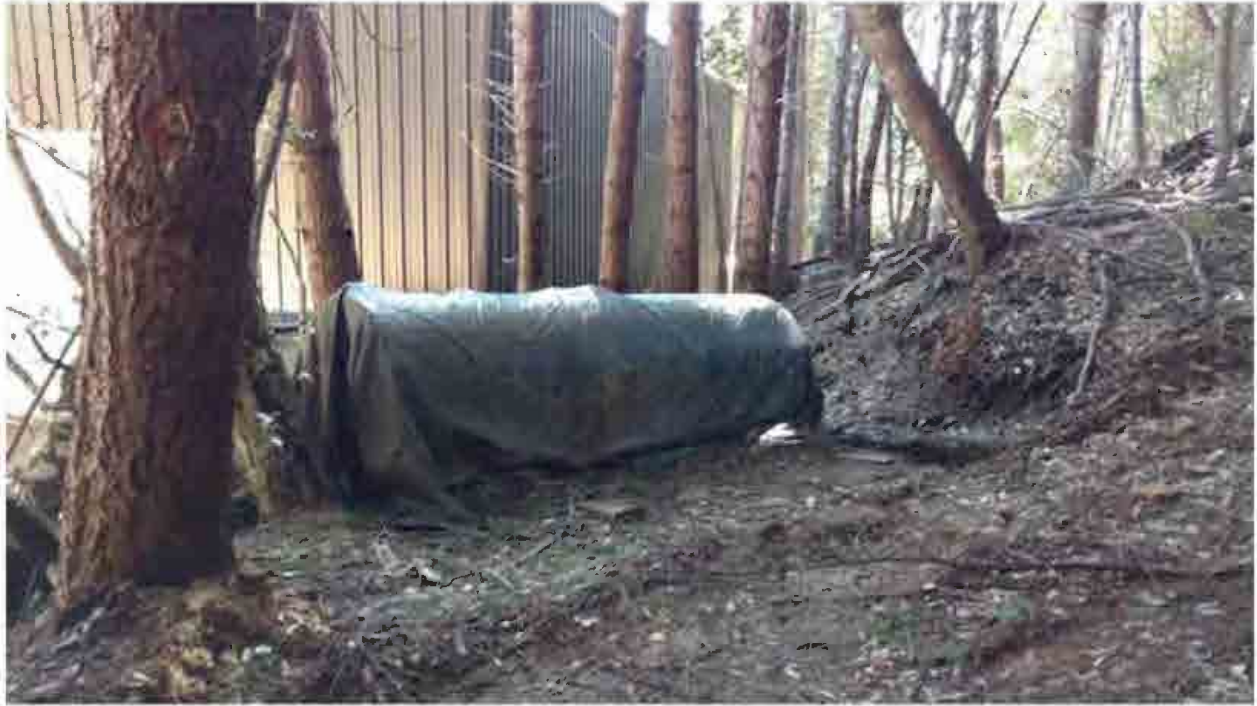
Figure 15. Site number 14, fuel storage tank without containment
