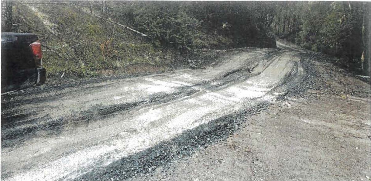
Photo looking southwest at Site 04. Note road rutting and rock surfacing. Additional competent rock surfacing (4" – 6" crushed angular) will be required here.
