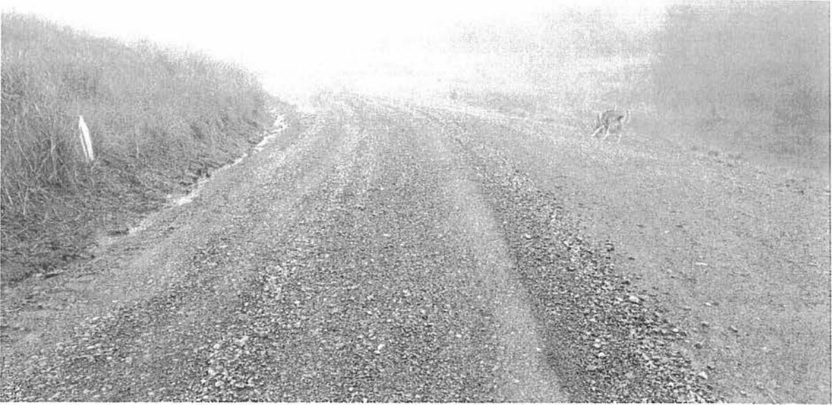
Photo looking down grade at Site 08. A ditch relief culvert will be installed here to drain the long, undrained, inside ditch that is discharging into a wetland area and the head of a Class III watercourse crossing. Note road rock surfacing and the stable road base. The majority of roads on the property are in similar condition.
