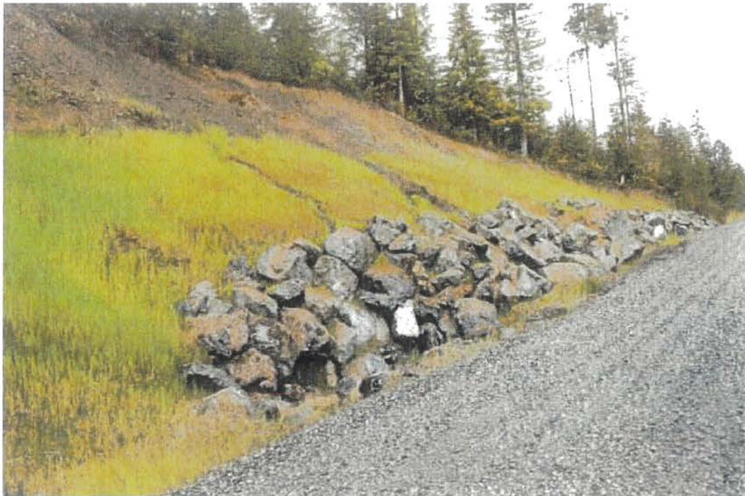
FIGURE 52. This wet and potentially unstable cut slope on a newly constructed road was stabilized using a buttress of large rock armor. To assure their effectiveness, rock buttresses and other retaining structures should be designed by a qualified engineer or engineering geologist.
