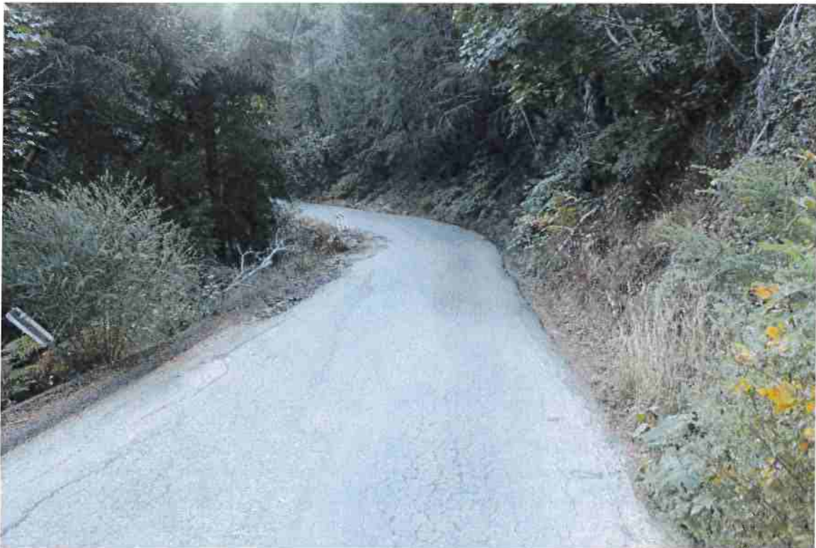
Photo 26. Mile 2.35: ~15-ft road width pinch point at partial road failure.
