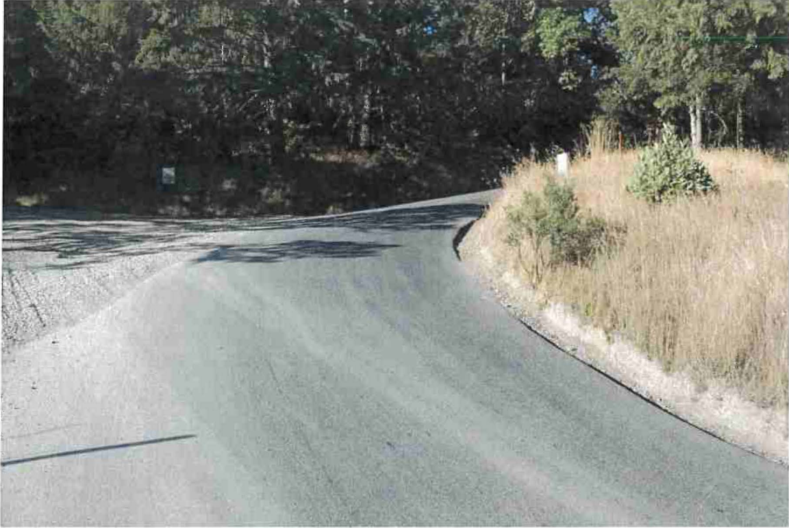
Photo 45. Mile 3.85: Blind corner at intersection with Lower Thomas Road. 16-ft road width with 1-ft shoulders. Potential location to widen corner on inside to improve visibility.
