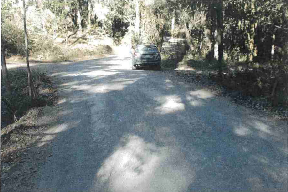
Photo 13. Mile 1.0: 16-ft road width with no shoulder at culvert crossing. The road could be widened at this location but not necessary because there is decent visibility.
