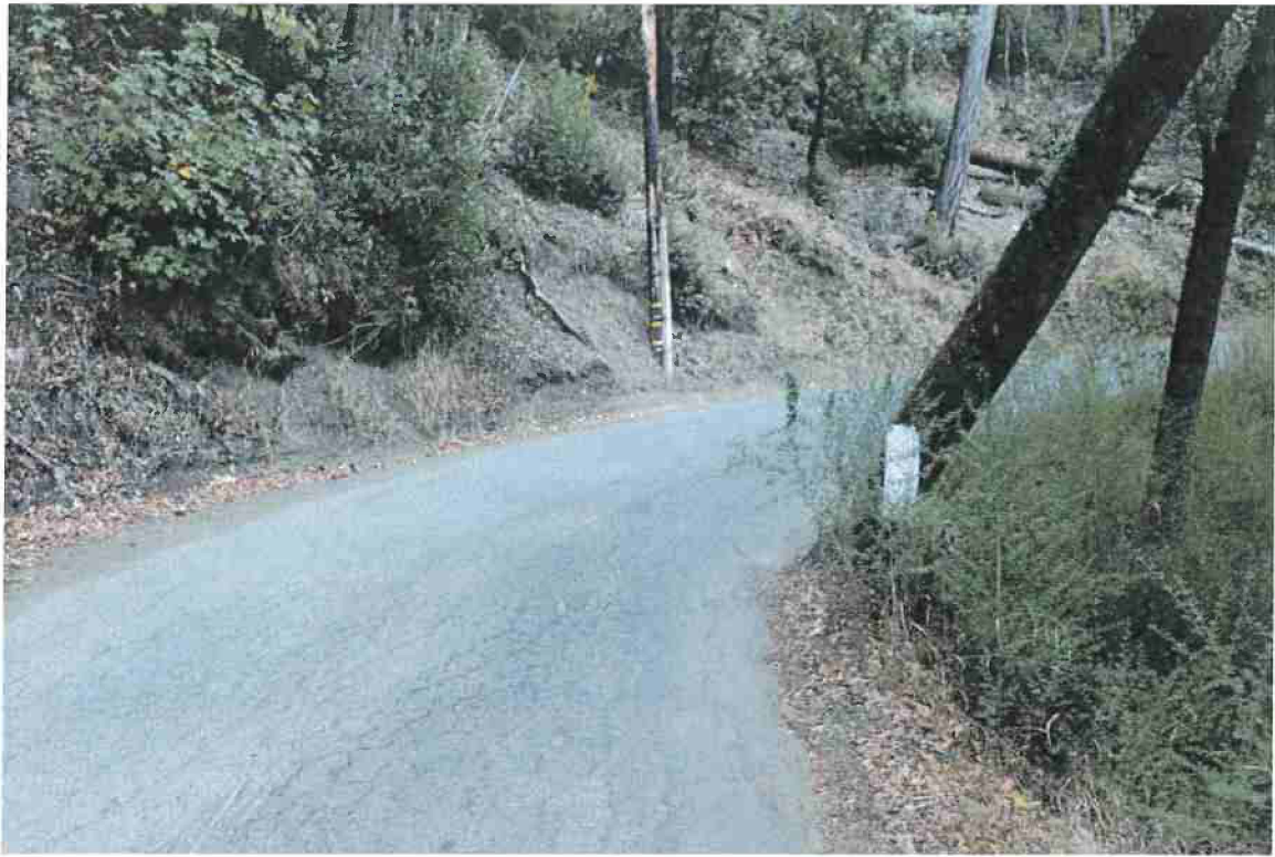
Photo 23. Mile 2.15: Pinch point at tree, 15-ft road width, 1-ft shoulder.
