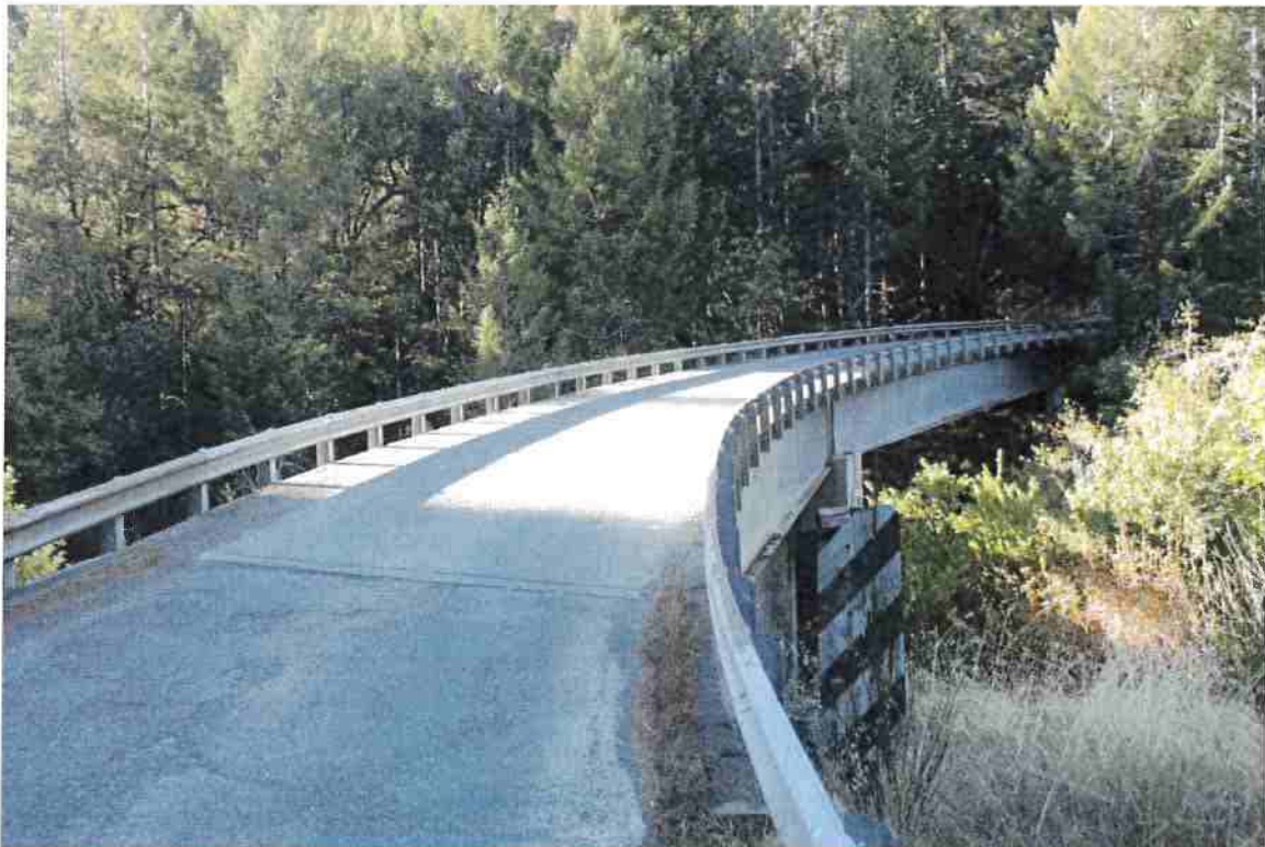
Photo 38. Mile 3.3: 16-ft wide bridge, no shoulders. Recommend removing vegetation on west extent of bridge to improve visibility.
