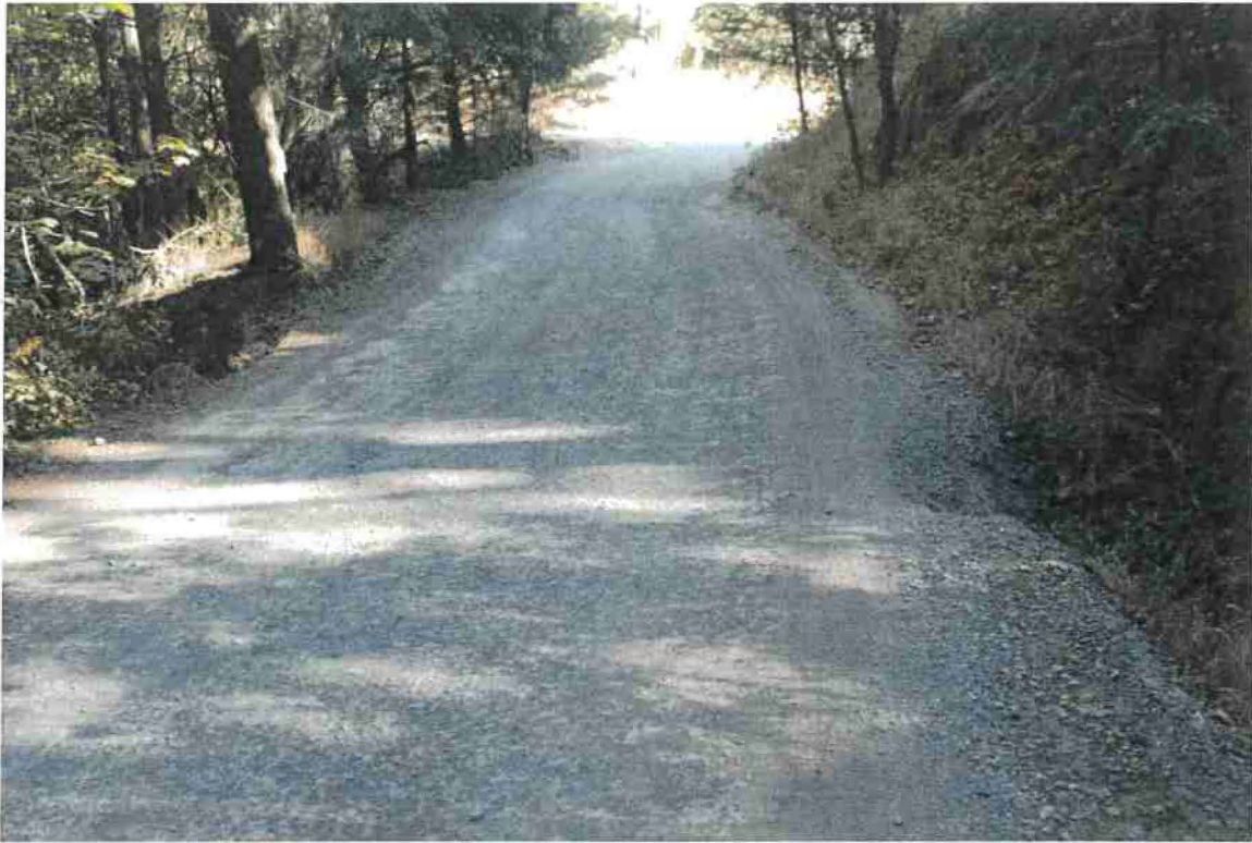
Photo 5. Mile 0.35: Pinch point at culvert; 16-ft road width with no shoulder and partial blind corner.
