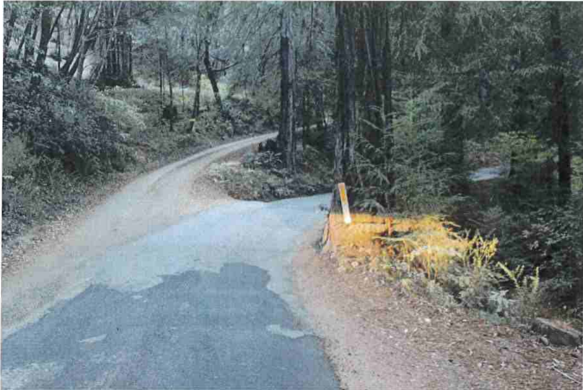
Photo 1. Mile 0.1: Pinch point at tree: 15-ft road width with 1-ft shoulders, decent visibility.
