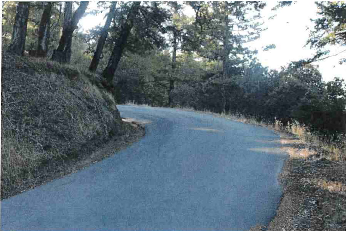
Photo 36. Mile 3.15: Dangerous pinch point at blind corner. 15-ft road width with 1-ft shoulders. Potential spot to widen corner on inside to improve width and visibility.
