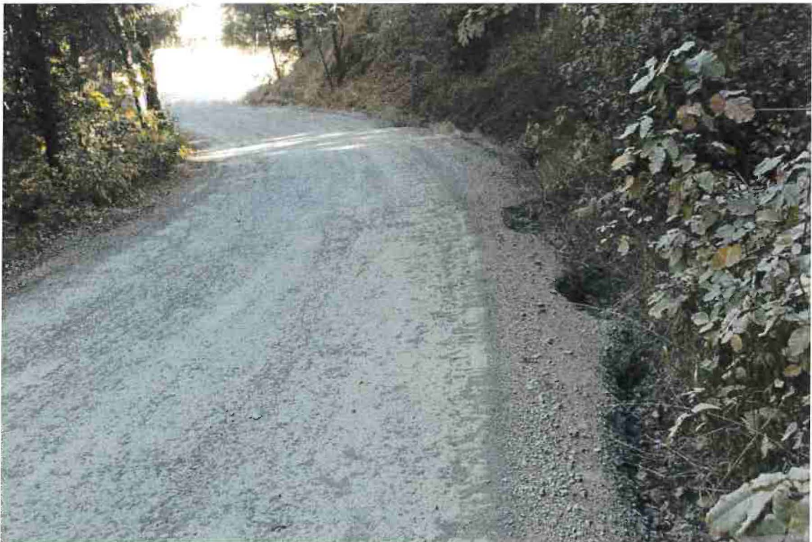
Photo 4. Mile 0.35: Inboard ditch eroding into road.
