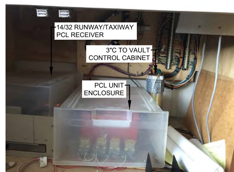
1 PCL UNIT AND RUNWAY/TAXIWAY PCL RECEIVER IN CONTROL CABINET SCALE: NTS
