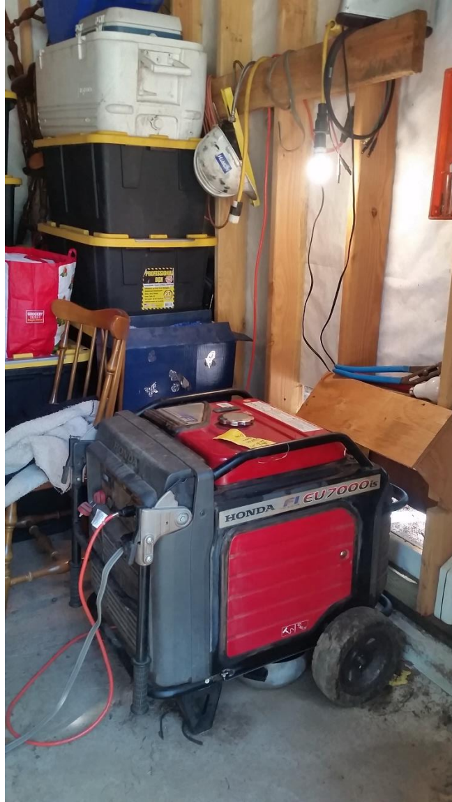
Photo 17. inside of generator shed - insulated with concrete floor
