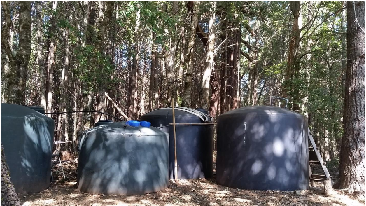
Photo 23. Tank Farm at Site D near well shed
