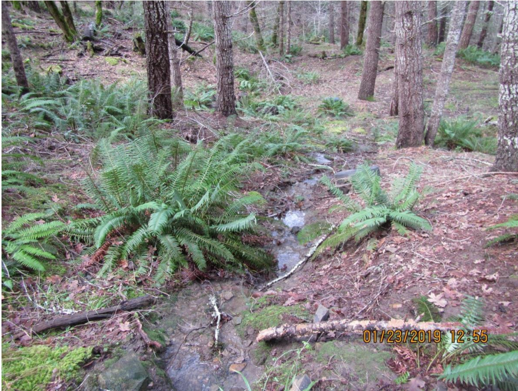
Photo 7. Looking downstream at the outboard fill where it used to cross the road
