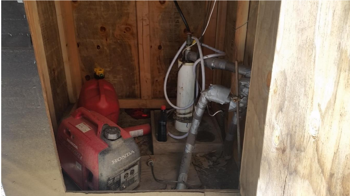
Photo 14. Generator and gas can in well shed; Site D.
