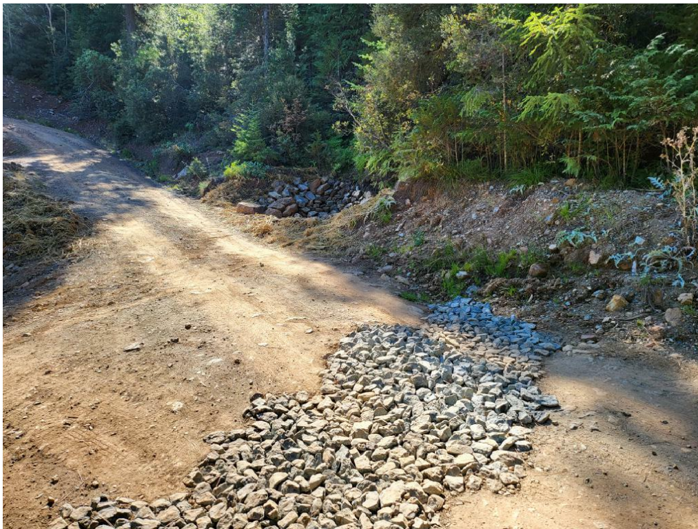
Figure 34: MP10 disconnected road surface from watercourse.
