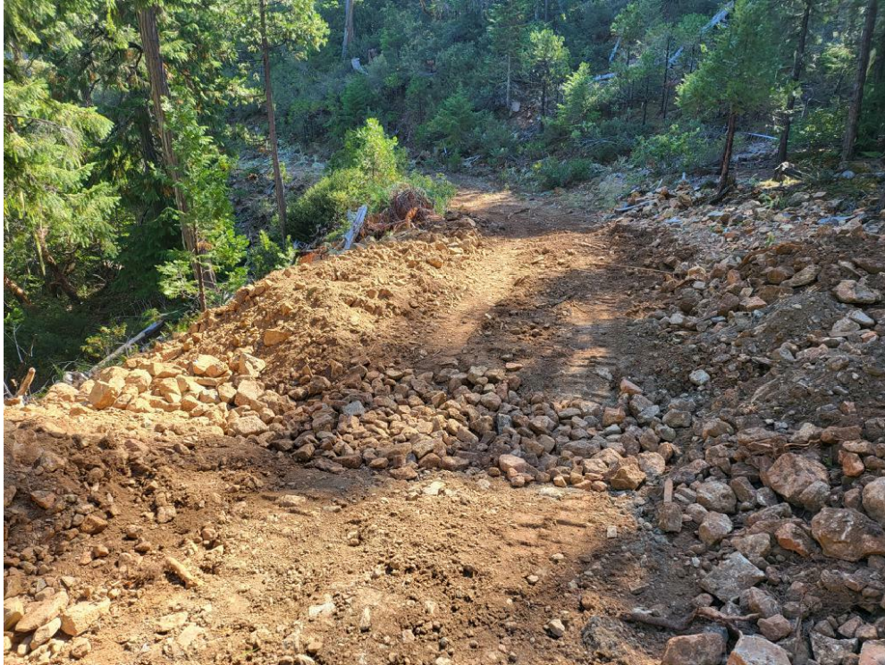
Figure 9: MP4 disconnected roadway.
