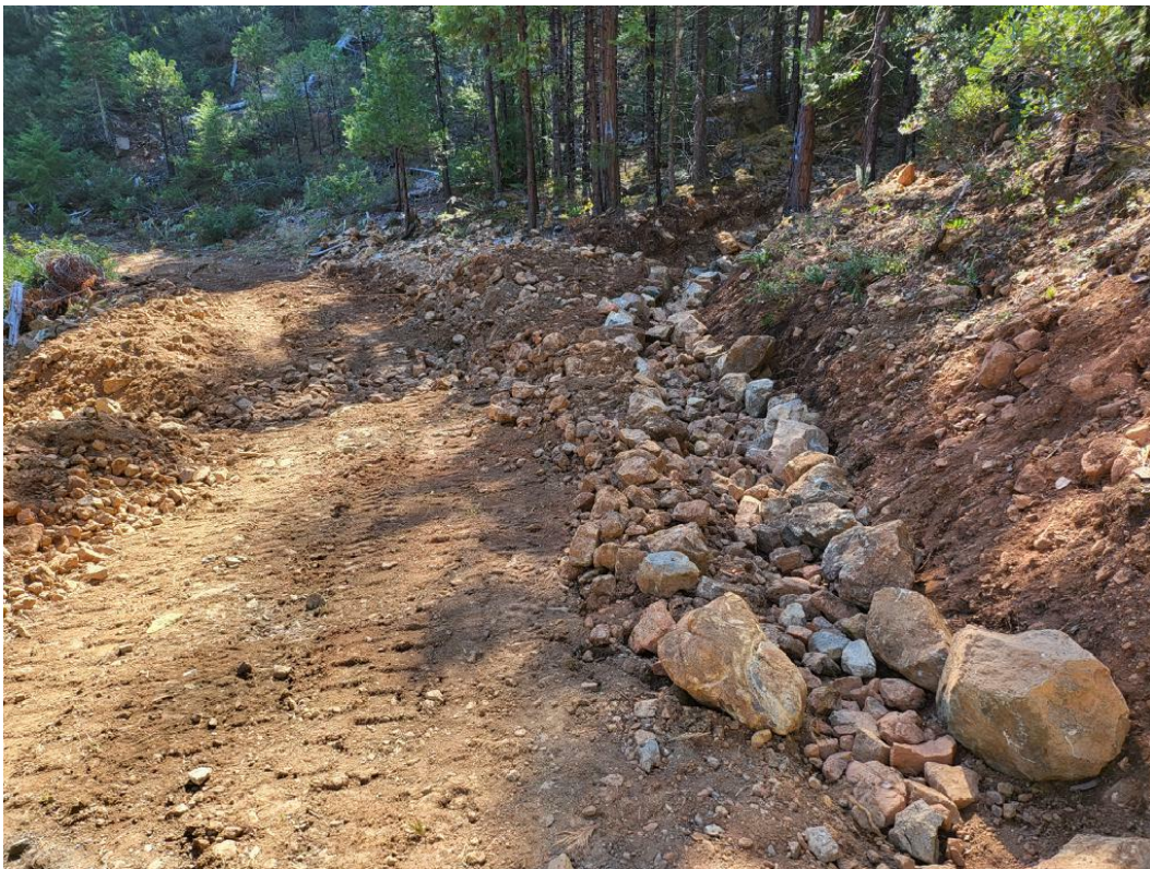
Figure 8: MP4 rocked ditch disconnecting spring from roadway.
