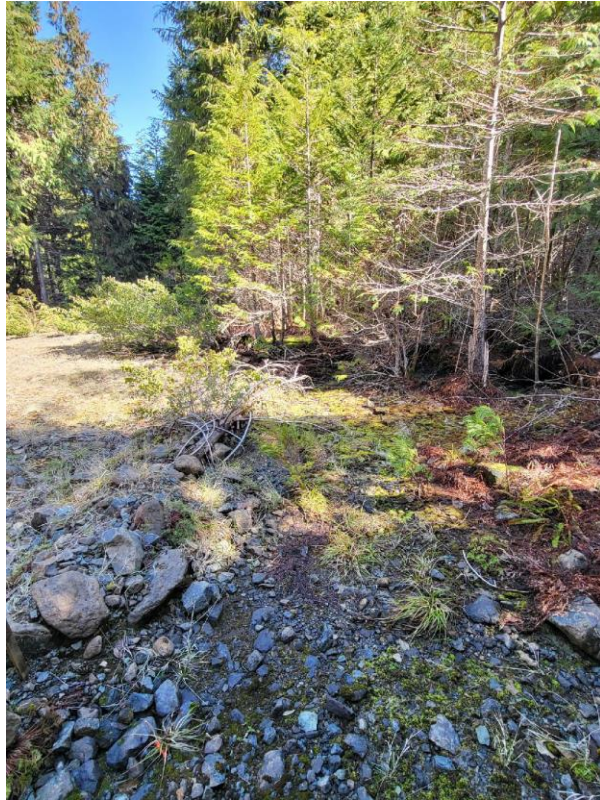
Figure 45: MP14 naturalized channel with rock.
