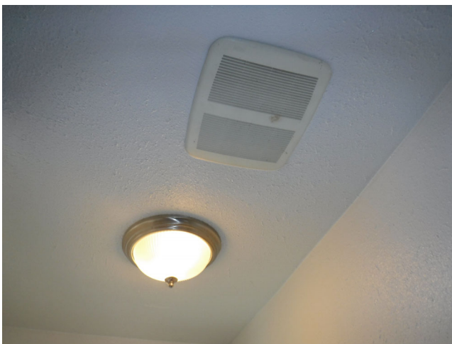
33. Bathroom ventilation and typical light fixture.
