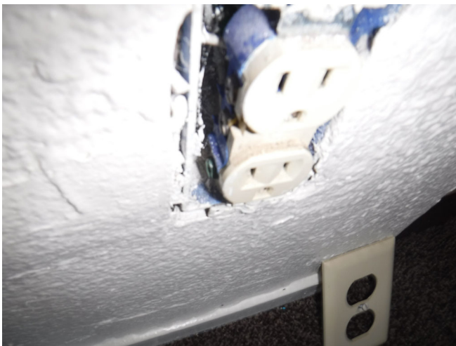
29. Copper wire observed and reported.
