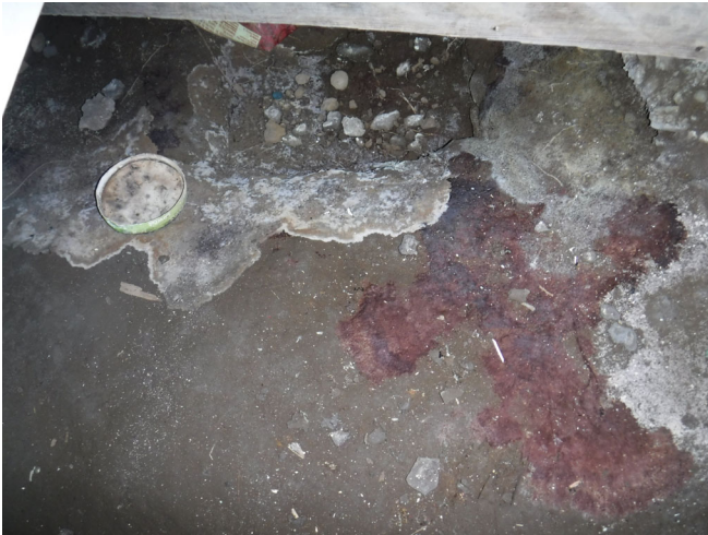
15. Debris in crawl space and mildew or mold on soil, lack of vapor barrier.
