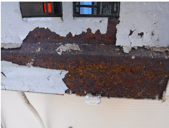
27. Rust damaged electrical subpanel at meter.
