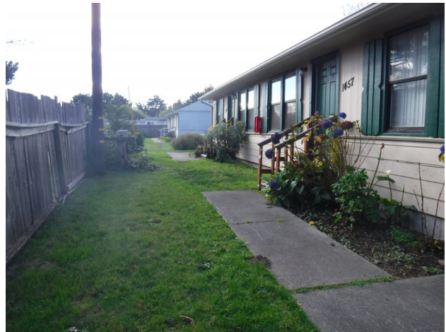
2. East perimeter of the Property, view south. Note damaged wood fencing.
