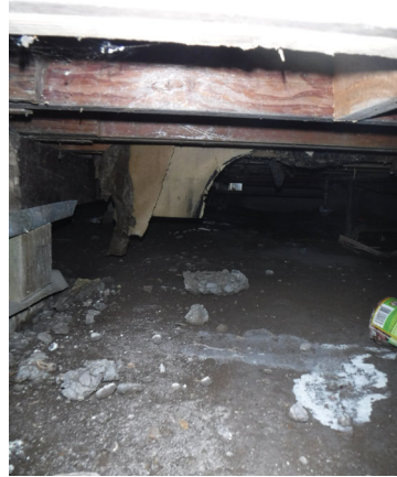
14. Typical crawl space conditions, not damaged insulation, waste, debris and moisture.
