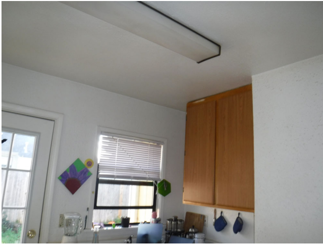
43. Florescent lighting at unit kitchen.
