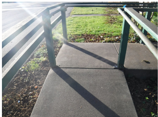
6. Non-conforming ramp at accessible unit entry.
