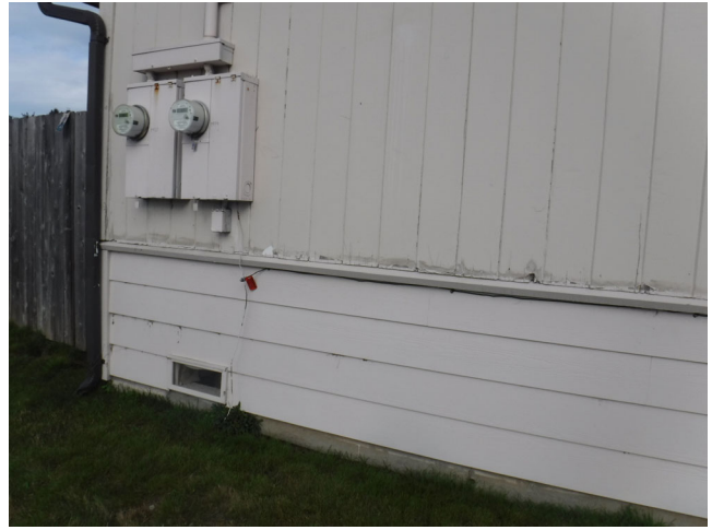
20. Damaged siding and individual electrical meters.
