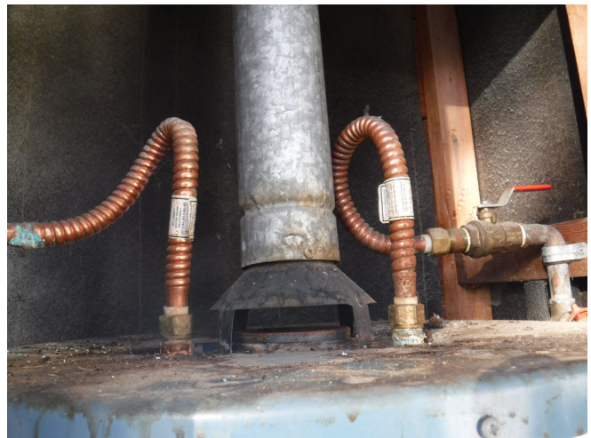
24. Copper water lines.
