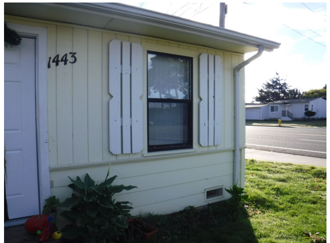
18. Building mounted signage, unit entry, single hung window, siding and downspout for roof drainage.
