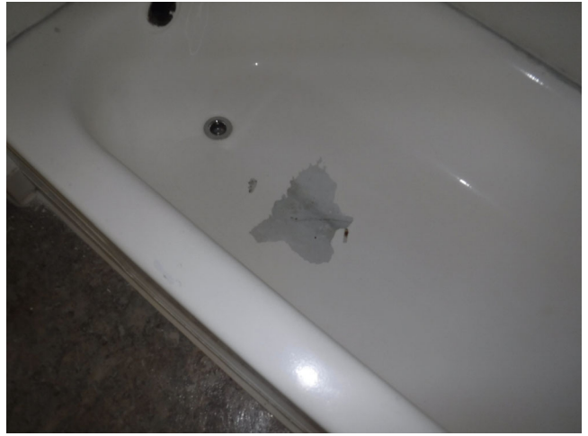
44. Peeling finish at bathroom tub.
