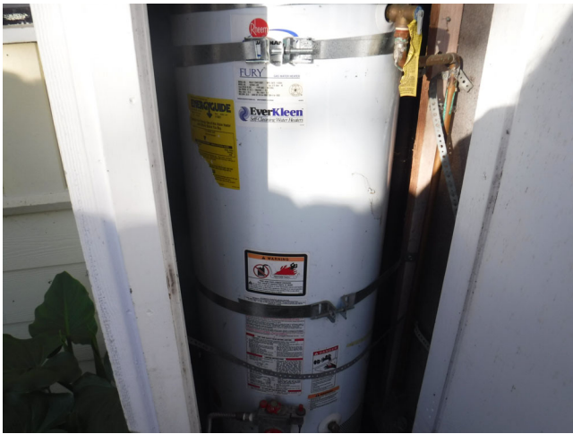
25. Typical water heater.
