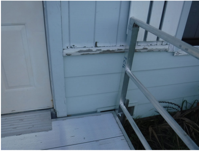
19. Peeling paint at exterior siding and trim.
