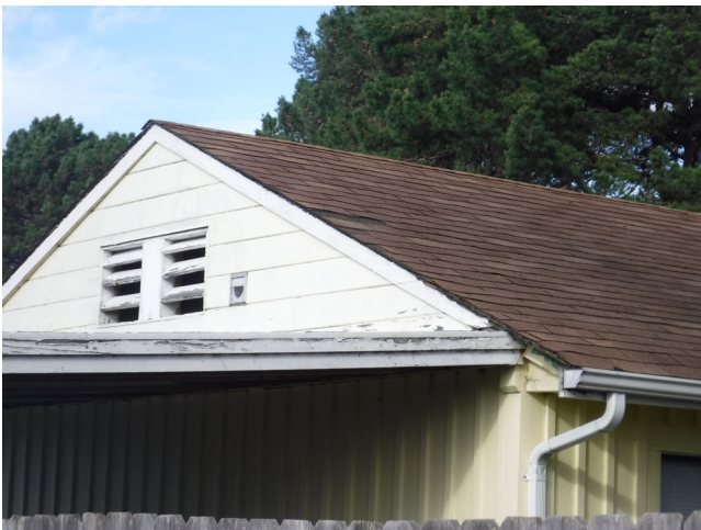
17. Worn and missing roofing, peeling paint and damaged siding.
