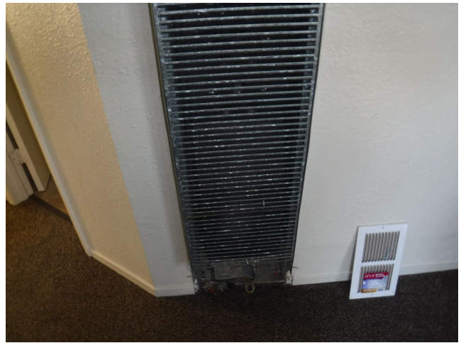
32. Typical unit heater.
