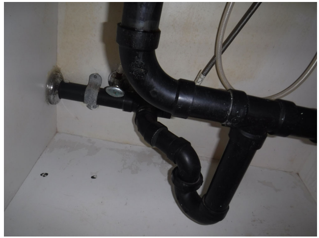
26. ABS waste line below bathroom sink.
