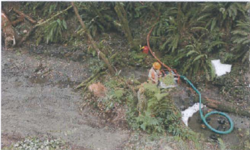
FIGURE 198. Sand bag retention dam on this small stream was used to pond streamflow so it could be pumped around a culvert installation site. The green intake hose is screened to keep out rocks and debris while the red pump hose extends several hundred feet around the project work area.
