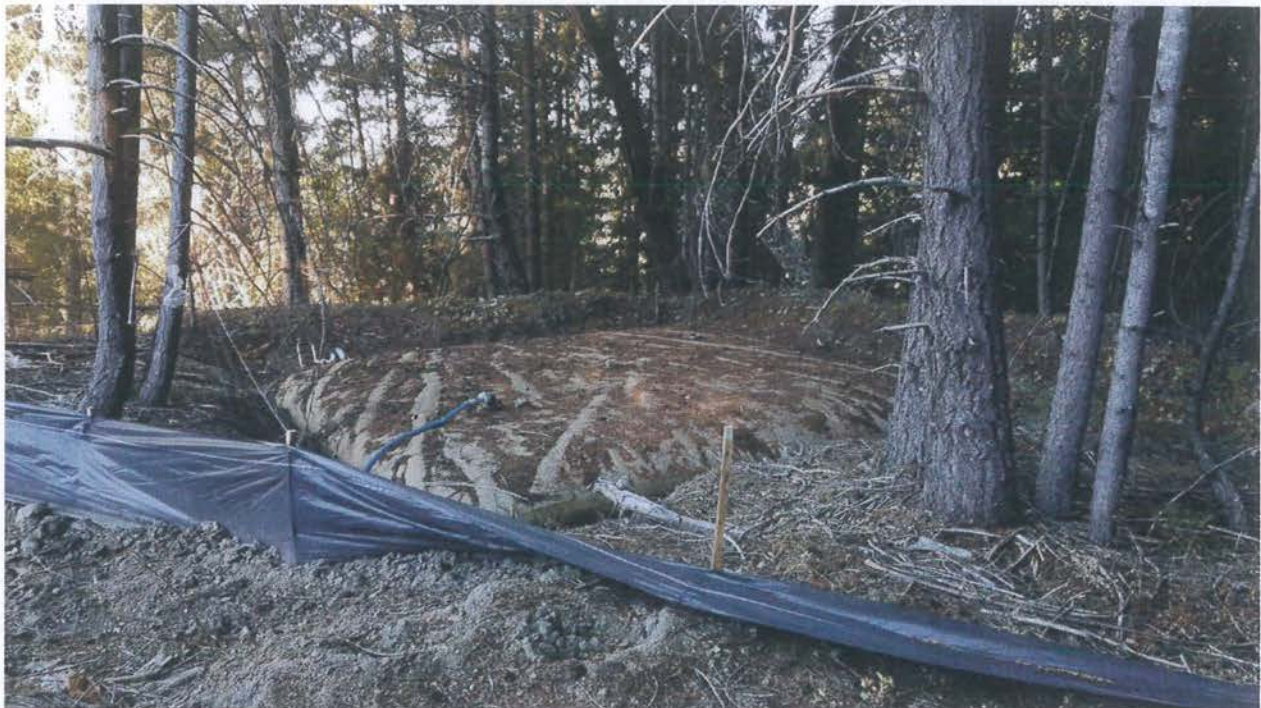
This is an example of a containment pit which will assist in mitigating the impacts if this storage bladder failed.
