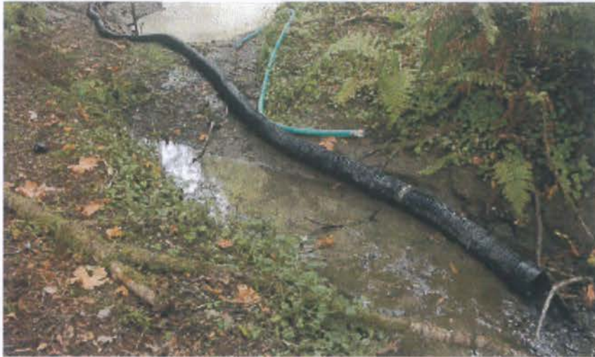
FIGURE 197. Flex pipe stream diversion around a road construction site. The inlet to this 8 inch diameter flex pipe inlet collects clear streamflow from a retention dam above the project site and gravity feeds it around the project area and back into the natural channel downstream from construction work (see photo).
