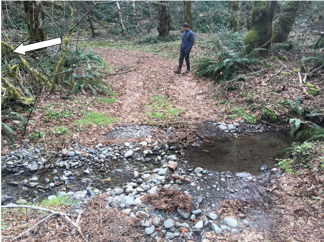
Photo 7. Ford crossing – Looking road-right. White arrow indicates location of recommended berm relief.
