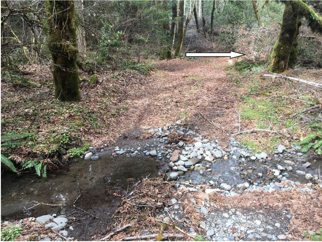
Photo 6. Ford crossing – looking road-left. White arrow indicates location of recommended berm relief.
