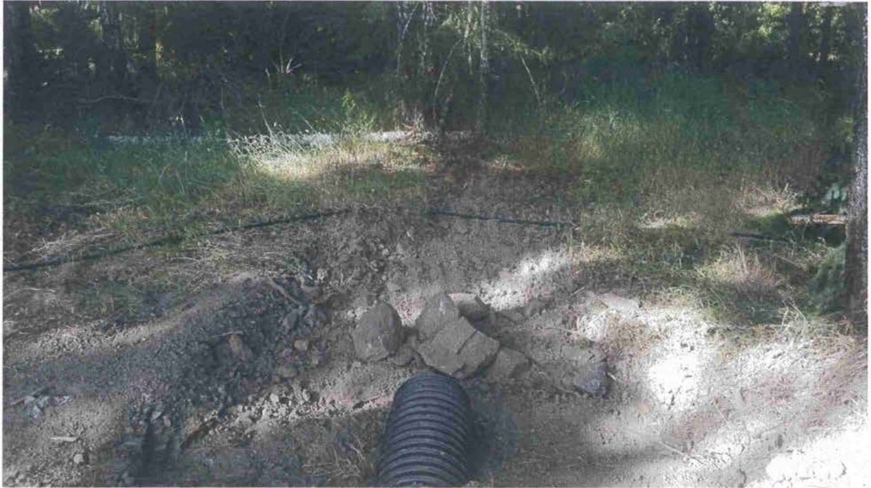
Picture 8: This is the overflow spillway outlet for the rain catchment pond. Photo date 7-06-2017.
