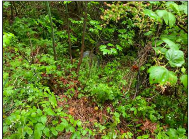
Photo #64 Private Access Looking @ Clogged Culvert Out (Size Unknown)
