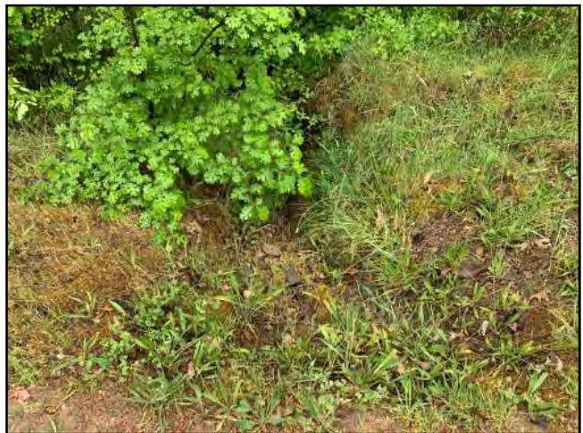
Photo #166 Private Access Rd Looking @ Clogged Culvert out (size Unknown)
