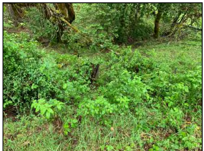
Photo #180 Private Access Rd Looking @ Clogged Culvert Out (Size Unknown)
