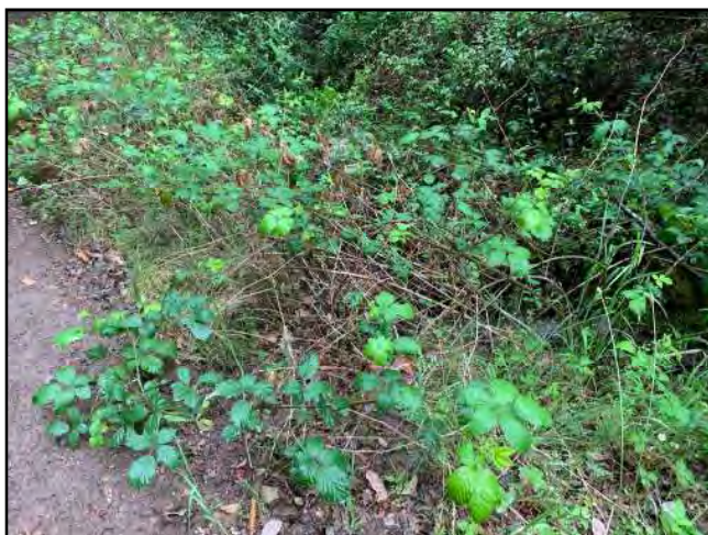
Photo #209 Stewart Ranch Rd Looking @ Clogged Culvert Out (Size Unknown)
