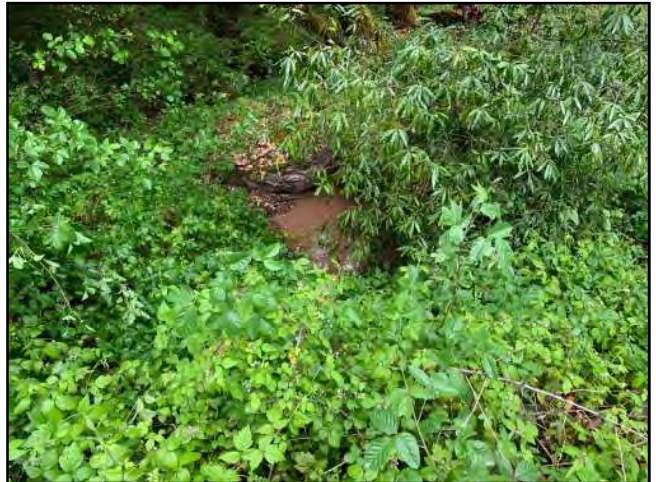
Photo #172 Private Access Rd Looking @ Partially Clogged 12" Culvert In
