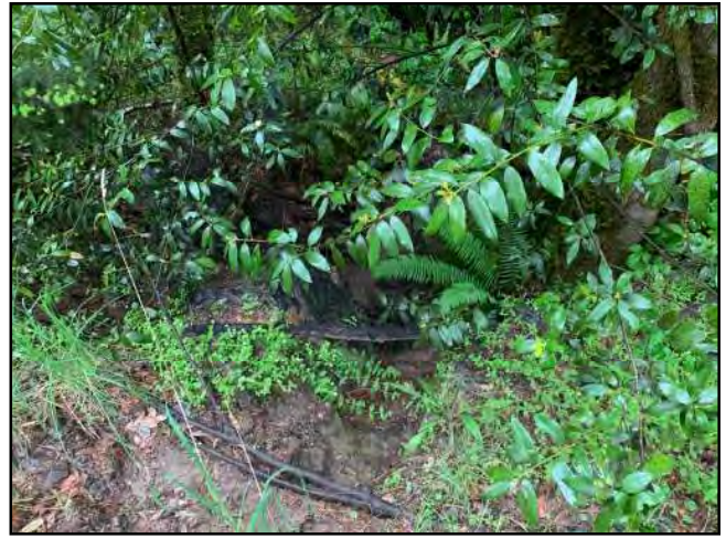
Photo #14 Private Access Rd APN 216-202-009 Looking @ Clogged Culvert Out (Size Unknown)
