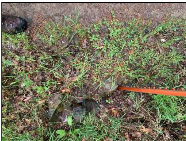
Photo #179 Private Access Rd Looking @ Clogged Culvert In (Size Unknown)
