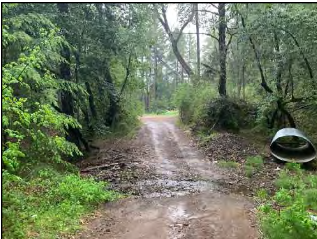
Photo #21 Private Access Rd APN 216-202-009 Looking North @ Area Needing Rock Ford
