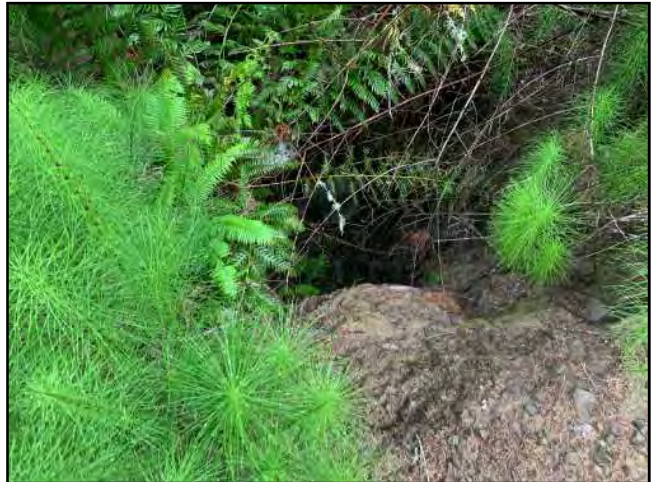
Photo #88 Private Access Looking @ Partially Clogged 24" Culvert Out
