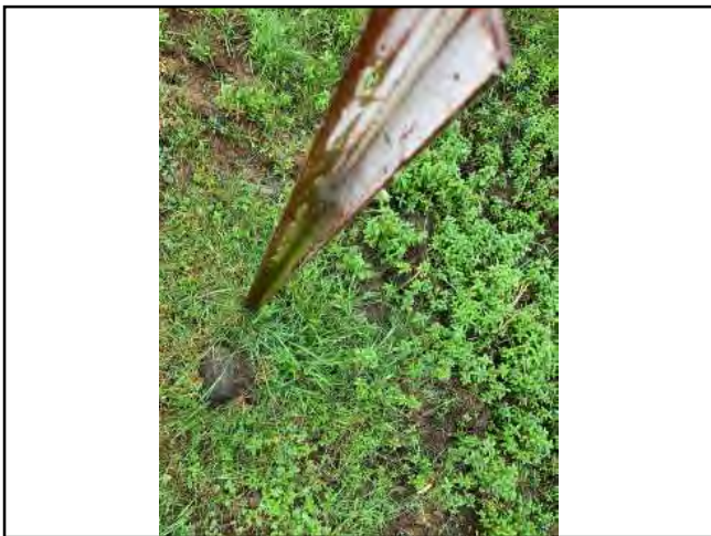
Photo #165 Private Access Rd Looking @ Clogged Culvert In (size Unknown)
