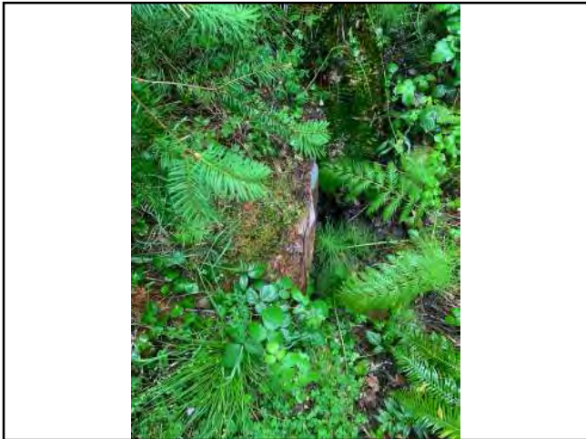
Photo #87 Private Access Looking @ PARTIALLY Clogged 24" Culvert Out
