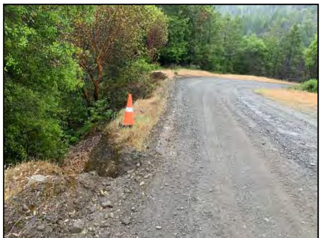
Photo #234 Stewart Ranch Rd Looking SW @ Erosion
