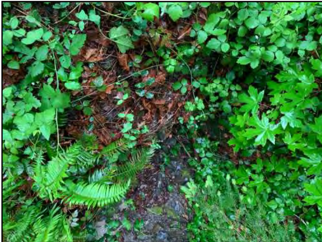
Photo #63 Private Access Looking @ Clogged Culvert In (Size Unknown)
