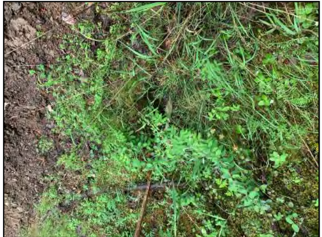
Photo #208 Stewart Ranch Rd Looking @ Clogged Culvert In (Size Unknown)
