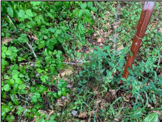
Photo #129 Private Access Rd Looking @ Clogged Culvert In (Size Unknown)
