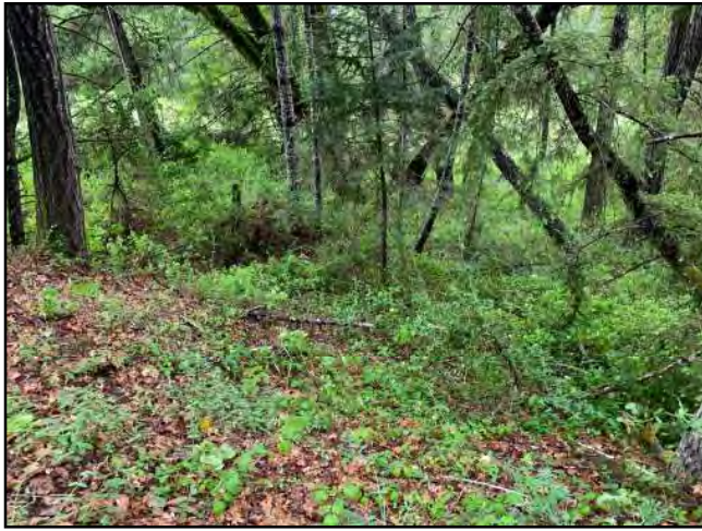
Photo #157 Private Access Rd Looking @ Partially Clogged Culvert In (size Unknown)
