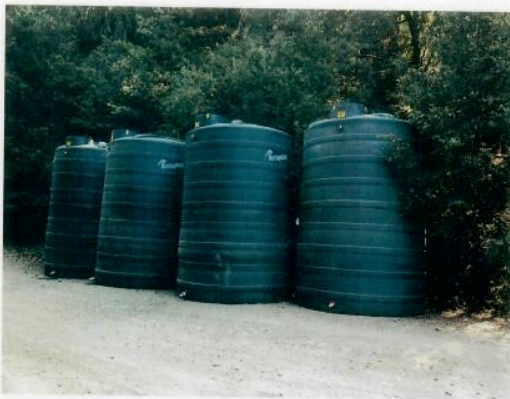
Four 5,000-gallon plastic tanks recently added to the property, which were not part of the original notification.
