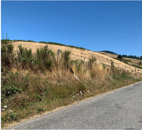
Sign post in ditch
