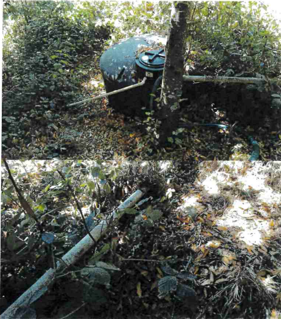
Pictures 6 & 7: These are photographs of the domestic POD #3. This diversion consists of a 3 inch PVC buried into the hillside. The diversion diverts to this 550 gallon storage tank. The rate of diversion is approximately 2 gallons per minute. Photo date: 09/13/2016
