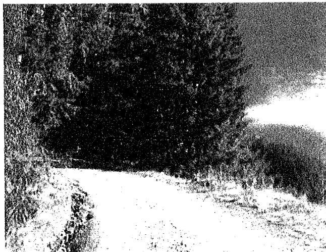
Figure RP 5. Photograph showing erosion on the inboard ditch of Roadway 3 (Private Access Road) from approximately 350 ft. up gradient from its start. A rolling dip needs to be installed approximately
