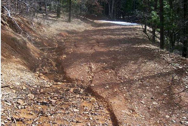
Figure 19. Erosion caused by ditch water leaving the ditch and traveling across the road. Photo: Susan Kocher.
