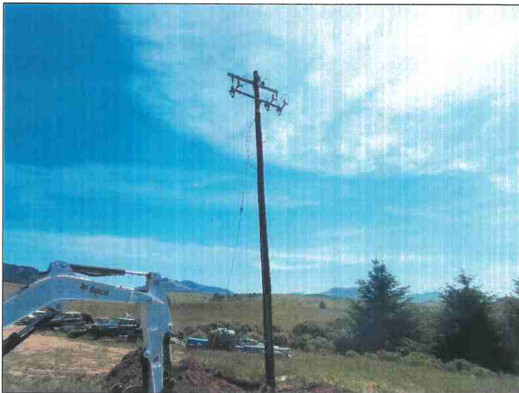
Figure 4. The new PG&E power drop.
