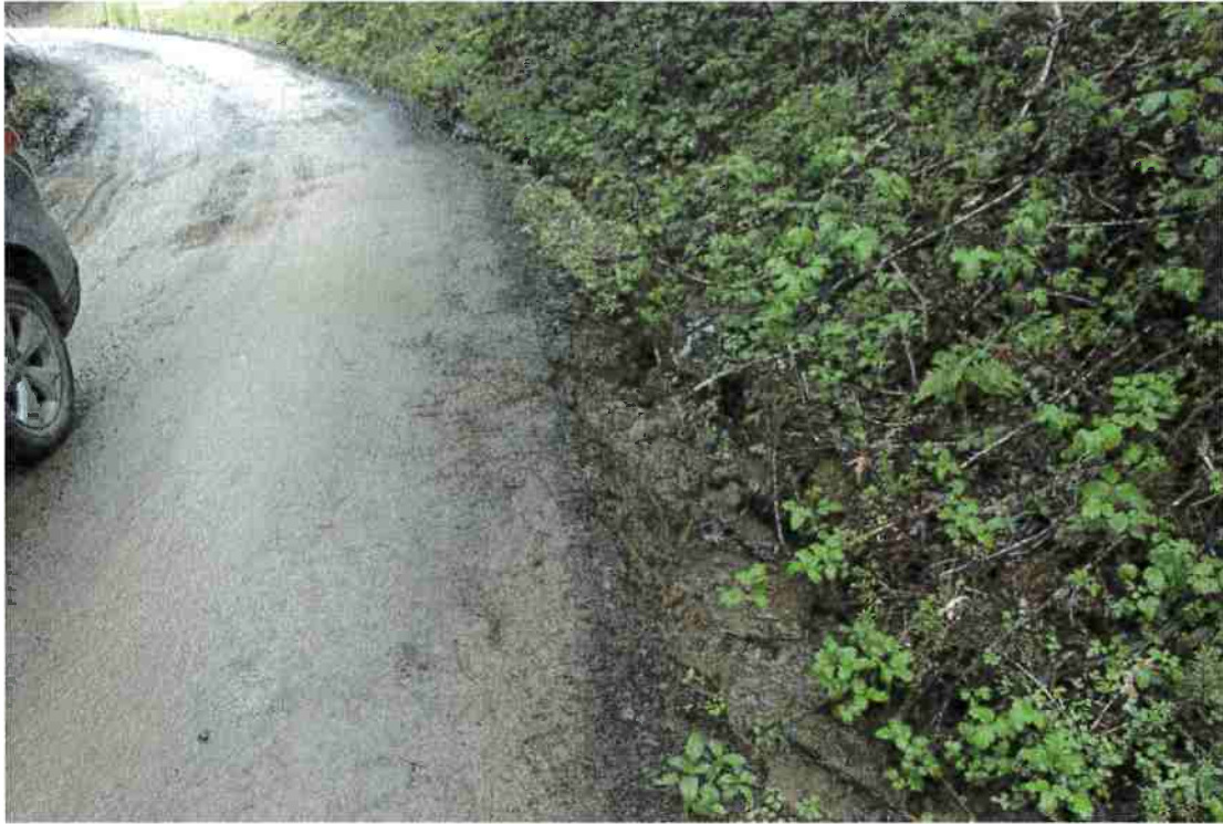
Photo 15. Mile 6.7: Inboard ditch erosion, new culvert at natural swale proposed to eliminate problem.
