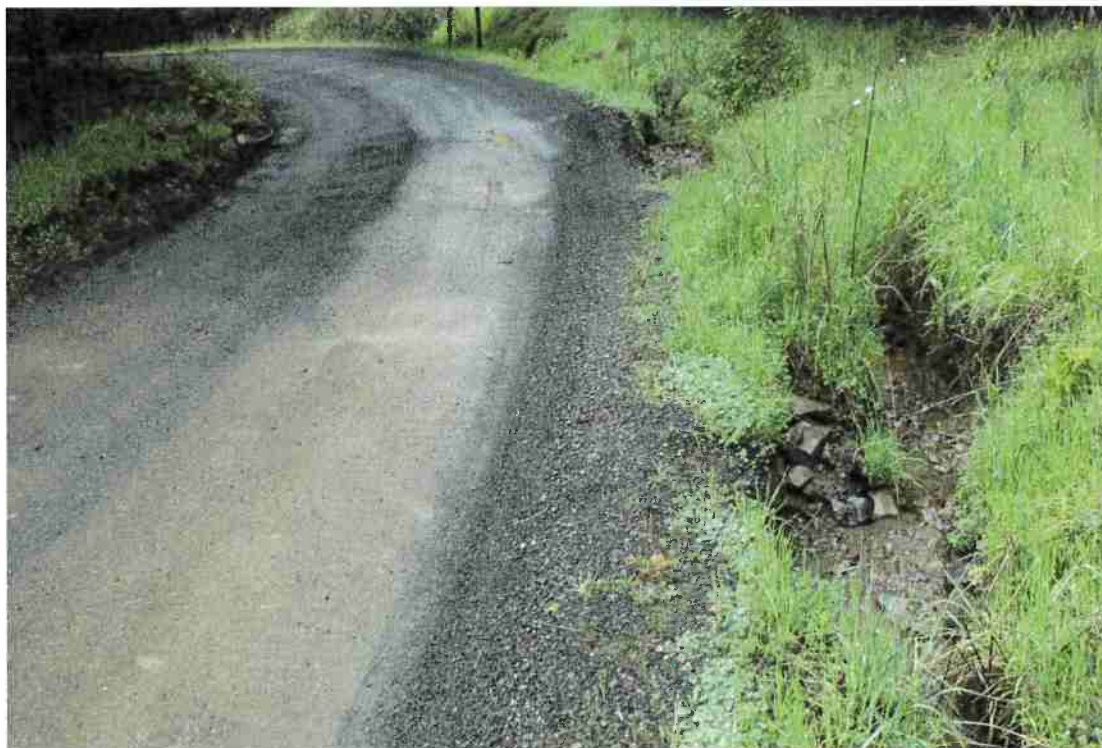
Photo 8. Mile 6.3: 16-ft road width with 1-ft shoulder, Inboard ditch erosion, new culvert at natural swale proposed to eliminate problem.
