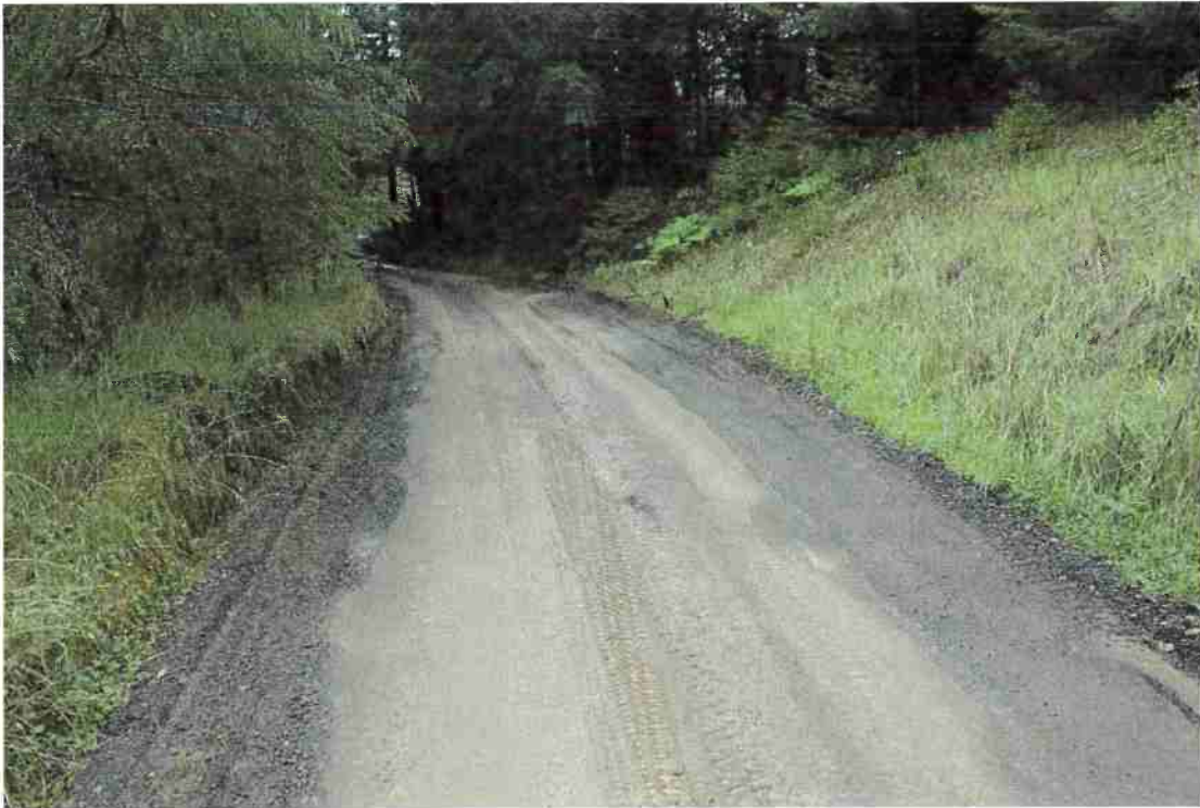
Photo 17. Mile 6.8: 12-ft road width with no shoulder.
