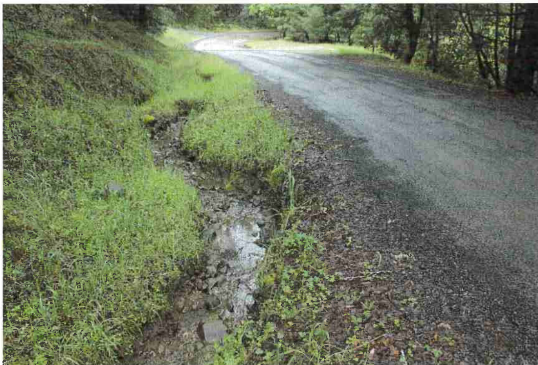
Photo 5. Mile 6.2: Inboard ditch erosion, new culvert at natural swale proposed to eliminate problem.
