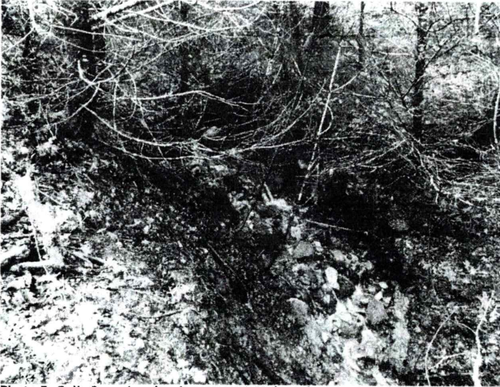
Photo 5. Gully 2 erosion showing segment at downslope extent of failed pond berm.
